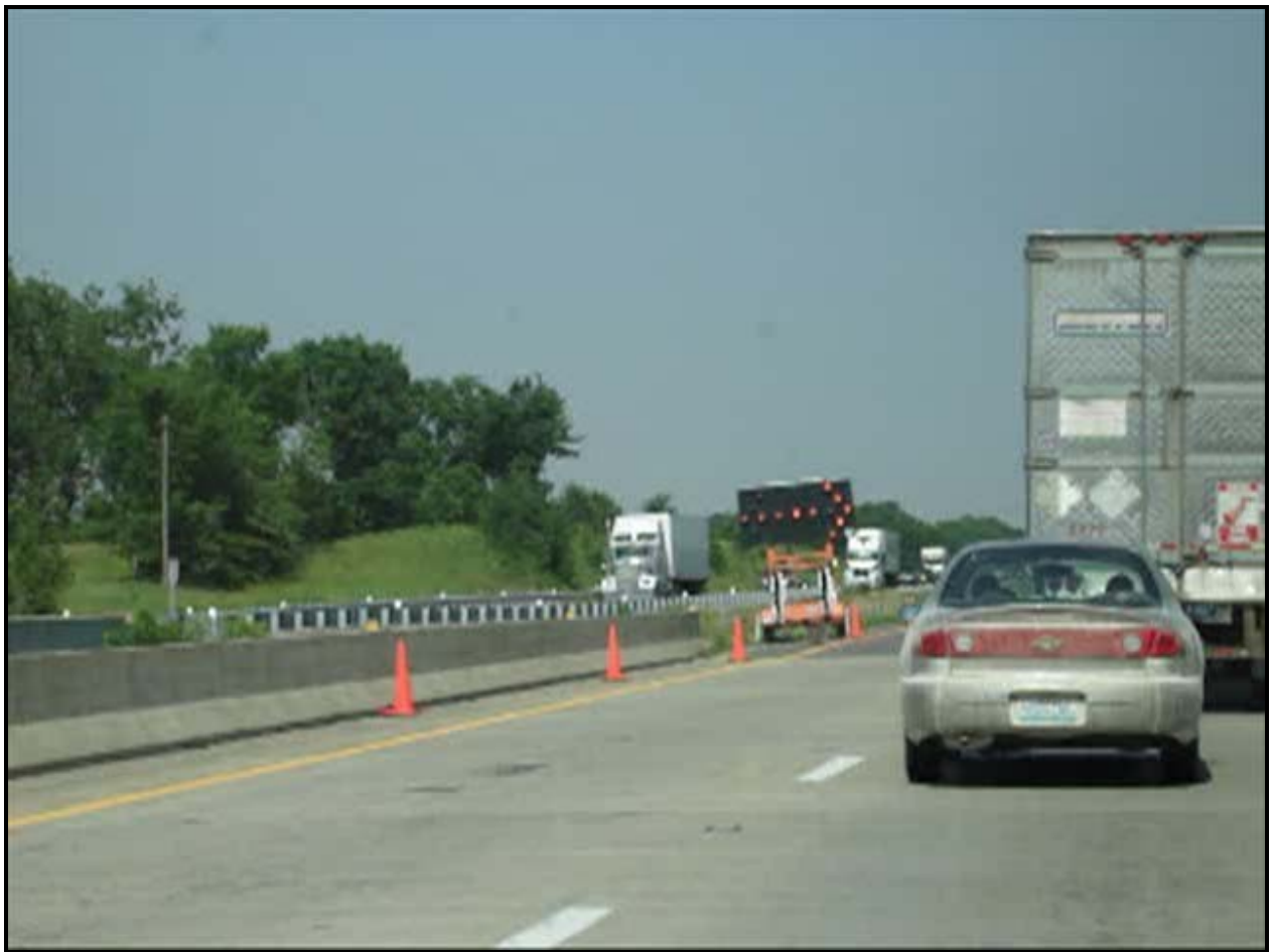
FIGURE 1 Typical advance warning arrow display at a long-term work zone (flashing arrow displayed).
