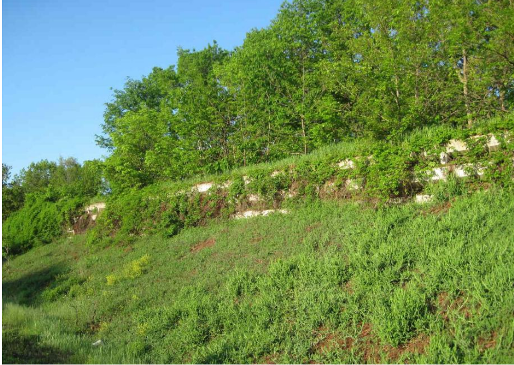
Figure 4.1: Front View of the Manchester Green Noise Barrier (Courtesy of the NHDOT)
