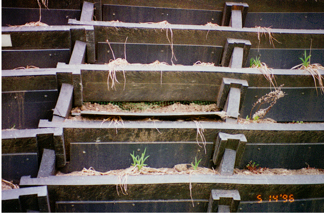
Figure 4.8: Excessive Deformation in the Horizontal and Vertical Supports (14)
