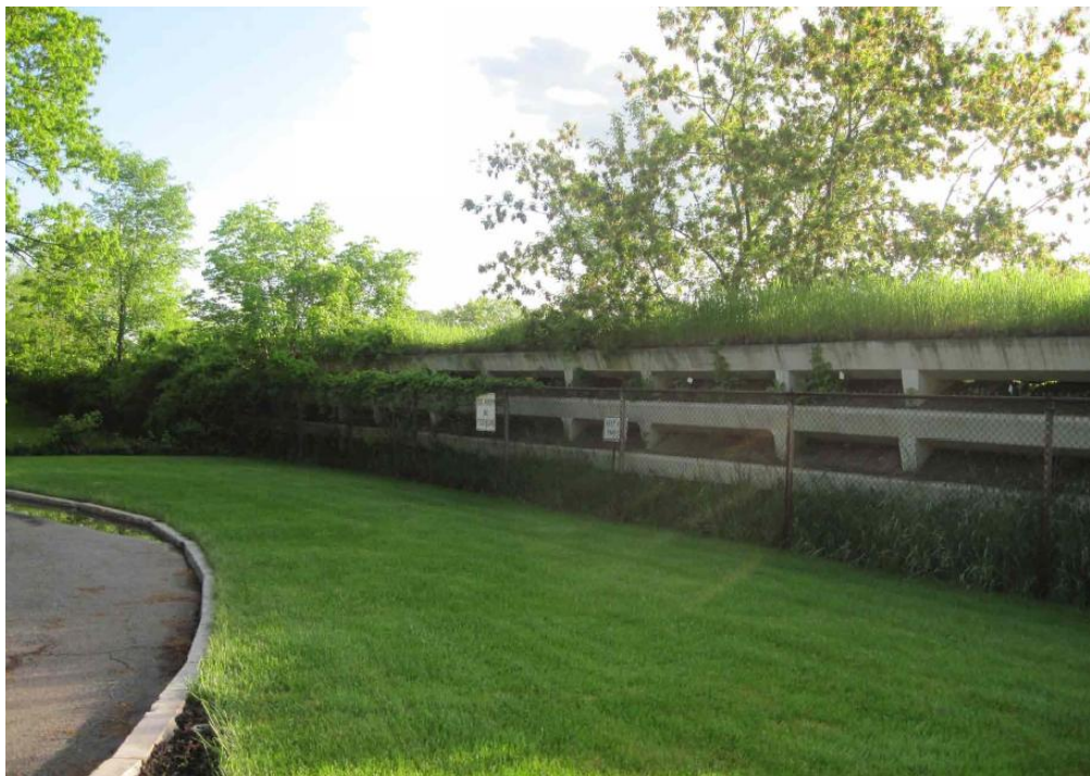
Figure 4.2: Back View of the Manchester Green Noise Barrier, A Small Hole in the Wall Can Be Noticed in the Right Side of the Picture (Courtesy of the NHDOT)
