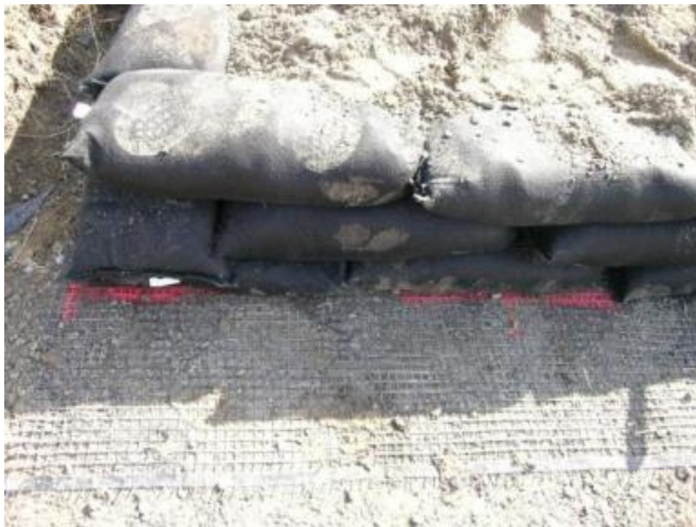
Figure 5.9: First Layer of Geogrid and Two Rows of Deltalok Bags Containing Gravel
