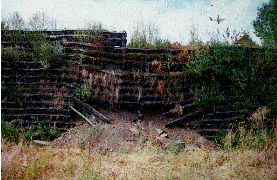
Figure 4.10 Collapse of the Wisconsin Recywail (14)
