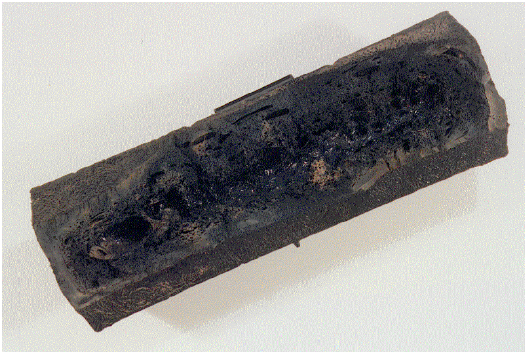
Figure 4.9: Large Air Voids in Plastic Connections Due to Factory Defects (14)
