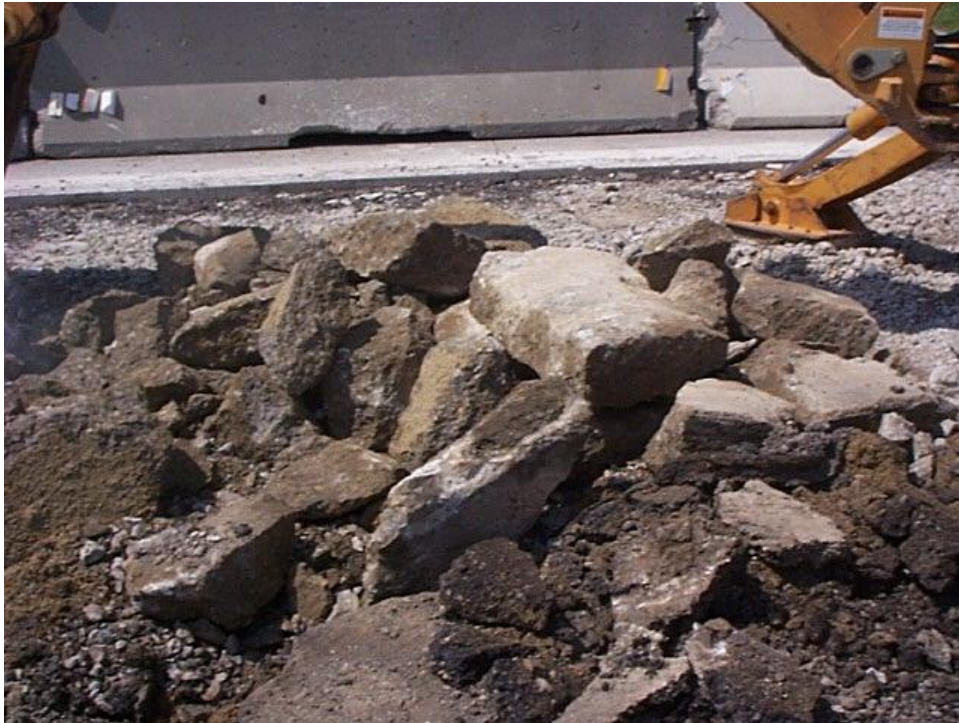
Figure 6. Large Uncracked Pieces at the Bottom of Concrete Pavement
