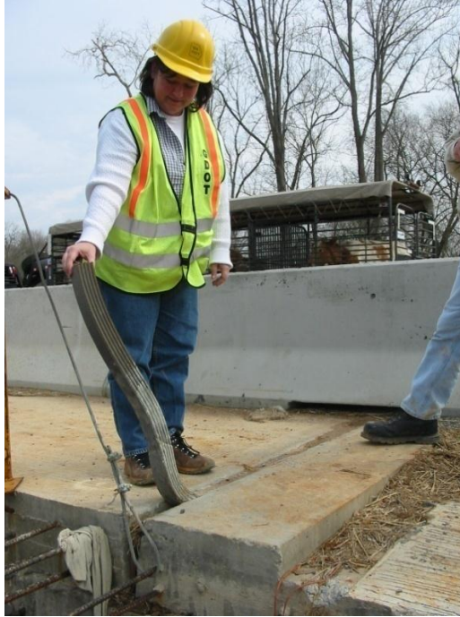
Figure 3.2.2.1 – Ms. Harper holding an Evazote expansion joint being installed (bridge supporting GA SR 113 at Etawah River)
