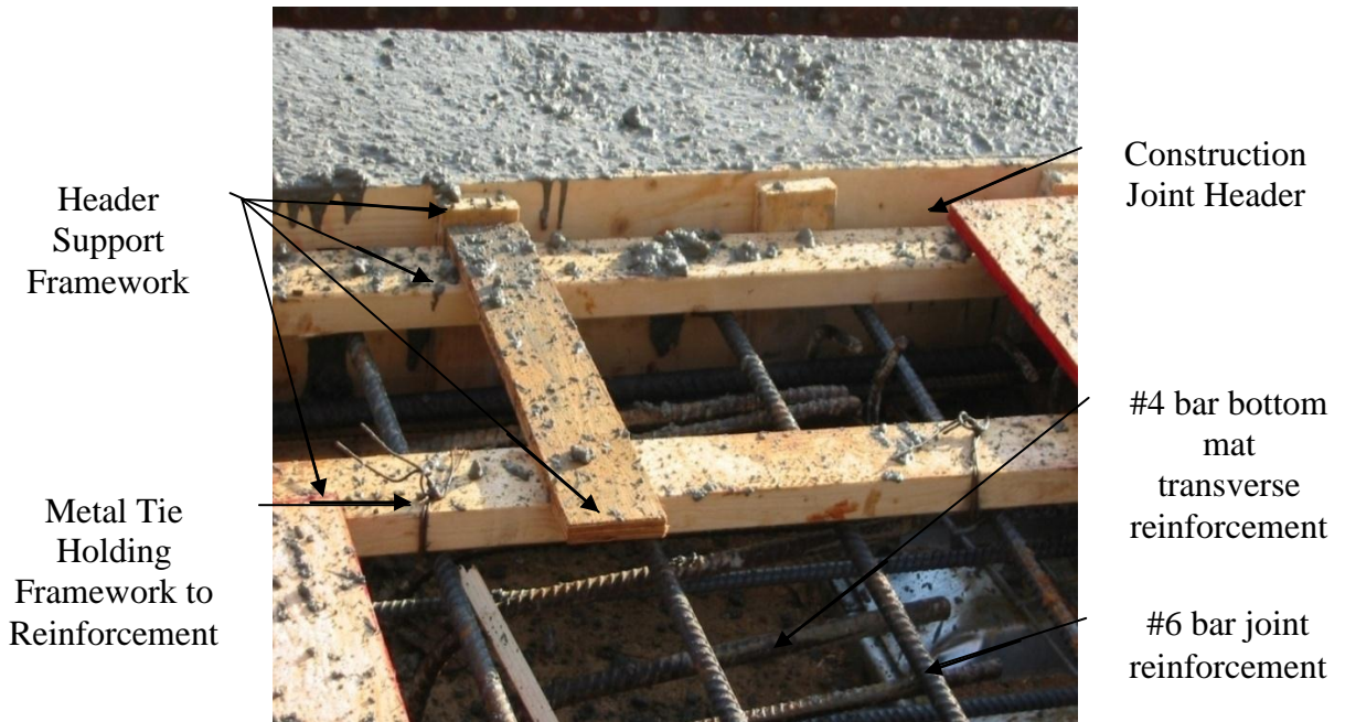
Figure 3.2.1.2 – Header construction layout for #6 bars in continuous deck detail (bridge supporting GA SR 113 at Etawah River)
