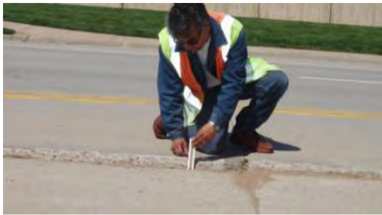
Figure 2. A faulted longitudinal joint.
