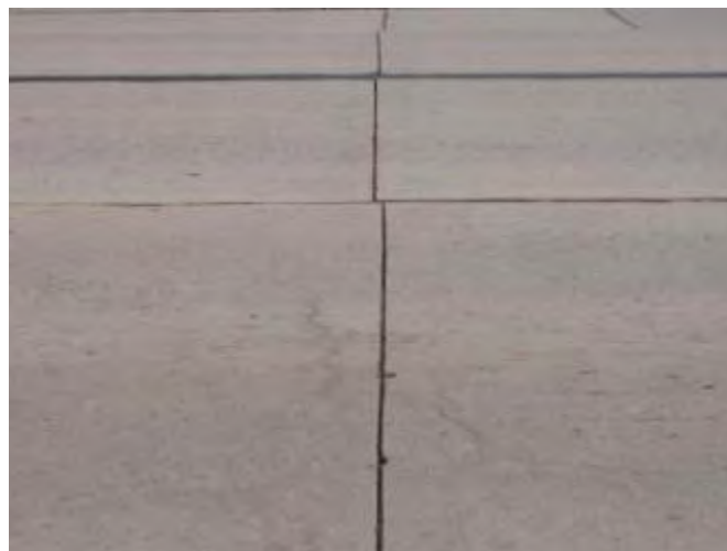
Figure 3. Slippage between lanes as evidenced by misaligned transverse joints in adjacent lanes.
