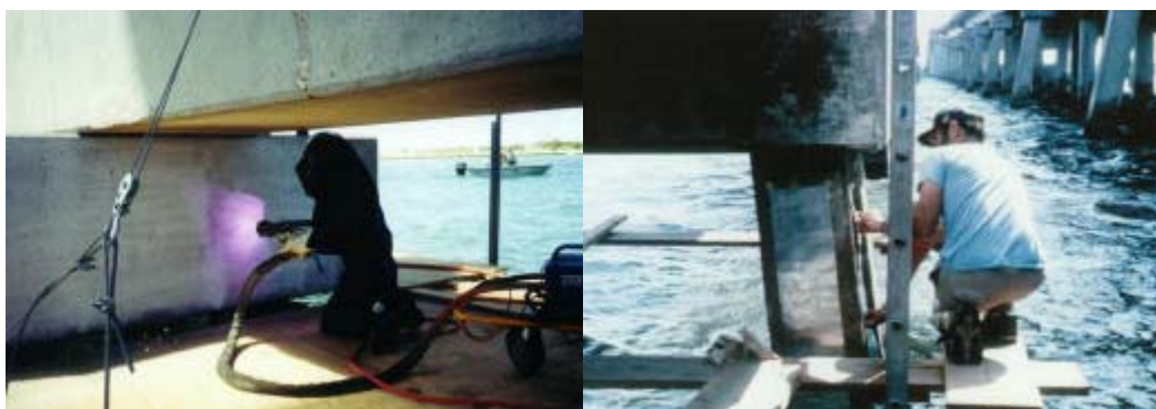
Figure 2.2: Arc spray application of galvanic Al-Zn-In to a bridge pier in Texas (left); and application of zinc/hydrogel anode to a bridge pier in Florida (right) (Daily 1999).
