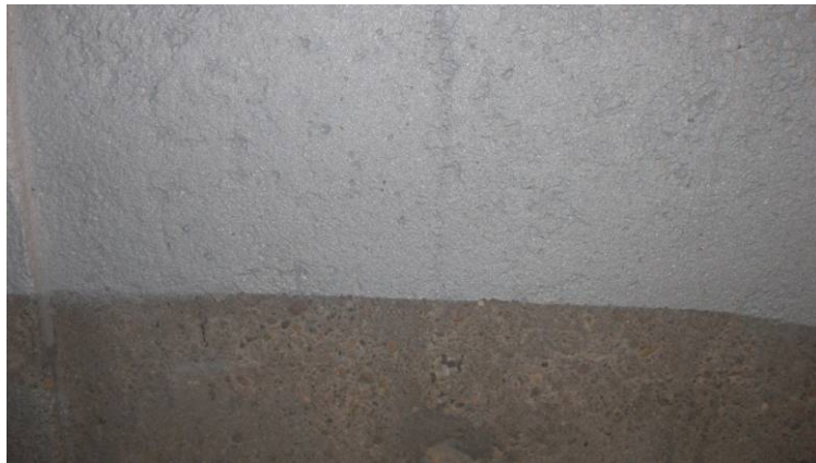
Figure 4.36: Irregular concrete surface due to paste loss.
