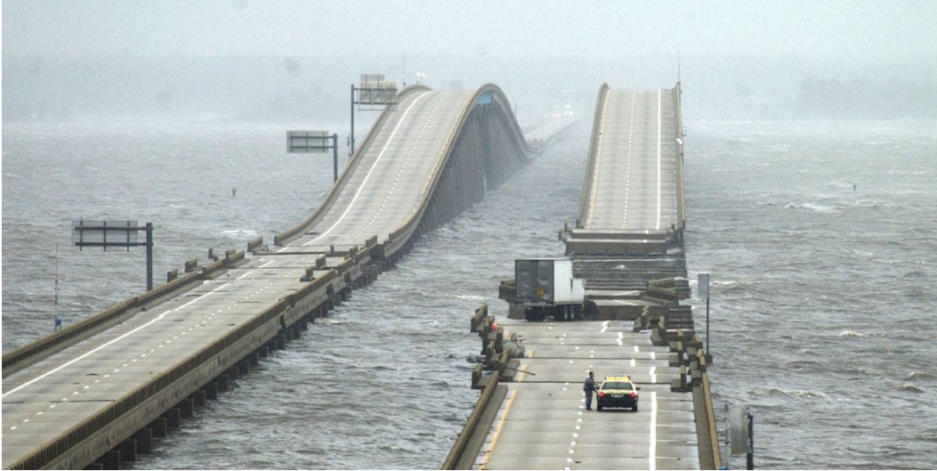
Figure 1.3. I-10 Bridge over Escambia Bay, FL, during Hurricane Ivan. (Source: Pensacola News Journal)
