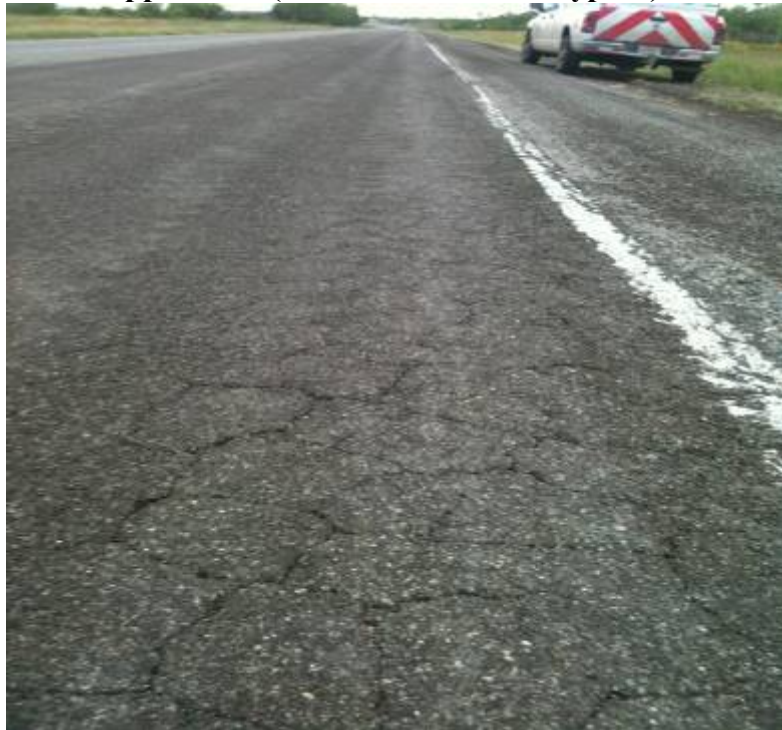
Figure 3.10. Alligator Cracking Reappeared Two Days after Placement of LRA Level-up.
