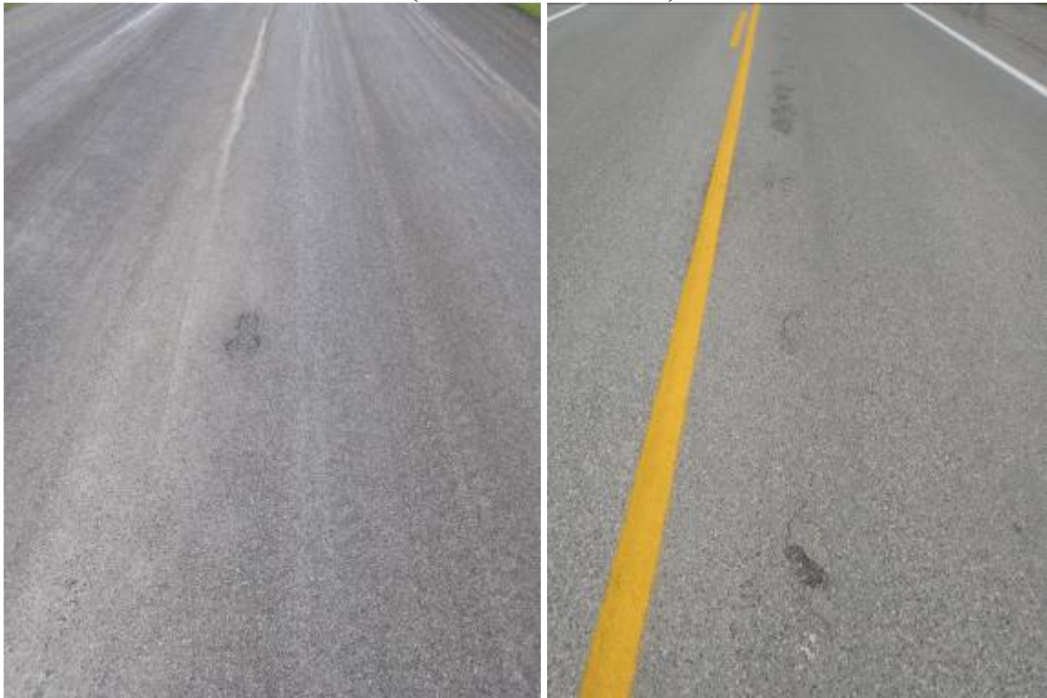
(b) Close up of Pothole (2 days After Rain) (c) Patched Potholes 3 months later. Figure 3.8. Jefferson Test Section Developed Pothole in Wheelpath in Area Holding Water (After a Rain in First Week).
