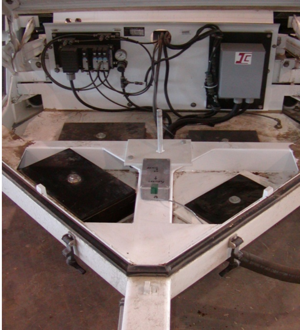
Figure 42. Accelerometer Unit Mounted on TTI E274 System.
