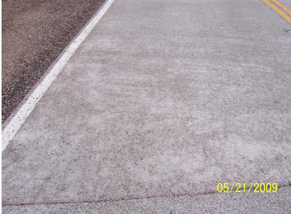
Figure 67. Surface sealed on Panel 4 by wet mixture or over compaction
