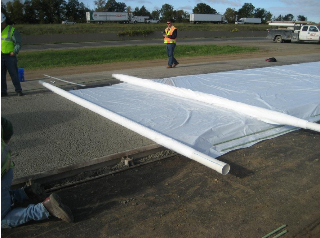
Figure 60. Completed surface of pervious overlay and covering with two layers of plastic
