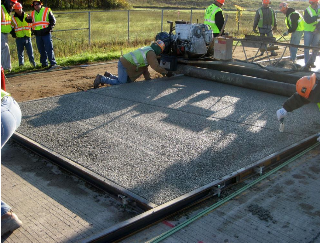
Figure 71. Observation of stretch marking on fresh pavement
