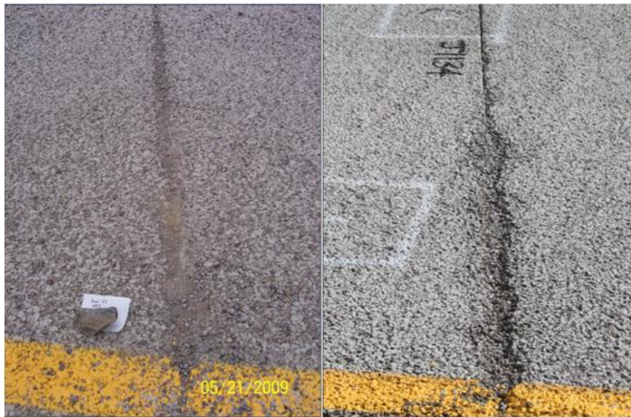
Figure 65. High severity level joint deterioration
