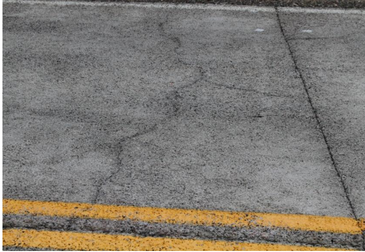
Figure 69. Transverse cracking on Panel 3
