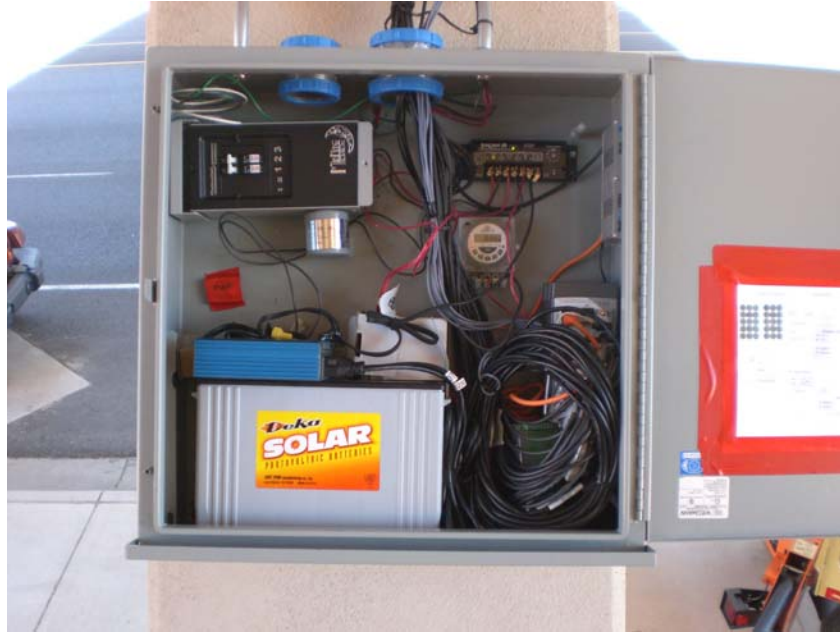
FIGURE 18 Data Acquisition System, Rechargeable Batteries, Power Inverter, Digital Timer Switch and the Wireless Modem Located at the Steel Box.
