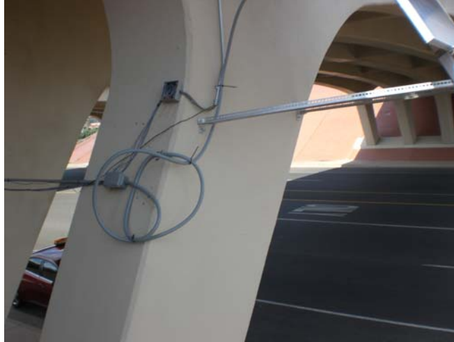
FIGURE 11 Electrical Boxes and Conduits to Pass Power to the SDAQ Using the Solar Panels.
