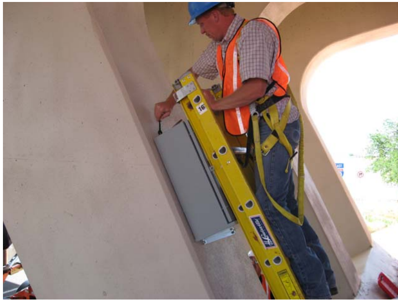
FIGURE 6 Installing of the Steel Box to House All Electrical Components at the Bottom of Bridge 7937.
