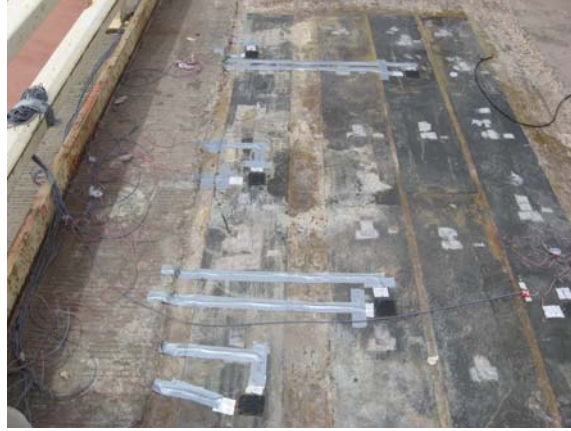
FIGURE 14 All the Strain Gauges After Being Installed on the FRP Sheets and Connected to the Wires Transmitting the Strain Signals to the Data Acquisition (DAQ) Device.
