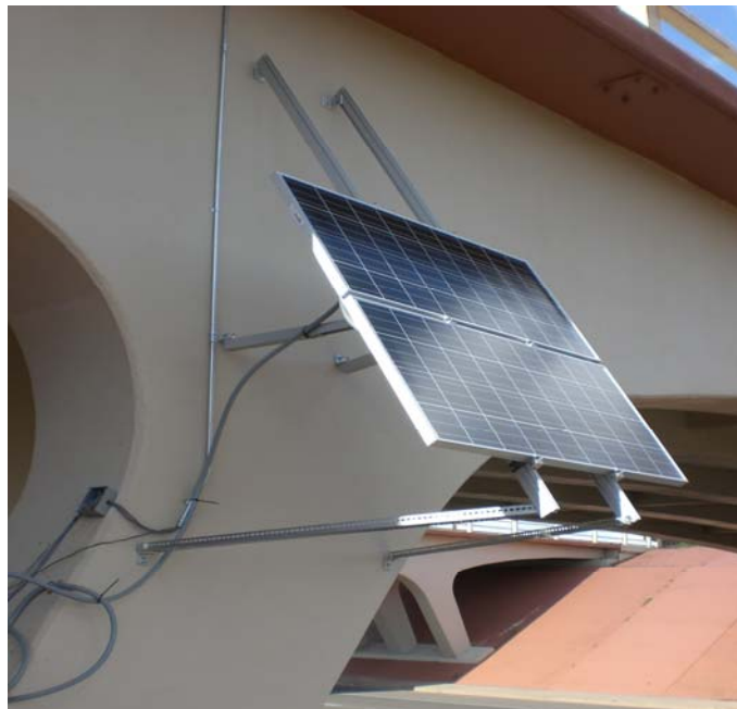
FIGURE 20 Solar Power System Installed on Bridge 7937 to Provide Clean Renewable Energy for The SHM System.
