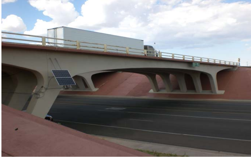
FIGURE 19 Solar Power System Installed on Bridge 7937 to Provide Clean Renewable Energy for The SHM System.
