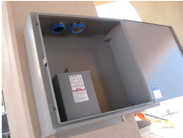
FIGURE 7 Steel Box Used for Housing the Data Acquisition System and All SHM Components.
