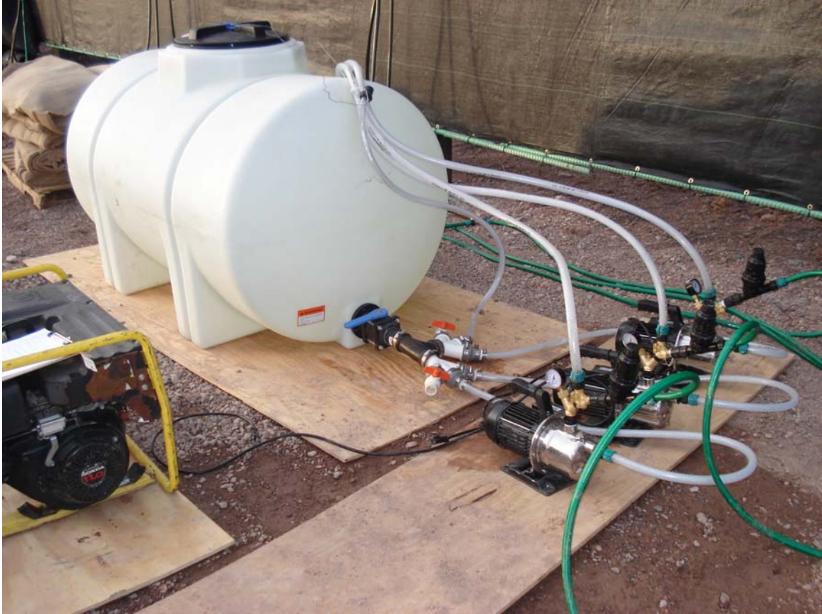
FIGURE 8 Water tank, water pumps and pressure gauges for the fogging system.
