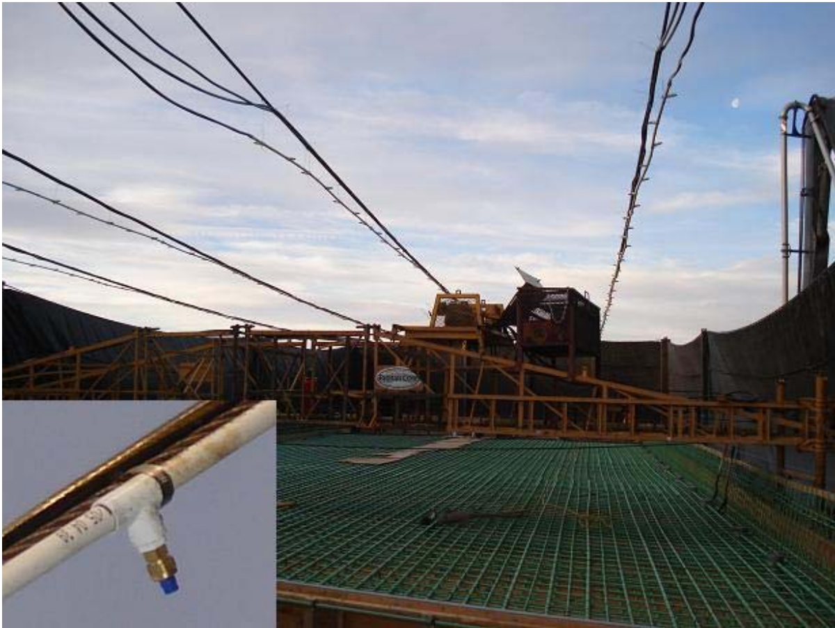
FIGURE 7 The fogging system installed at Bridge 5500.
