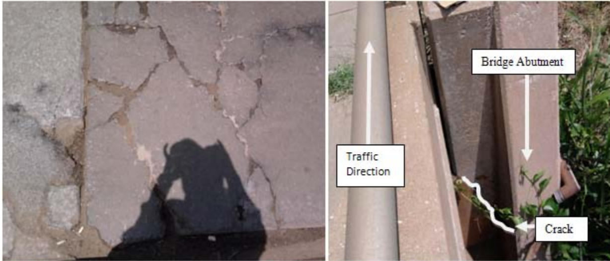
Figure 2.38 - Fines movement in first panels of intersection. Figure 2.39 - Cracking in abutments of the bridge.
