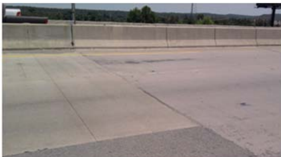
Figure 2.12 – The overlay terminates at a bridge and does not show any distress.
