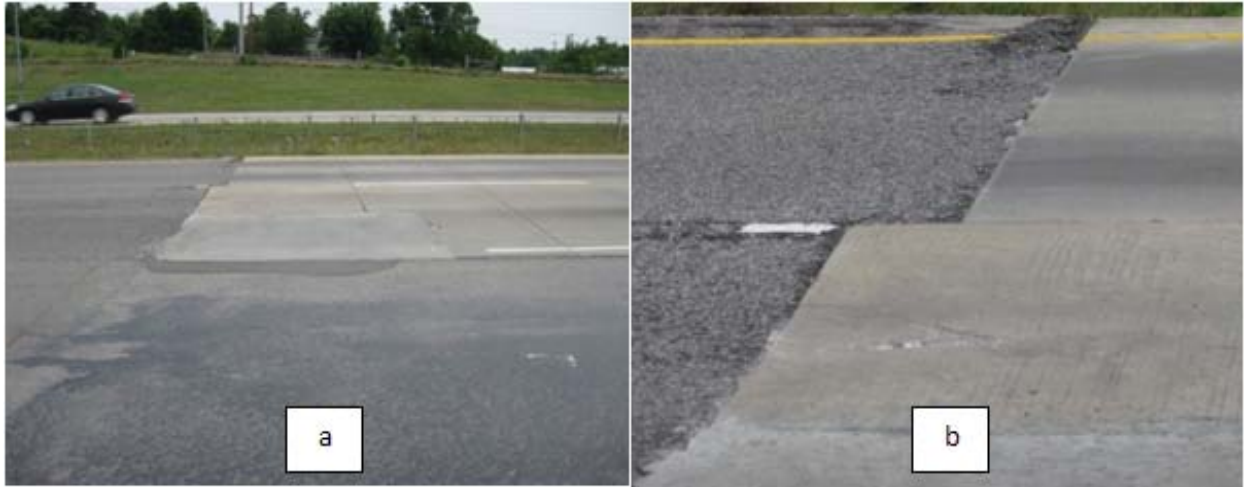
Figure 2.10 - Initial panel replacement at the start of overlay as seen in photo a, and in photo b we see how there is an elevation difference between the leaving asphalt panel and approaching concrete panel.
