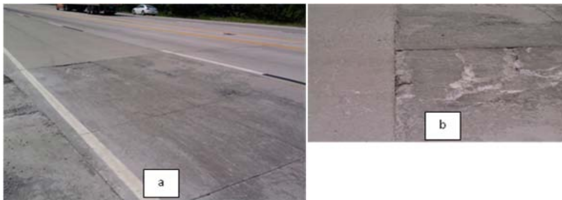
Figure 2.17 – Photo a shows a cracked panel at the start of an overlay. Photo b shows a closer view of that panel.
