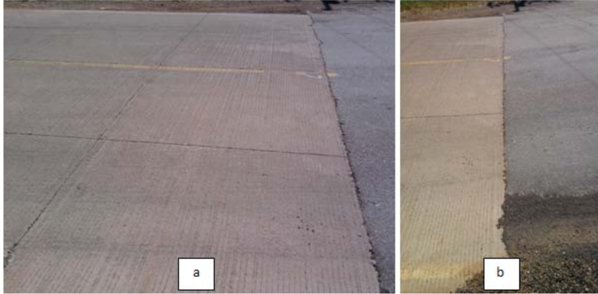
Figure 2.50 - Photos a and b show approach panels in un-distressed condition. Elevation difference between leaving asphalt pavement and approaching concrete panels is almost zero.
