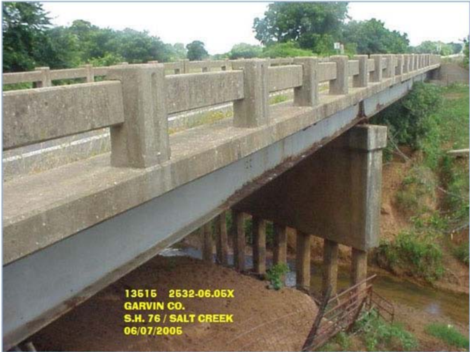
Figure 35. Picture demonstrating extent of damage to piers at bridge 13515 on SH 76 over Salt Creek.
