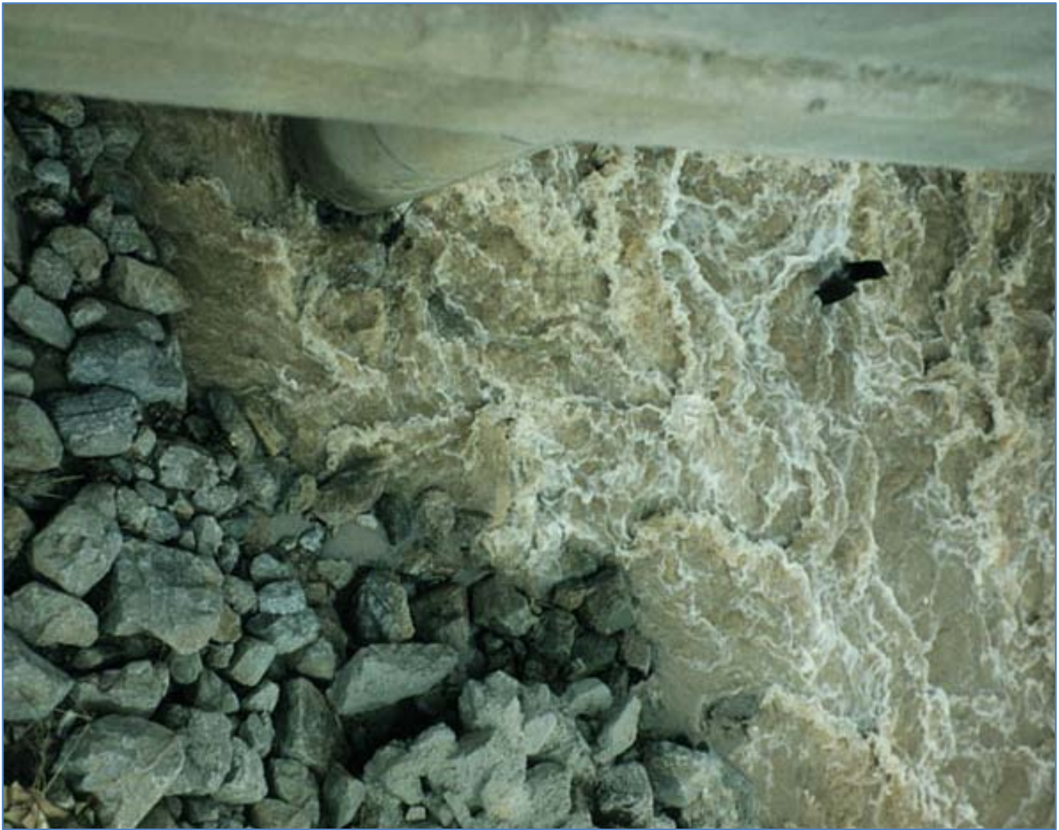
Figure 28. Picture demonstrating extent of damage to piers (b21120).
