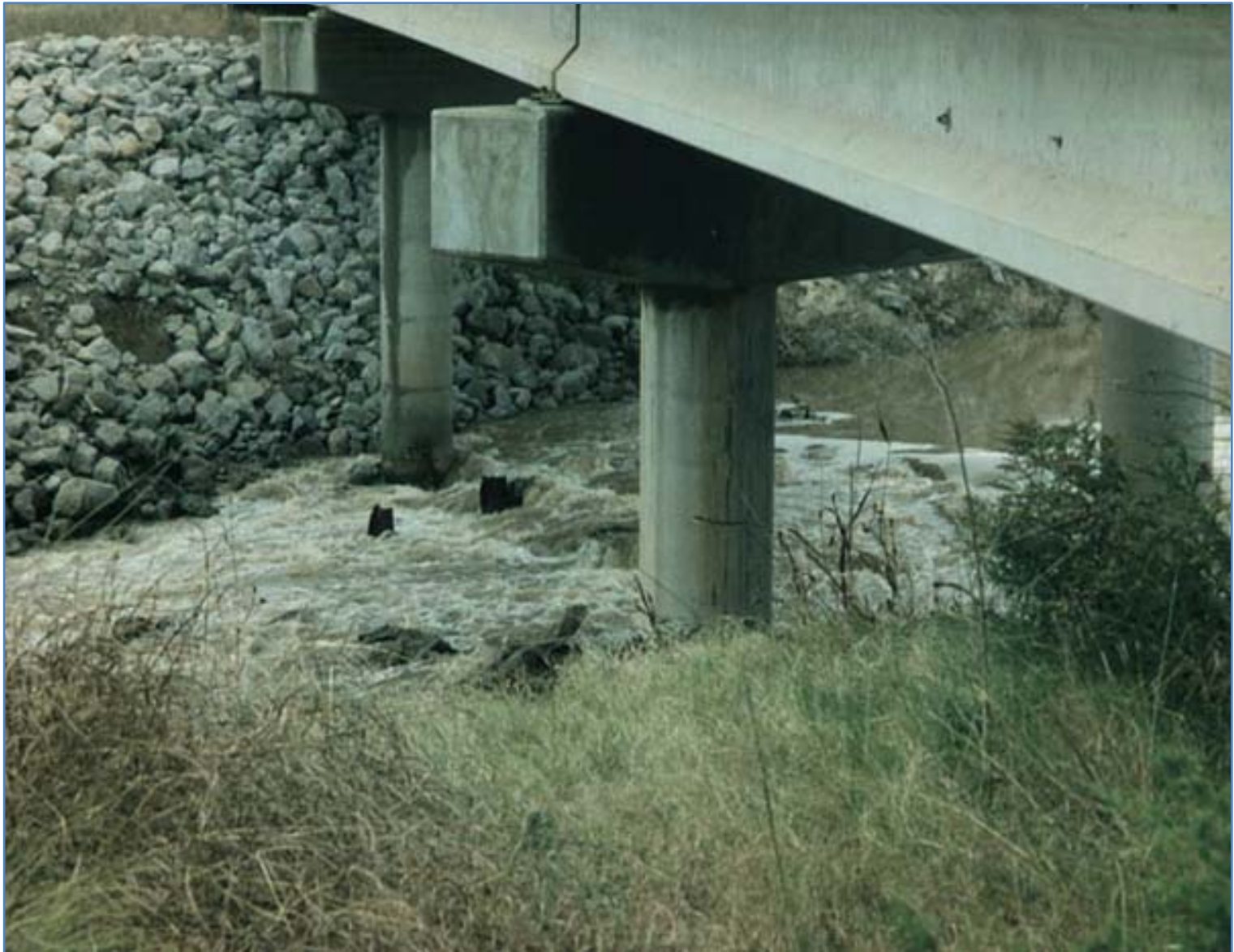
Figure 27. Picture demonstrating extent of damage to piers at bridge 21120 on SH 74 over Wildhorse Creek.
