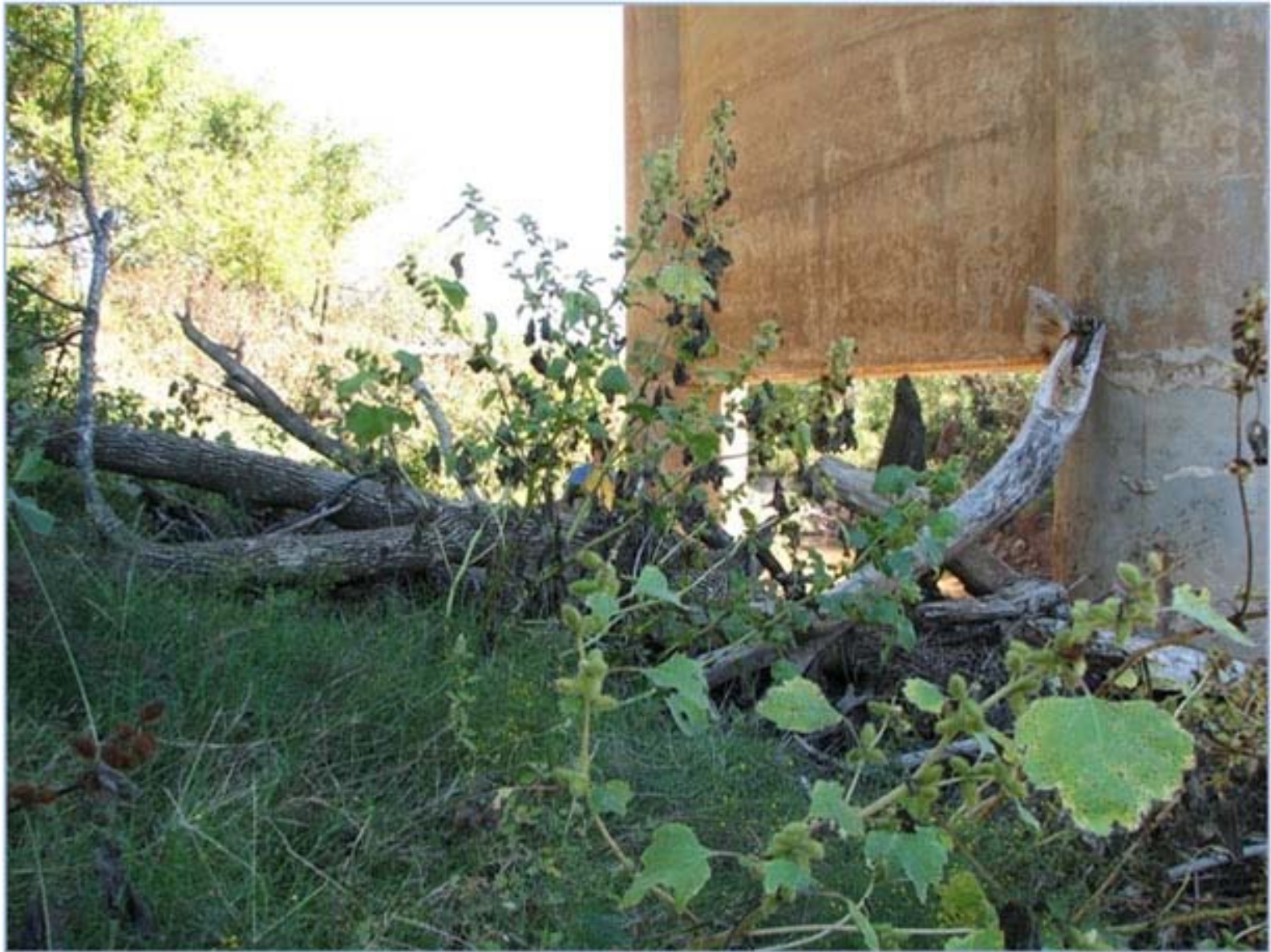
Figure 30. Picture demonstrating extent of damage to piers at bridge 13235 on SH 76 over Wildhorse Creek.
