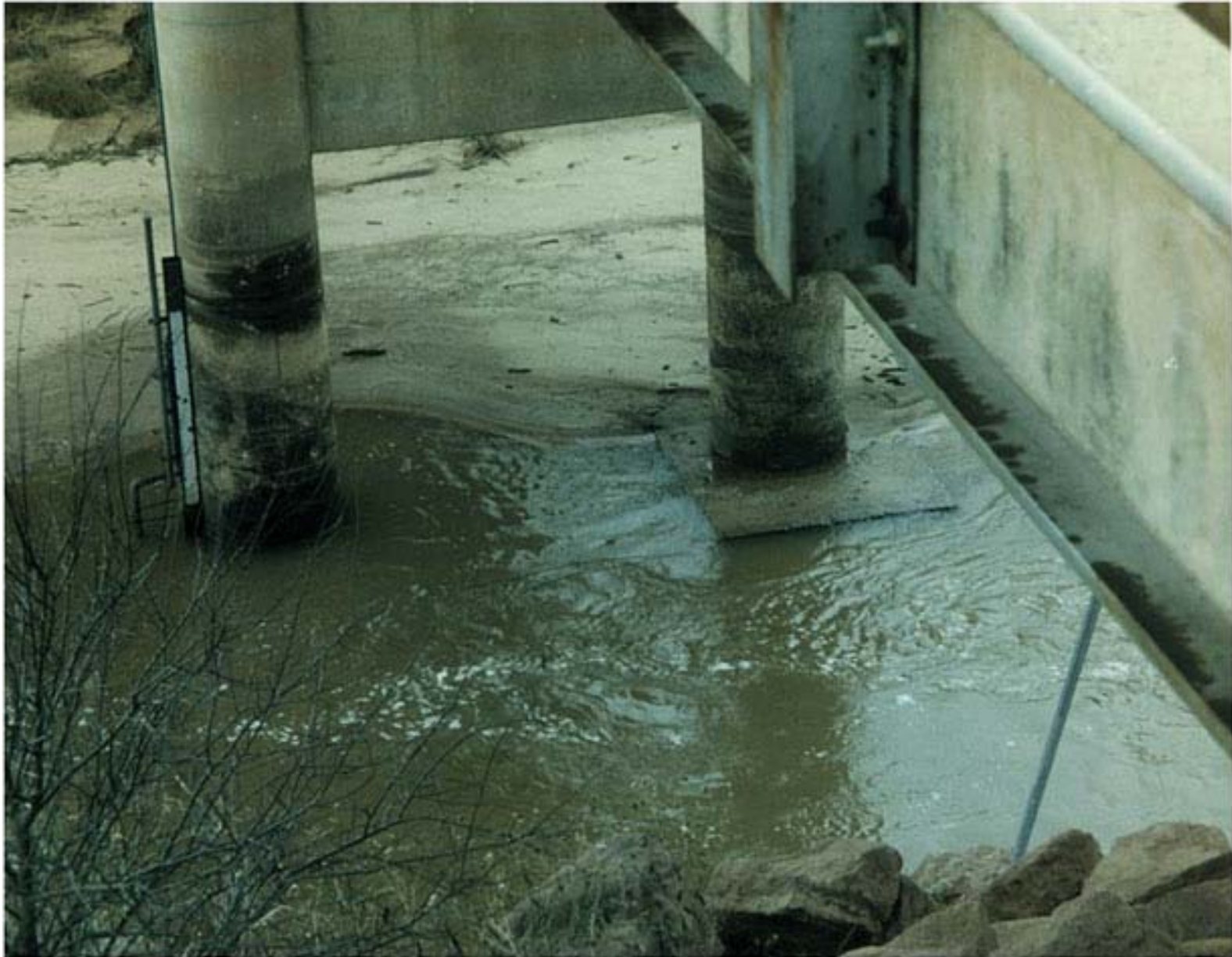
Figure 21. Picture demonstrating extent of damage to pier.
