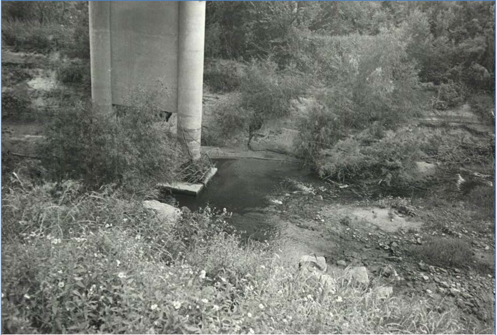
Figure 22. Picture demonstrating extent of damage to pier ar bridge 12643 on SH 76 over Rush Creek.
