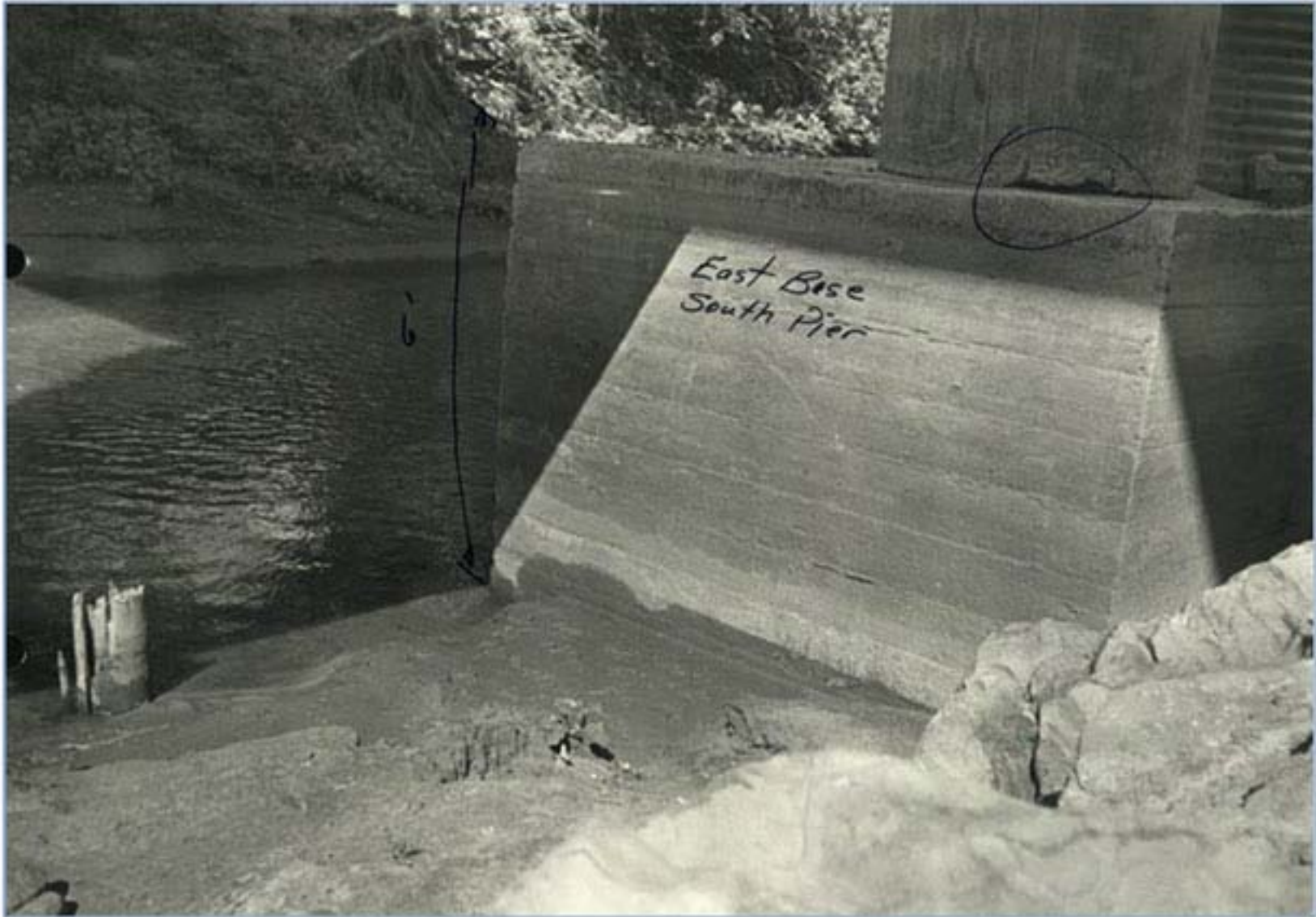
Figure 20. Picture demonstrating extent of damage to south pier at bridge 10738 on SH 74 over Rush Creek.
