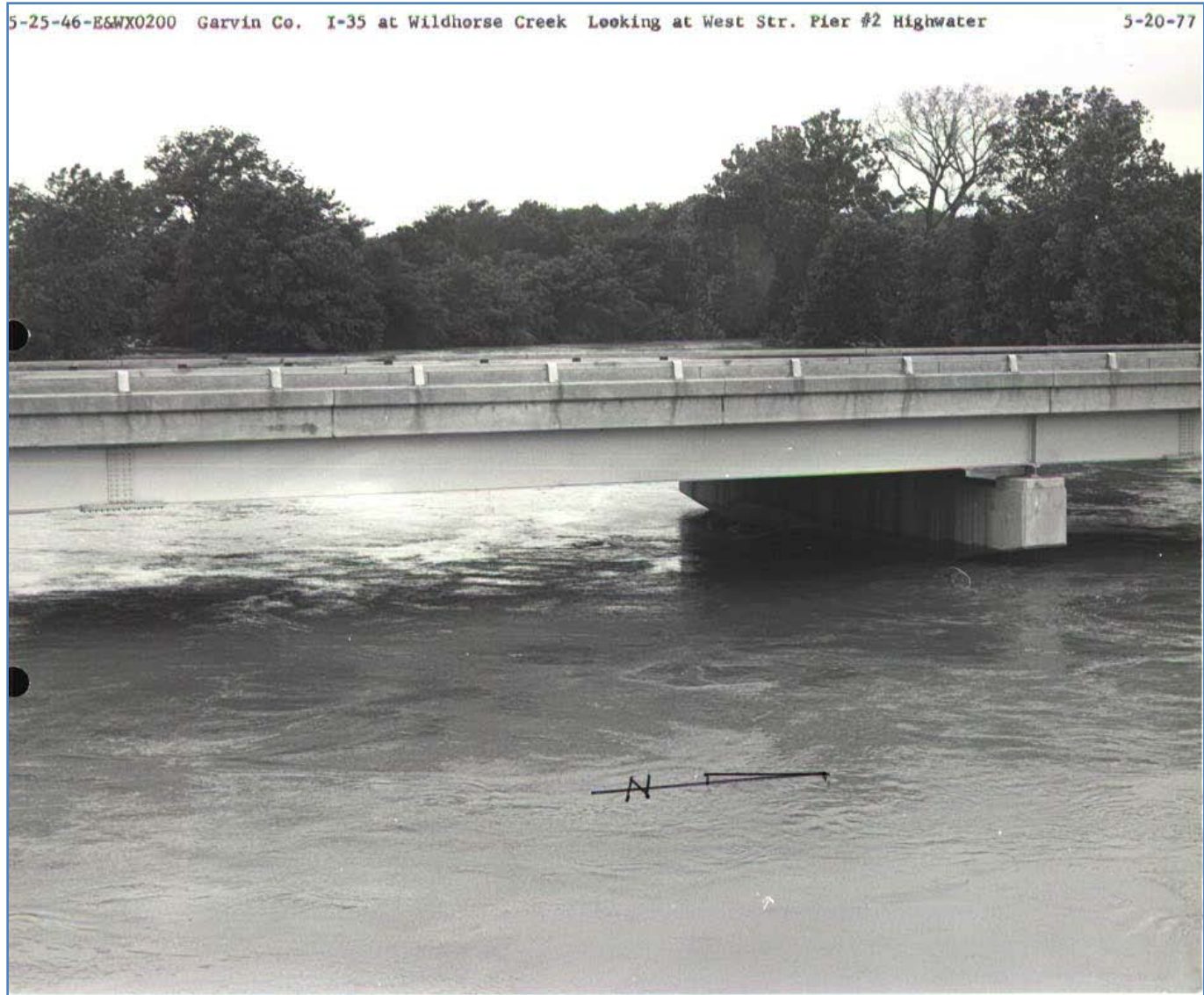
Figure 24. Picture demonstrating flood water level at pier at bridge 17590 on I-35 NB over Wildhorse Creek.
