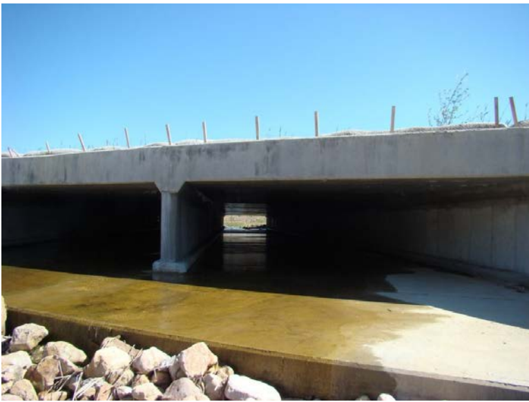
Figure 5.16 Structure #52-462-326 after One Winter in Service
