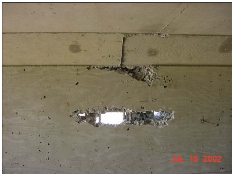
Figure 1.1 Concrete Void in the Wall of a Cast-In-Place Box Culvert (Courtesy SDDOT)
