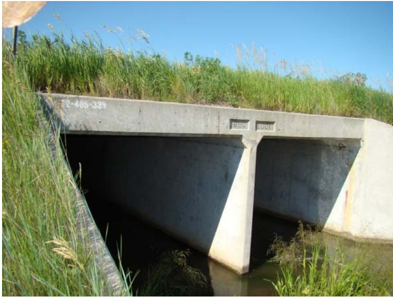
Figure 5.14 Structure #52-489-339 after One Winter in Service
