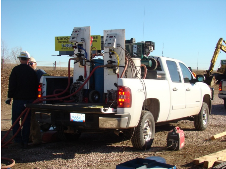
Figure 5.7 Superplasticizer and VMA Pump System
