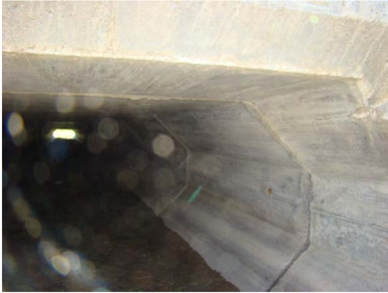
Figure 5.13 Structure #52-485-337 after One Winter in Service
