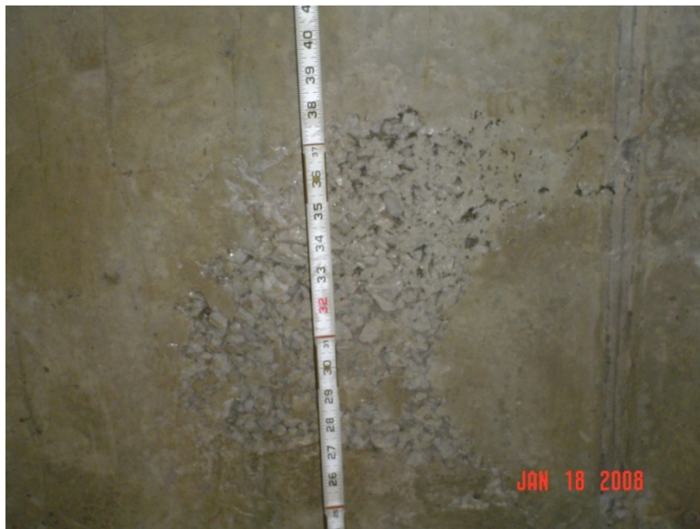
Figure 5.9 Honeycombing in the Wall of Structure #52-489-339
