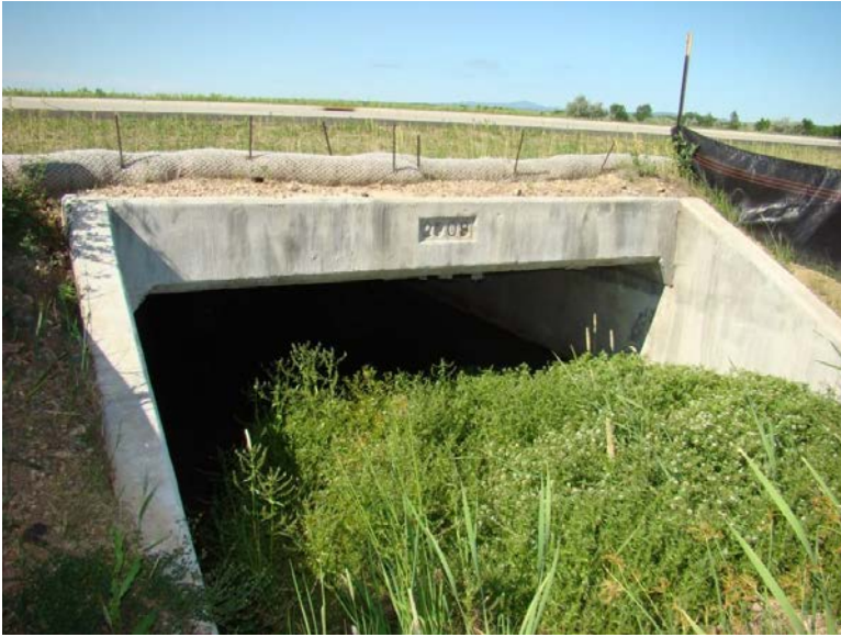
Figure 5.15 Structure #52-472-331 after One Winter in Service
