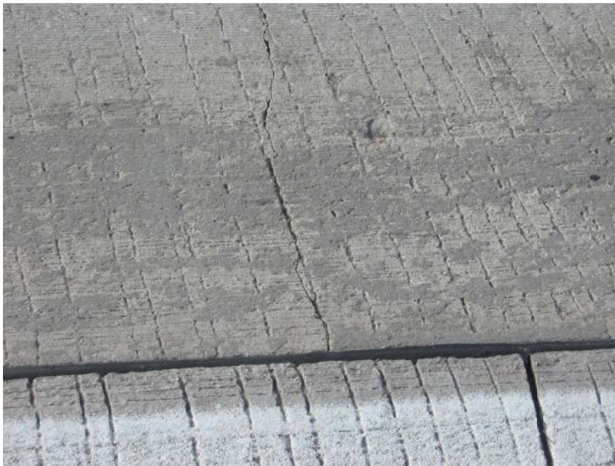
Figure 11. Close up view of transverse crack on Dan Ryan Expressway.
