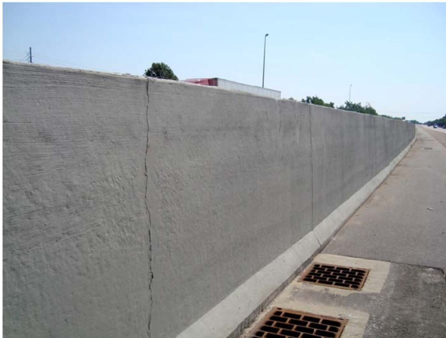
Figure 17. A crack in the barrier wall that appears to have been covered with a thin layer of paste, but has cracked through again.
