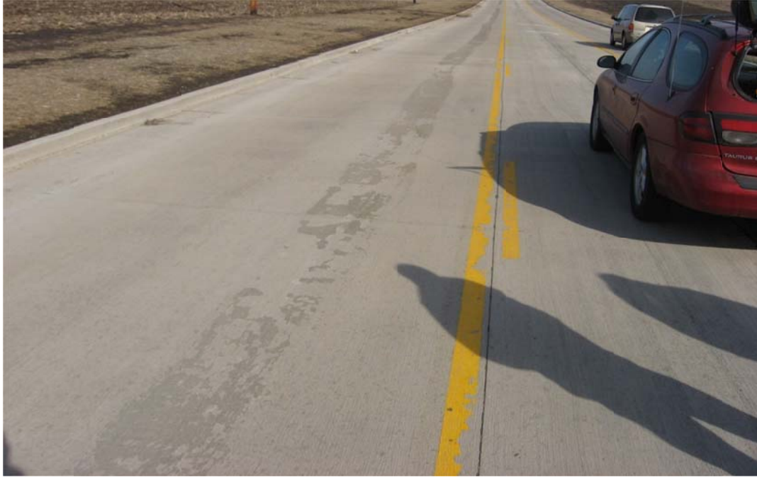
Figure 16. Westbound Cruger Road with proper surface texture (left lanes). The discoloration in the westbound lane is merely a cosmetic flaw.
