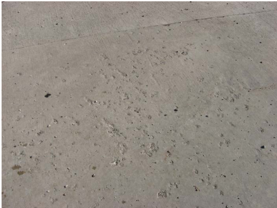
Figure 13. No surface texture and significant pop-out distress.
