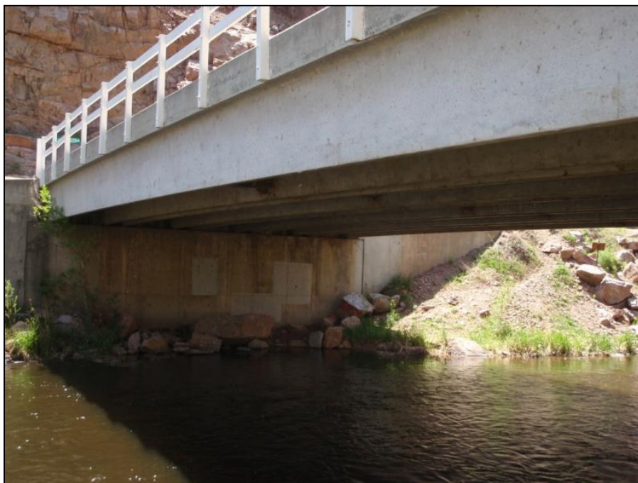
Figure E.22 Bridge 8 - Slight arch in bridge girders
