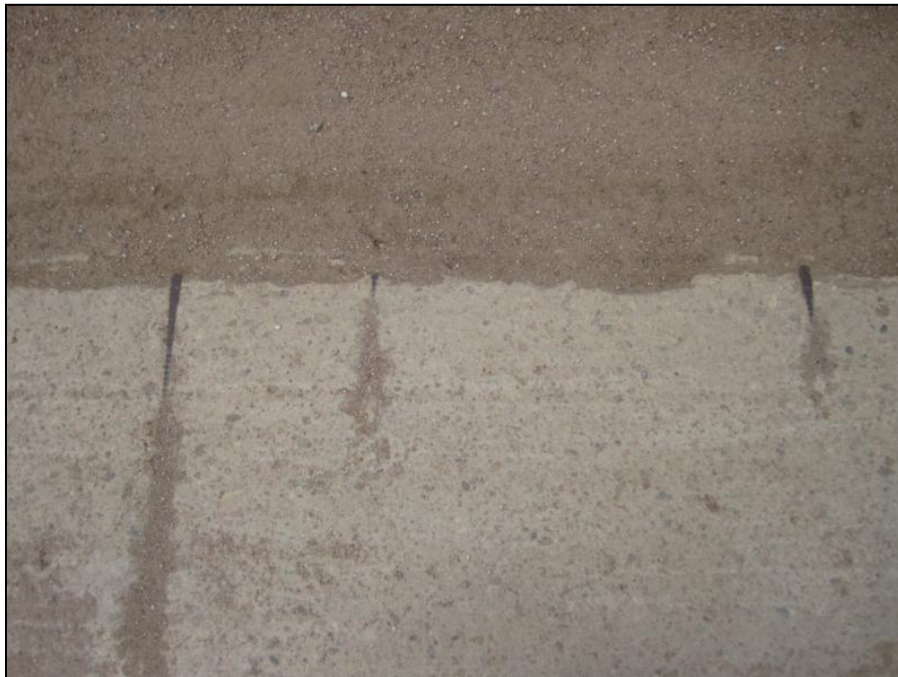
Figure E.55 Bridge 16 - Exposed rebar on wearing surface
