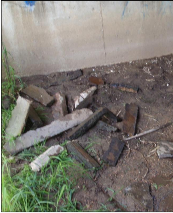
Figure 3.1 Concrete pieces from streambed underneath Bridge 12.
