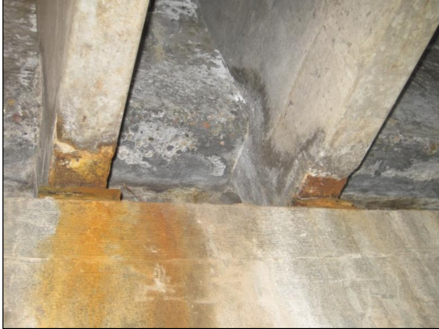
Figure E.25 Bridge 8 - Rust at supports
