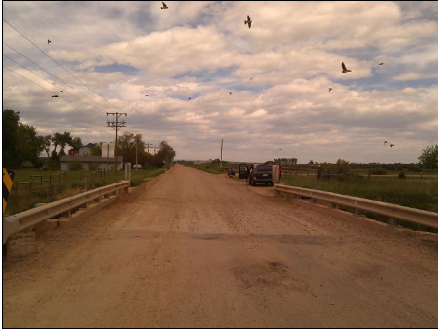
Figure E.7 Bridge 2 - Exposed Girder Flanges
