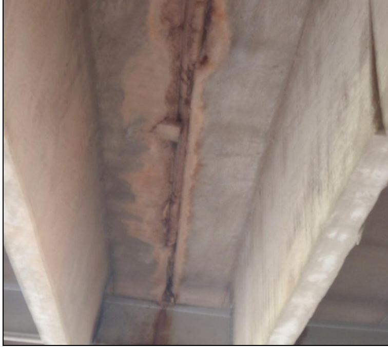
Figure E.58 Bridge 16 - Cracking at girder joint
