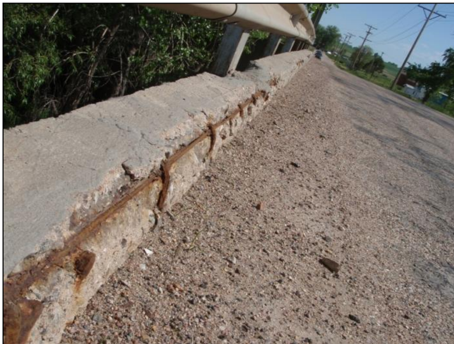
Figure E.2 Exposed Rebar on Bridge 1
