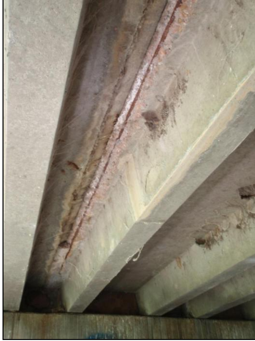
Figure E.40 Bridge 12 - Exposed rebar at girder joint
