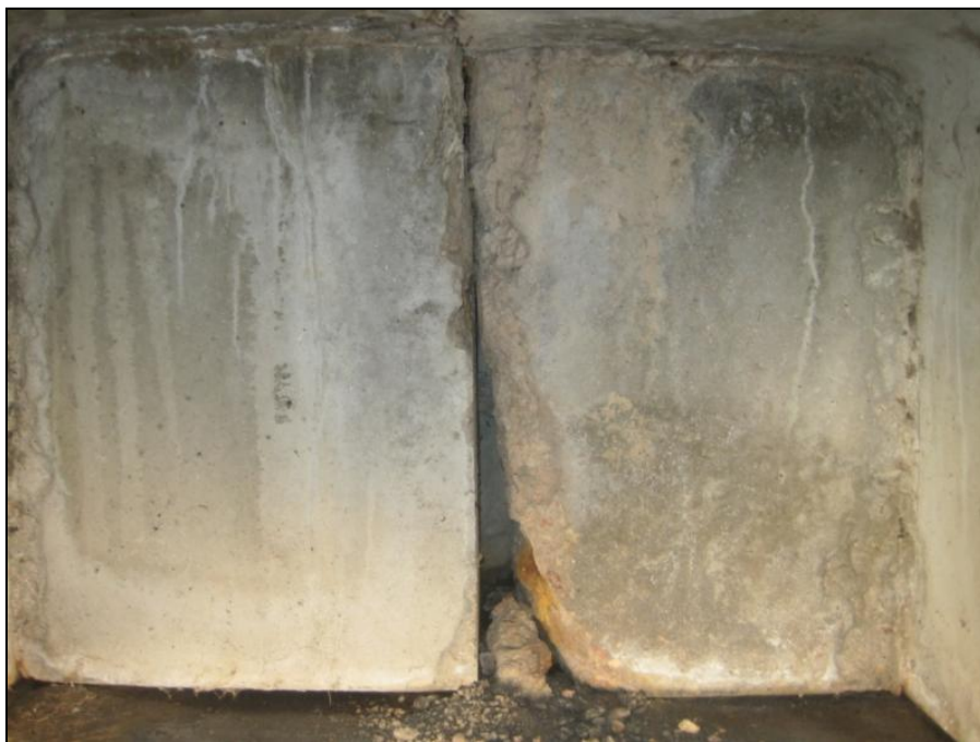
Figure E.16 Spalling of concrete on Bridge 6
