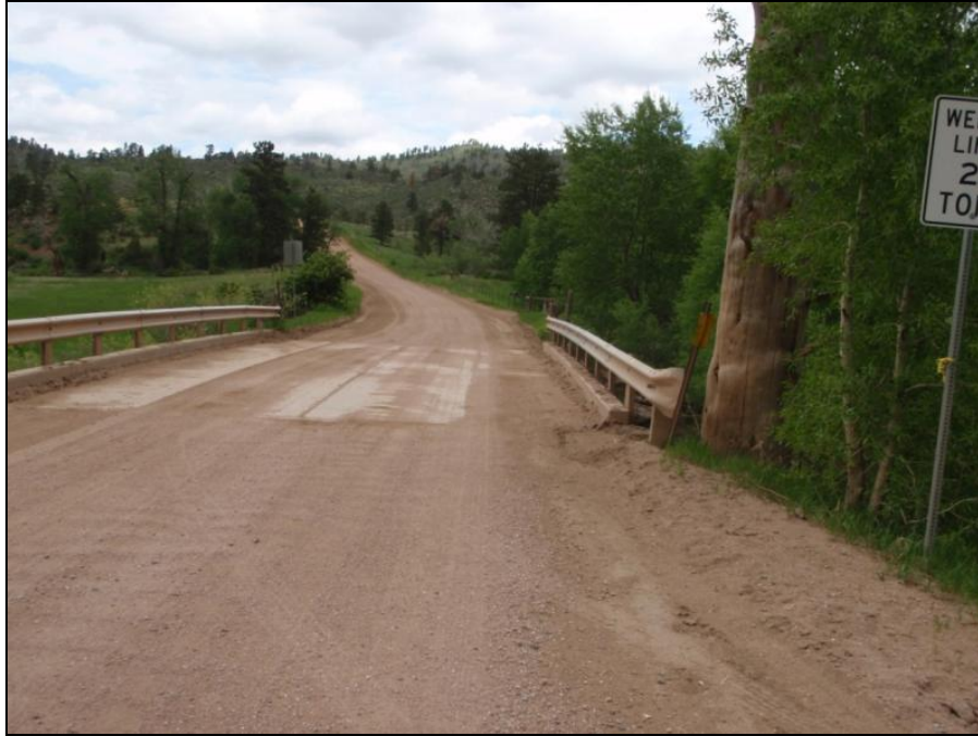
Figure E.56 Bridge 16 - Exposed Girder Flanges
