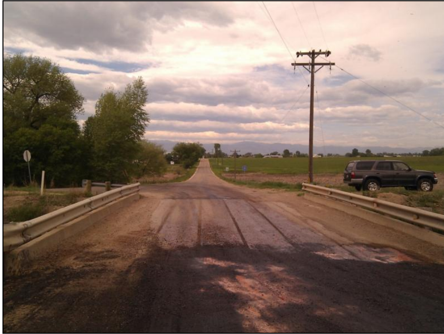
Figure E.36 Bridge 11 Deck - Exposed Flange
