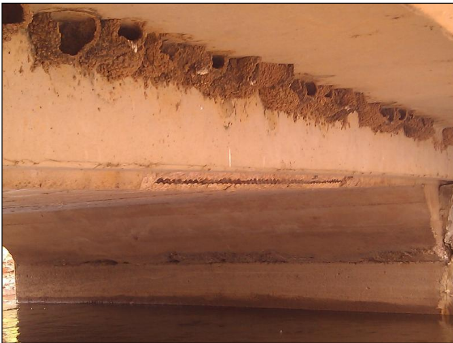
Figure E.51 Bridge 15 - Exposed Rebar
