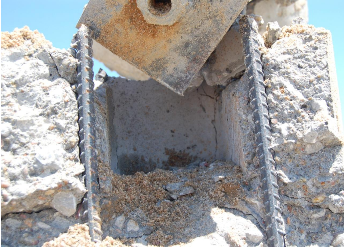
Figure 5.12 System Damage, Test No. HTC3-3
