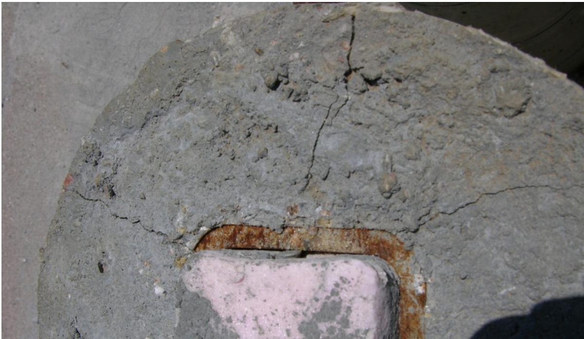
Figure 5.7 Concrete Damage, Test No. HTC2-2
