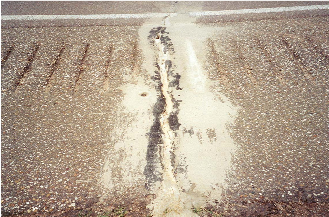
FIGURE 10 Treated transverse crack.
