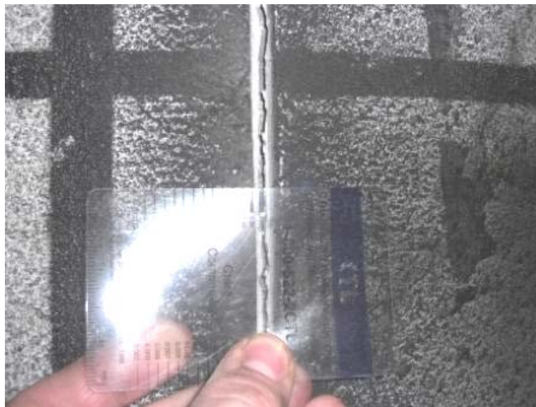
Figure 4.5: Original crack after jacket was cut
