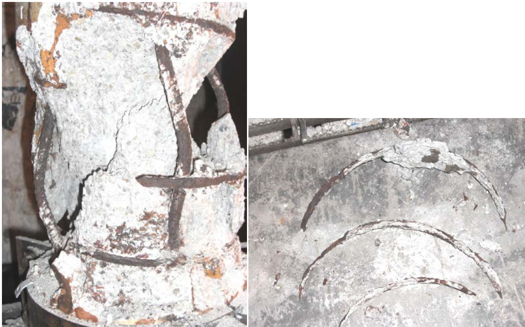
Figure 3.1: Effects of corrosion on steel spiral
