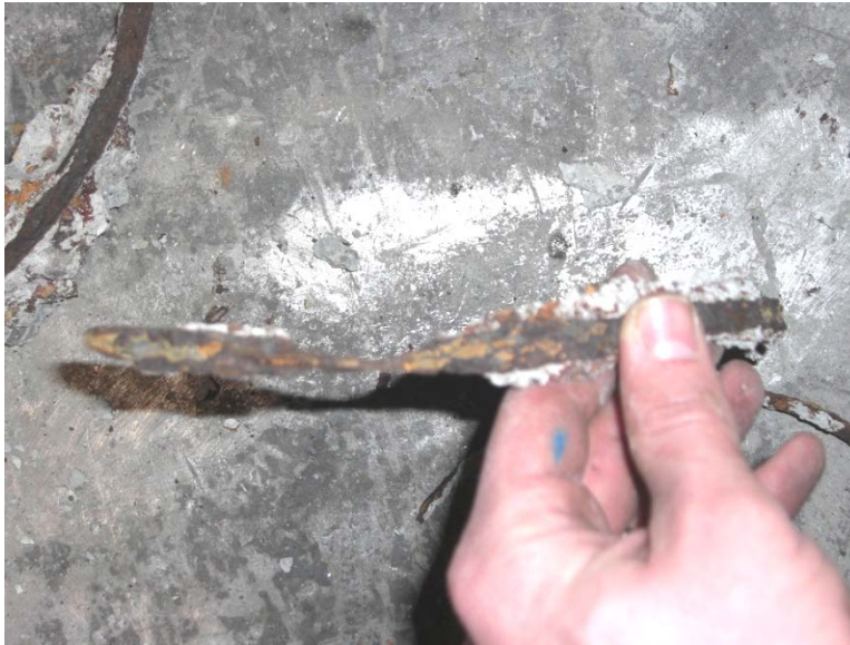
Figure 3.25: Section of spiral with more than 75% steel loss
