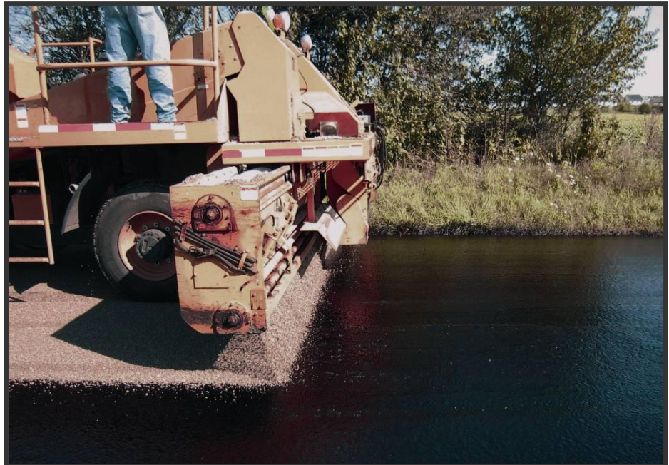
A chip spreader applies cover aggregate during a seal coat or "chip seal" operation on 74 th Street in Cedar Rapids, Iowa, during a road maintenance effort Photo: Dr. Charles Jahren, Iowa State University/CCEE
