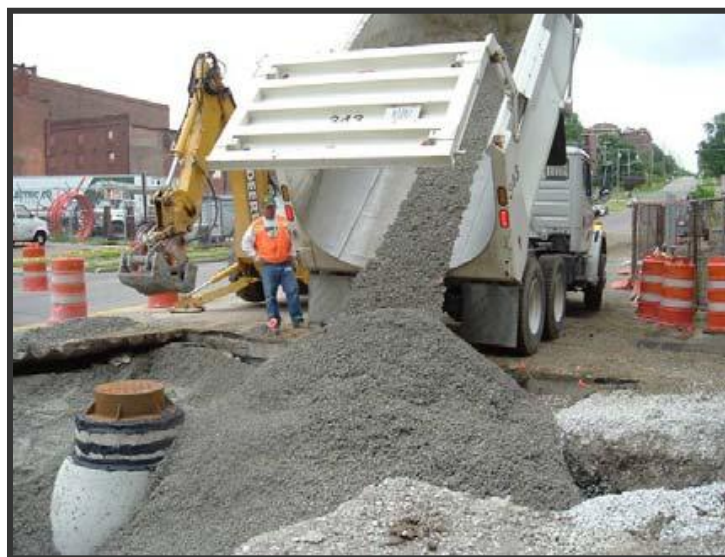
Large lift thickness used in utility cut trench backfilling Photo: Iowa State University/InTrans
