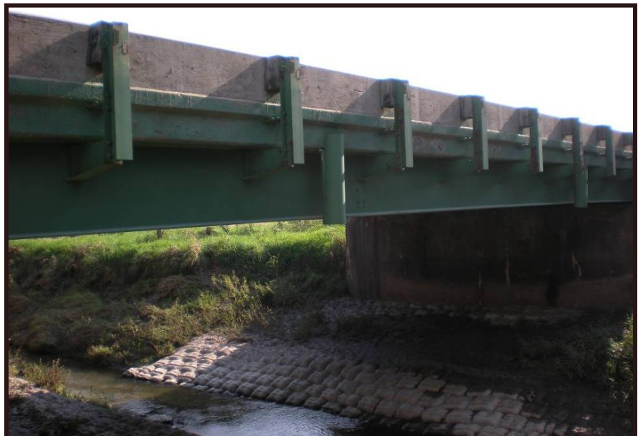
On-the Spot damage detection field testing on County IA-1, South of Iowa City, Iowa, near Gingerich Road
