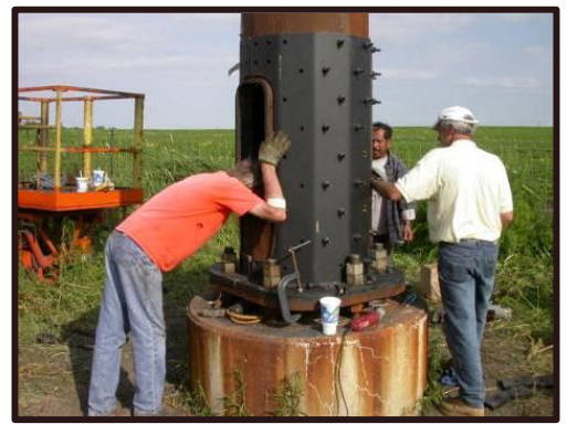
A bolted reinforcing jacket was placed on a tower in the I-35 & US 18 Interchange near Clear Lake
