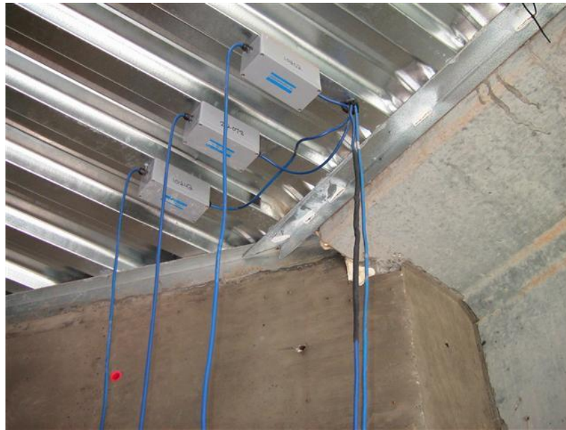
Figure 50 Surge protectors installed on one of every two embedded sensors at the same location
