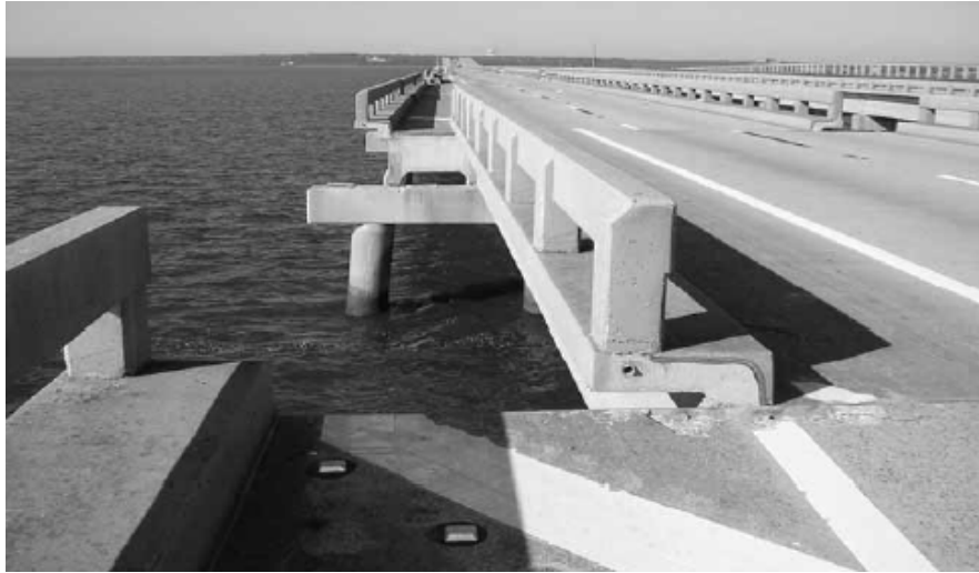
Figure 2.2 I-10 Bridge over Escambia Bay after Hurricane Ivan (Sheppard).
