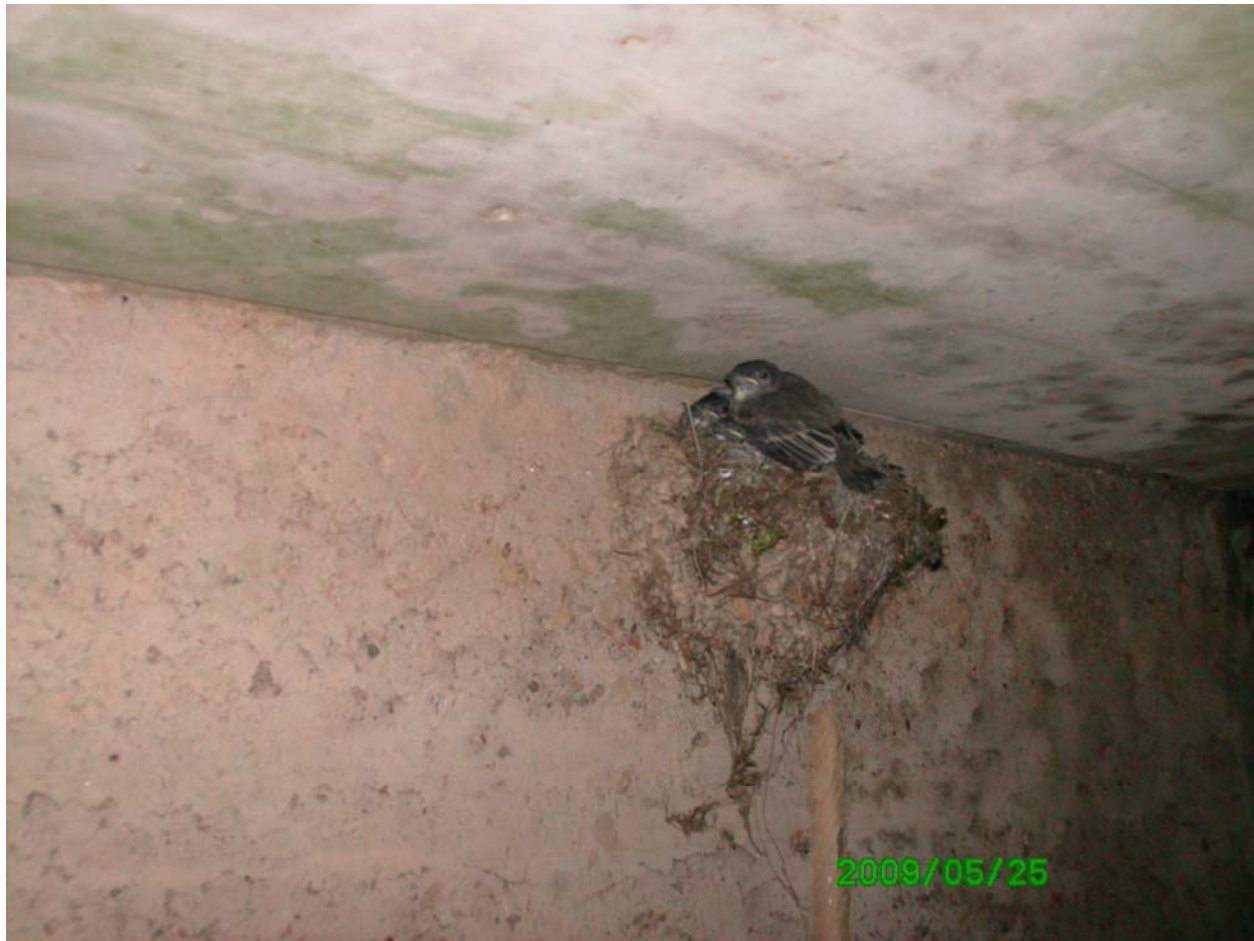
Figure 15. Eastern phoebe nestlings in a nest on a wall of a box culvert in Maryland.
