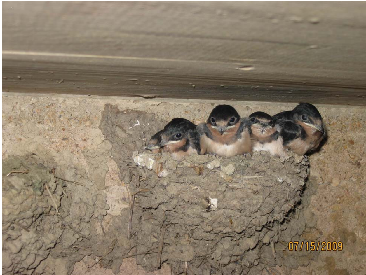
Figure 14. Barn swallow nestlings in a nest on the wall of a box culvert in Maryland.
