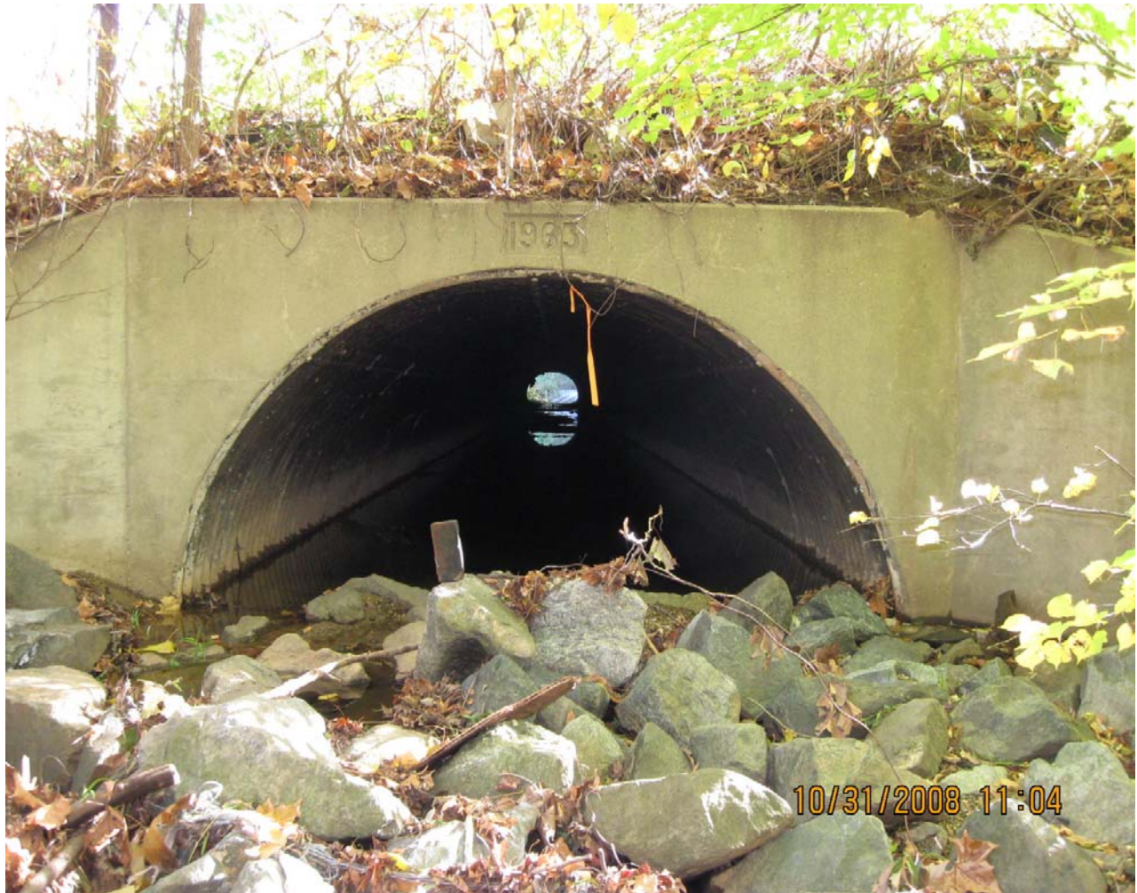
Figure 1. Culvert 15138X0 is 11 feet, 10 inches (3.6 m) wide, 7 feet 7 inches (2.3 m) tall, and 256 feet (78.8 m) long with 6 inches (15 cm) of water. This arch culvert cell had a gravel and sand substrate.
