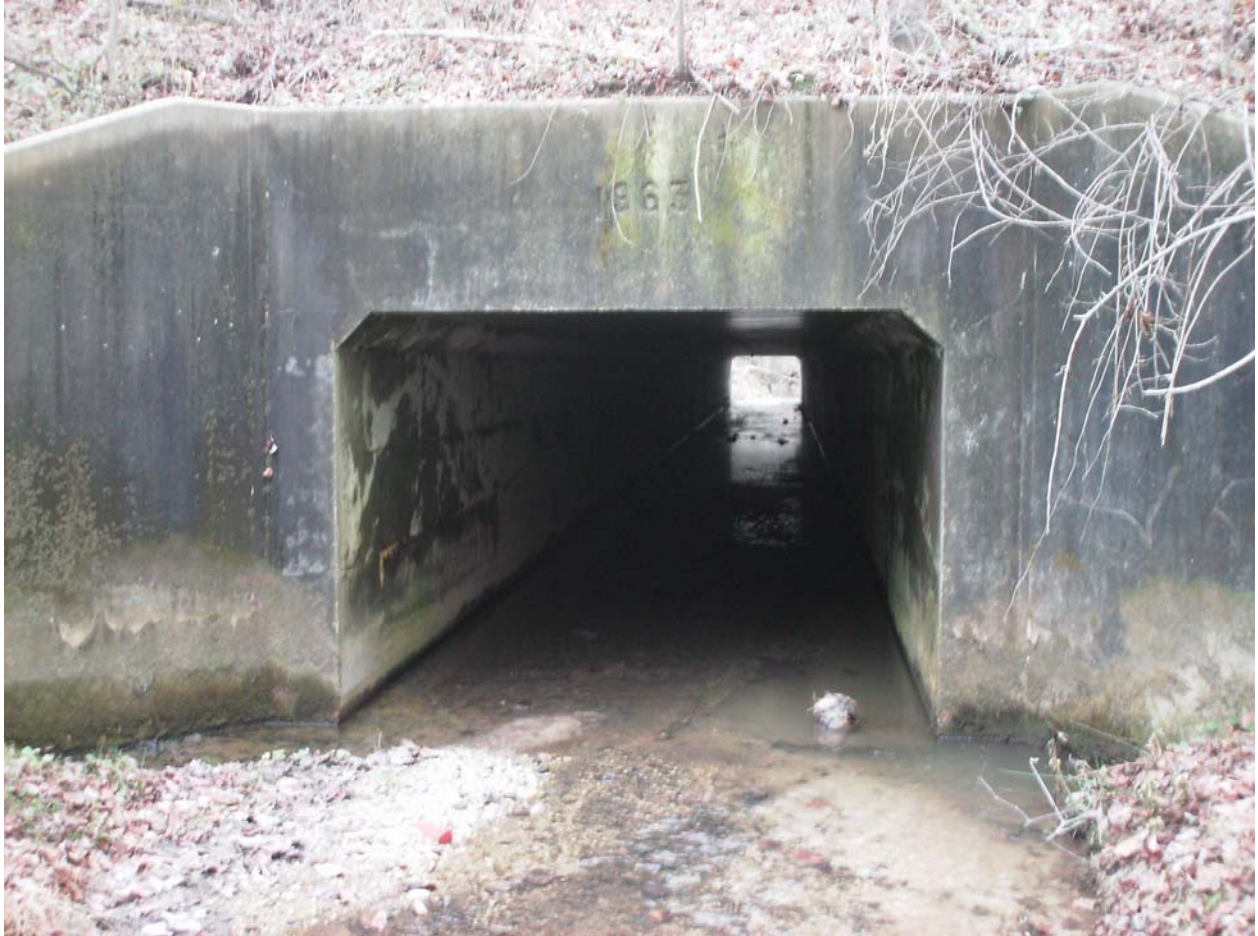
Figure 2. Culvert 02015X0 is 8 feet (2.4 m) wide, 6 feet (1.8 m) tall by 104 feet (31.7 m) long with 3 inches (7.6 cm) of water. This box culvert cell had a concrete substrate.
