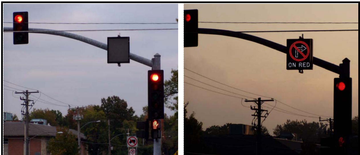
Figure 7-13. Blank-Out Signs Used to Control Right-Turn Movements by Time of Day. (Left: Off-mode vs. Right: Active-mode where right turns are prohibited)
