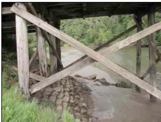
Figure 22. Bank under structure on north side
