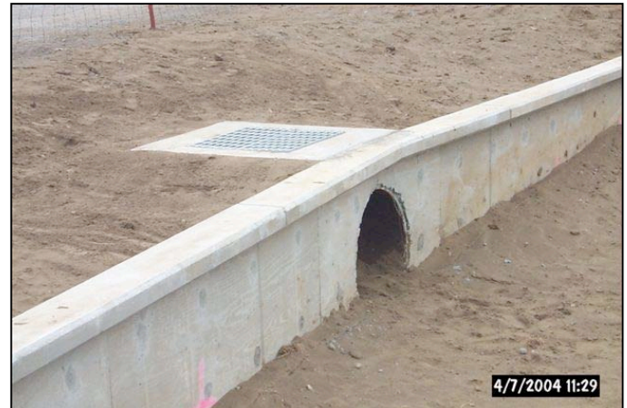
Figure 11. Turtle culvert, wall, and grate ©Port of Portland
