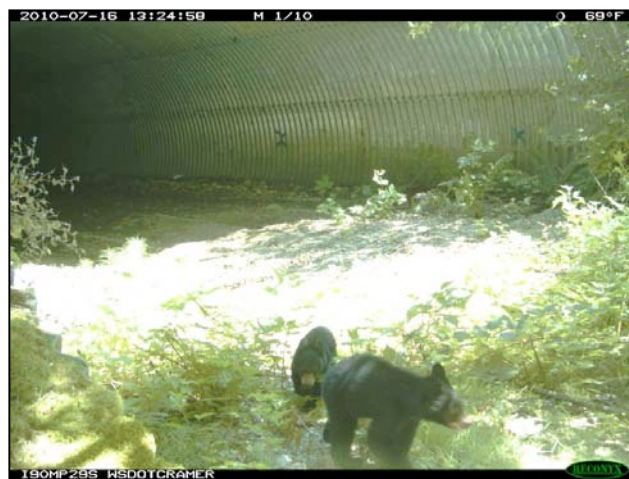
Figure 15. Black bear cubs passing through culvert behind mom, under I-90 Washington © P. Cramer, J. Kintsch & WSDOT
