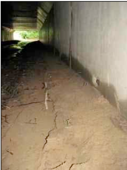
Figure 3. Muddy pathway through culvert
