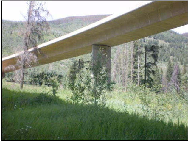
Figure 34. Example of a Class 4 extensive bridge or viaduct, I-70 Colorado © J. Kintsch
