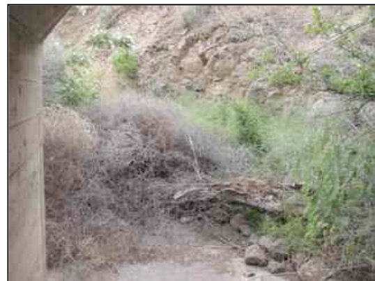
Figure 65. Debris at culvert outlet
