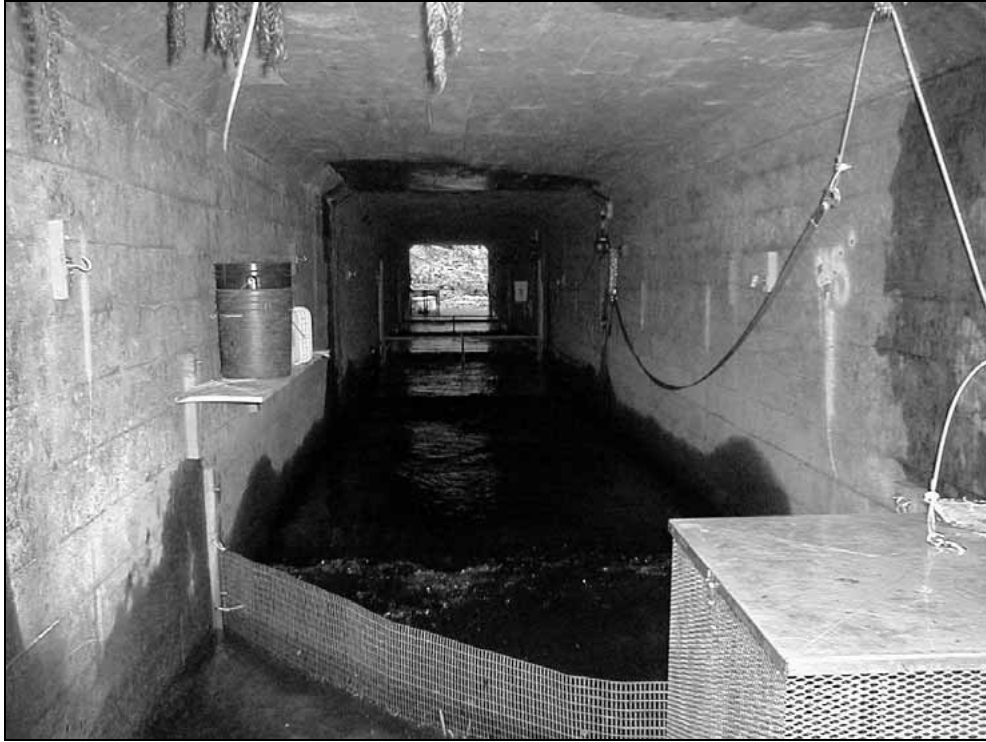
Figure 2.11: Downstream end of culvert on Big Noise Creek, illustrating the lower fish trap.
