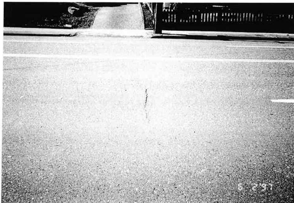
Figure 5.3: Typical Cracking in the Control Section
