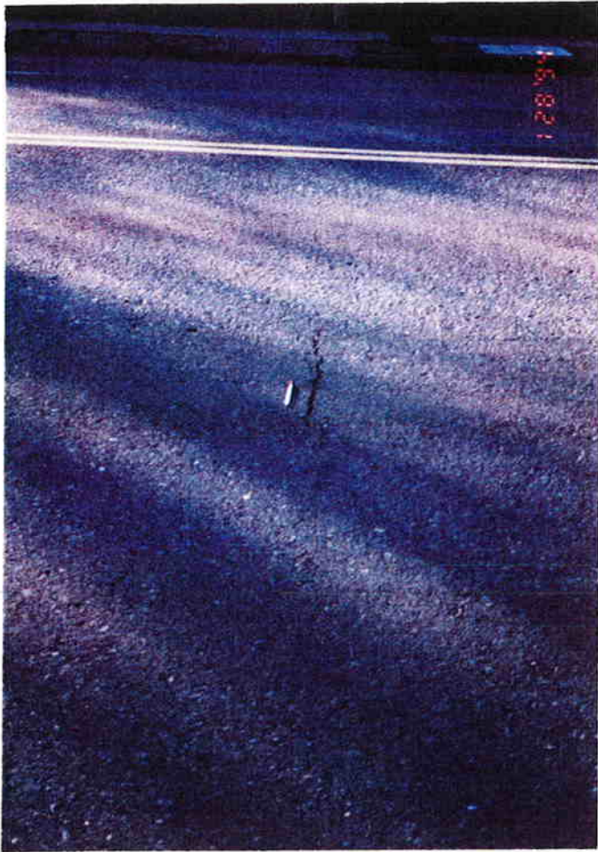
(a) Cracks in the AC Overlay in the Pavement Reinforcement (Glasgrid) Control Section
