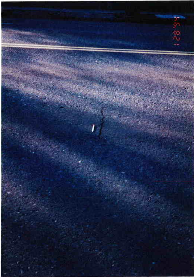
(a) Cracks in the AC Overlay in the Pavement Reinforcement (Glasgrid) Control Section
