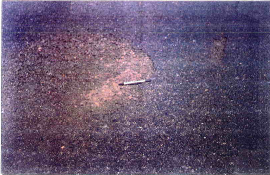
Figure 3.28 Close-up of raveled section.
