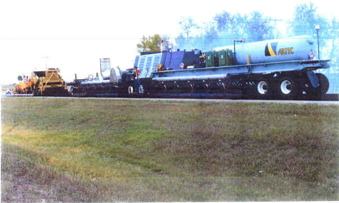
Figure 2.21 Close-up of Artec multi-stage second heater/miller (unit 3) and paver. (Photo courtesy of ARTEC.)
