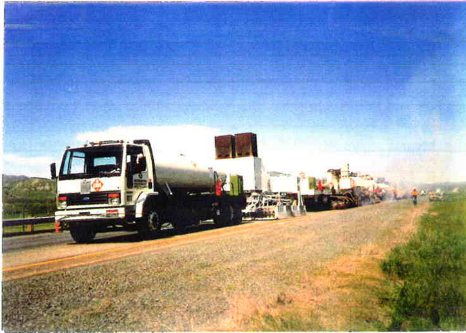
Figure 2.4 Pyrotech PYROPAVER 300E preheater (unit 1).
