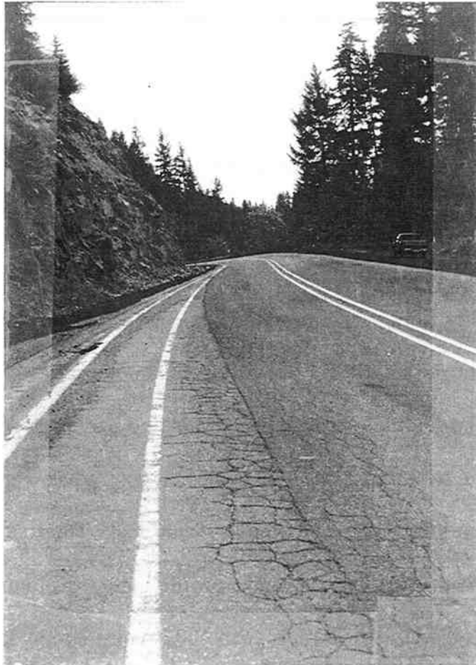
Figure 3.18 Section where cracking in pre-HIR pavement has reflected through near mile point 5.1.
