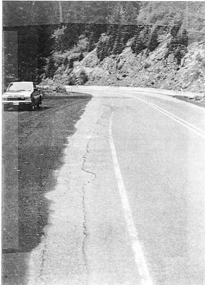
Figure 3.20 Section where HIR pavement has irregular edge seam near mile point 5.4.
