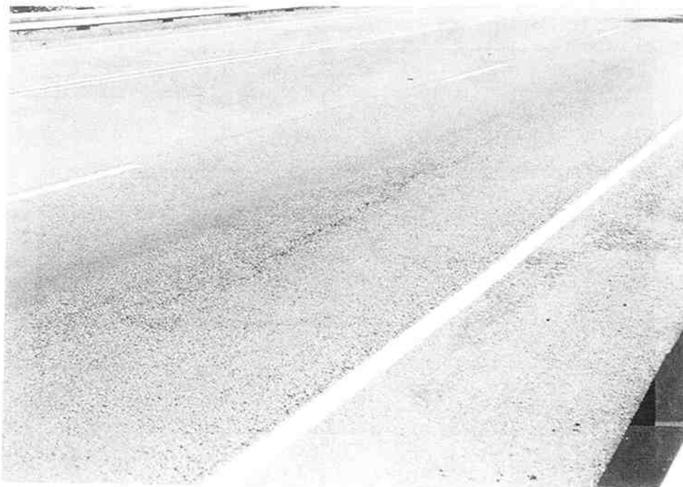
Figure 3.37 Close-up cracking near mile point 30.6.
