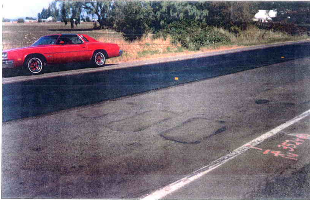
Figure 3.24 Section contrasting pre- and post-HIR pavement. The patched areas mark where the pre-construction pavement was milled.
