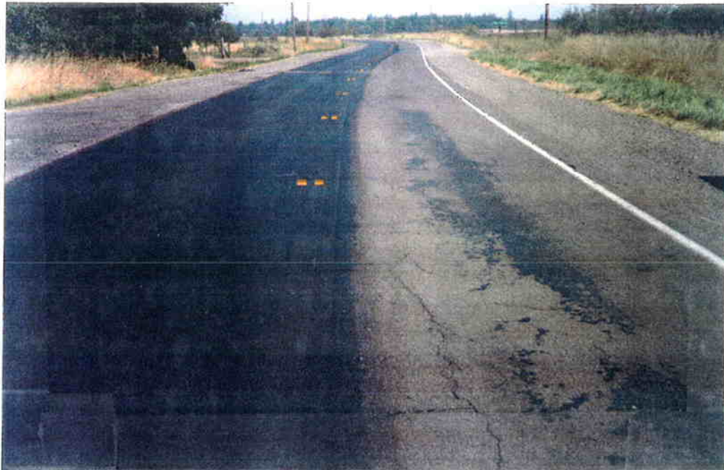
Figure 3.25 Section showing cracking and apparent flushing.
