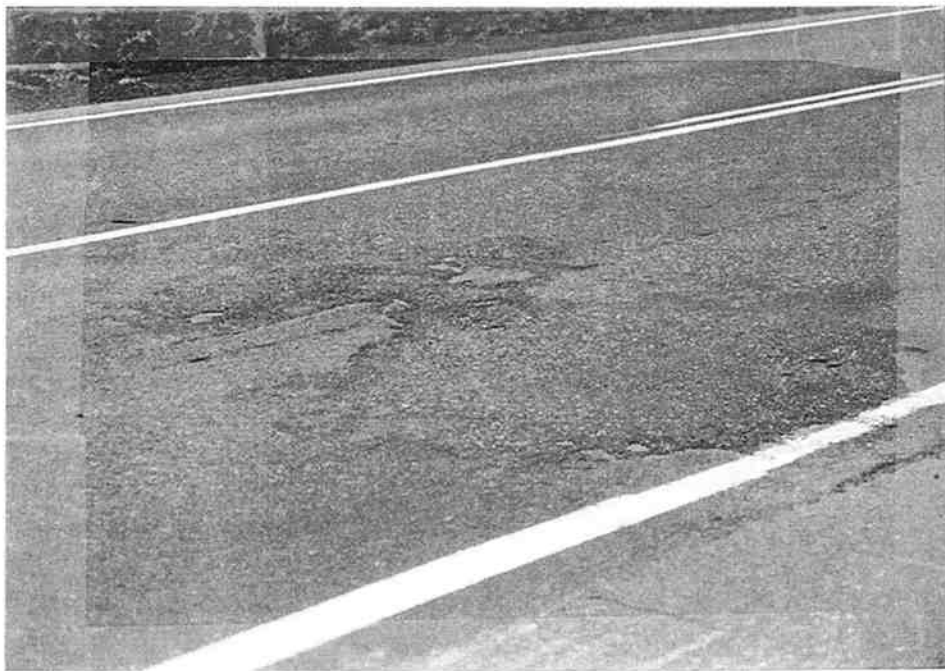
Figure 3.6 Minor problem area, what appears to be a previous coring site. (Looking northward near mile point 17.7.)
