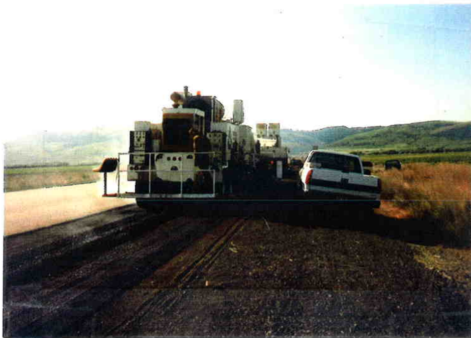
Figure 2.7 Milled RAP being windrowed into the center four feet of highway lane.
