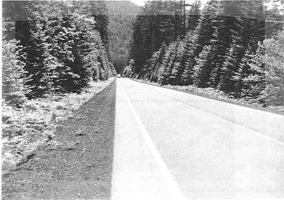
Figure 3.5 Good section on Clear Lake-Old McKenzie Hwy. two years after HIR. (Looking southward near mile point 17.7.)
