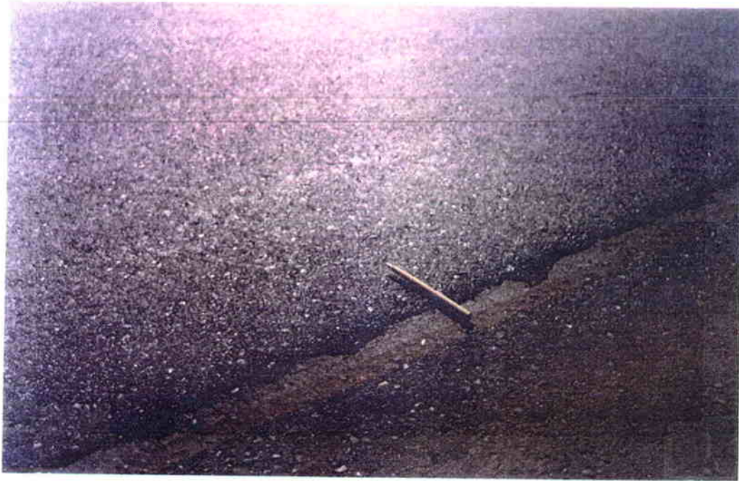
Figure 3.26 Section showing the raised edge seam produced by the added virgin mix.
