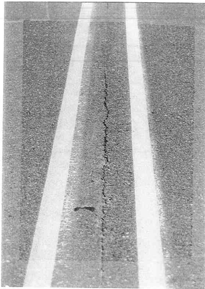
Figure 3.8 Section where centerline "seam" pulled apart near mile point 12.8.
