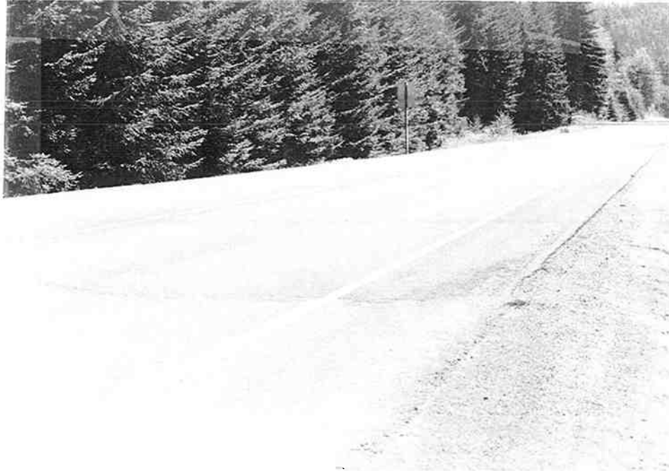
Figure 3.30 Photograph (looking East) of the patched area marking beginning of the HIR project near mile point 31.4.
