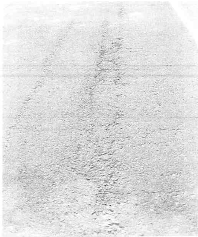
Figure 3.34 Close-up of the poor section near mile point 30.9.
