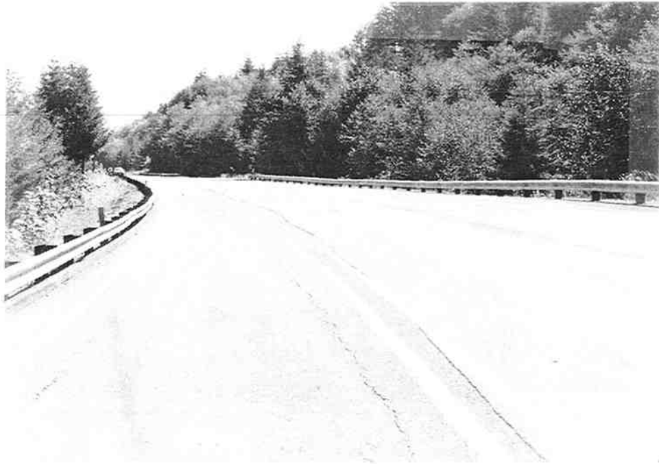
Figure 3.38 Section with "wandering" edge seam between HIR and non-HIR lanes near mile point 30.4. This photograph also shows raveling and cracking in this section.
