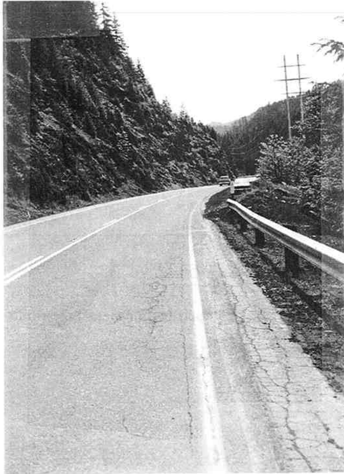
Figure 3.11 Section with reflective cracking breaking through the HIR pavement near mile point 11.1.
