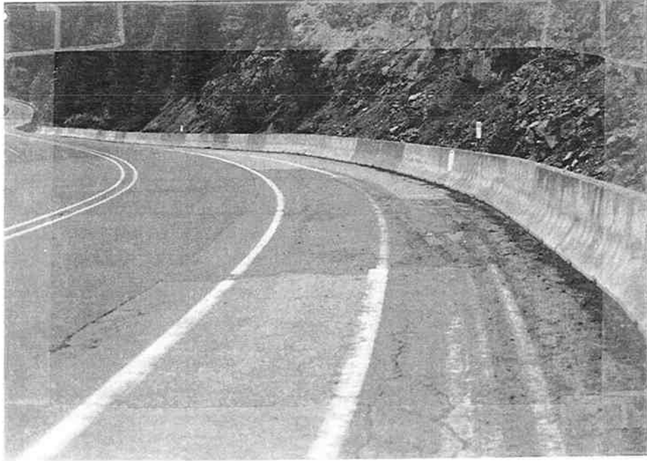
Figure 3.21 HIR edge seam well inside of fogline near mile point 5.4.
