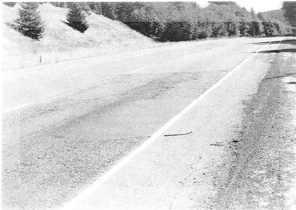
Figure 3.35 Patched, very rough looking section followed by a very good section near mile point 30.8.
