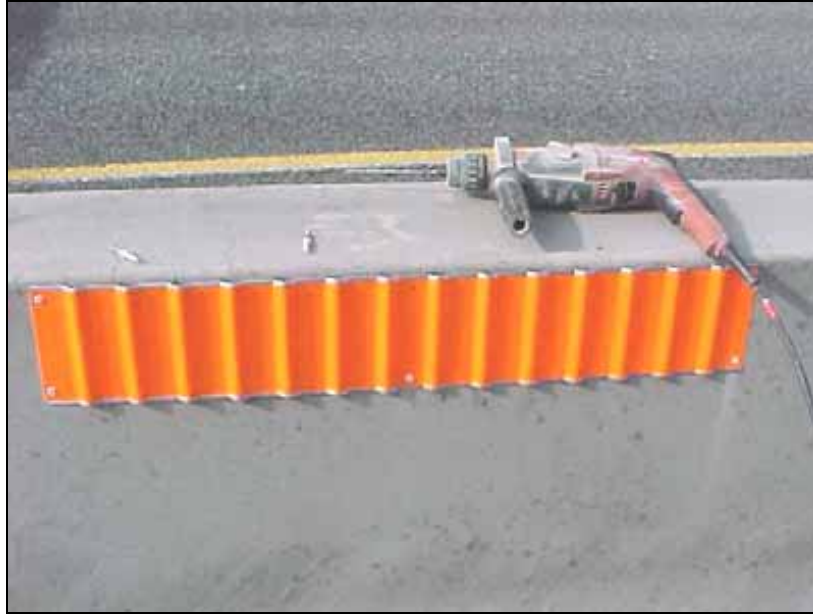
Figure 1.4: Drill and anchor bolts used to attach 3M™ LDS panels to the concrete barrier
