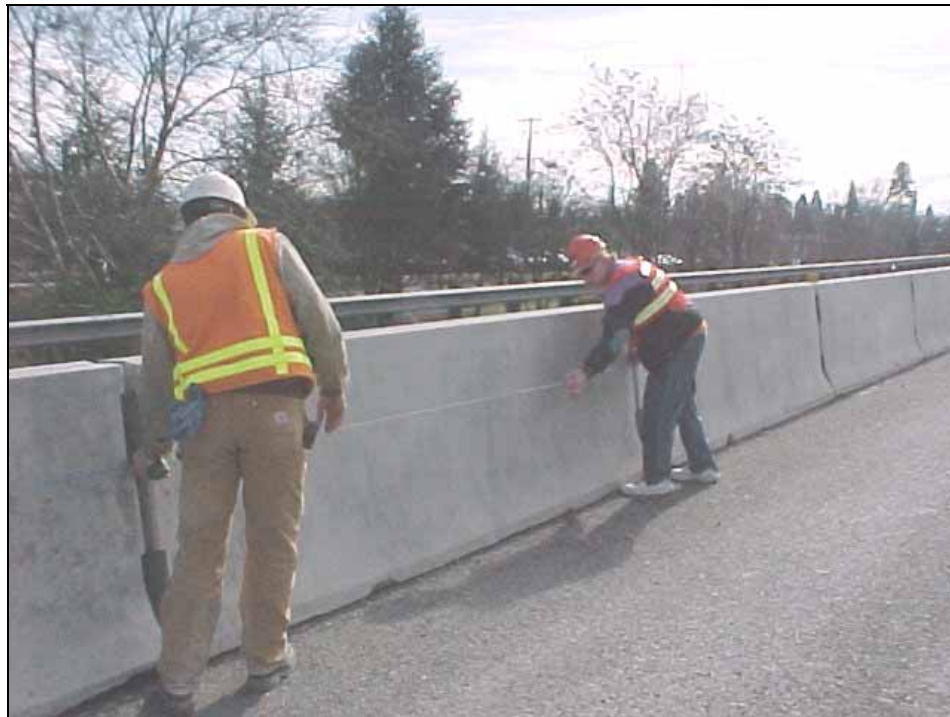
Figure 4.1: Snapping a chalk line on the concrete barrier at the Medford Viaduct project
