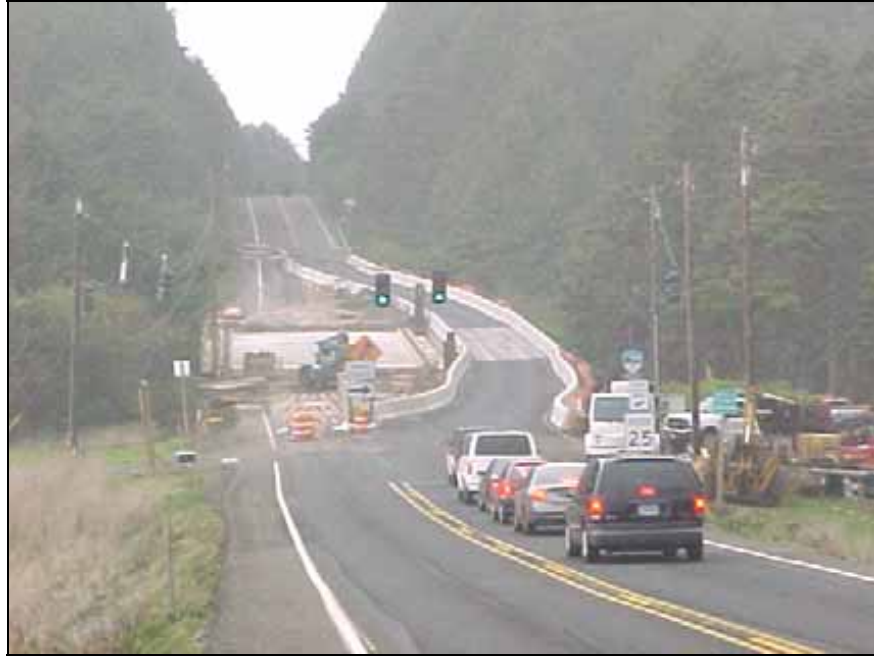
Figure 3.7: Approaching lane shift onto the temporary structure at the Bob Creek Bridge
