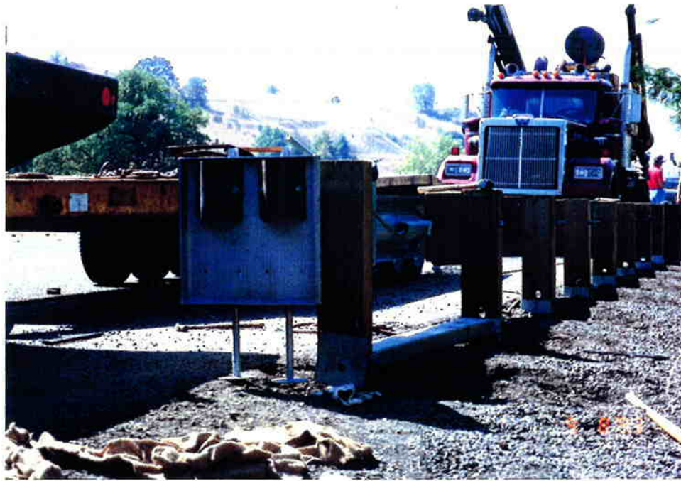
Figure A.2: ET-2000 Guardrail Extruder Head, Offset Strut, and Cable Assembly Installation.
