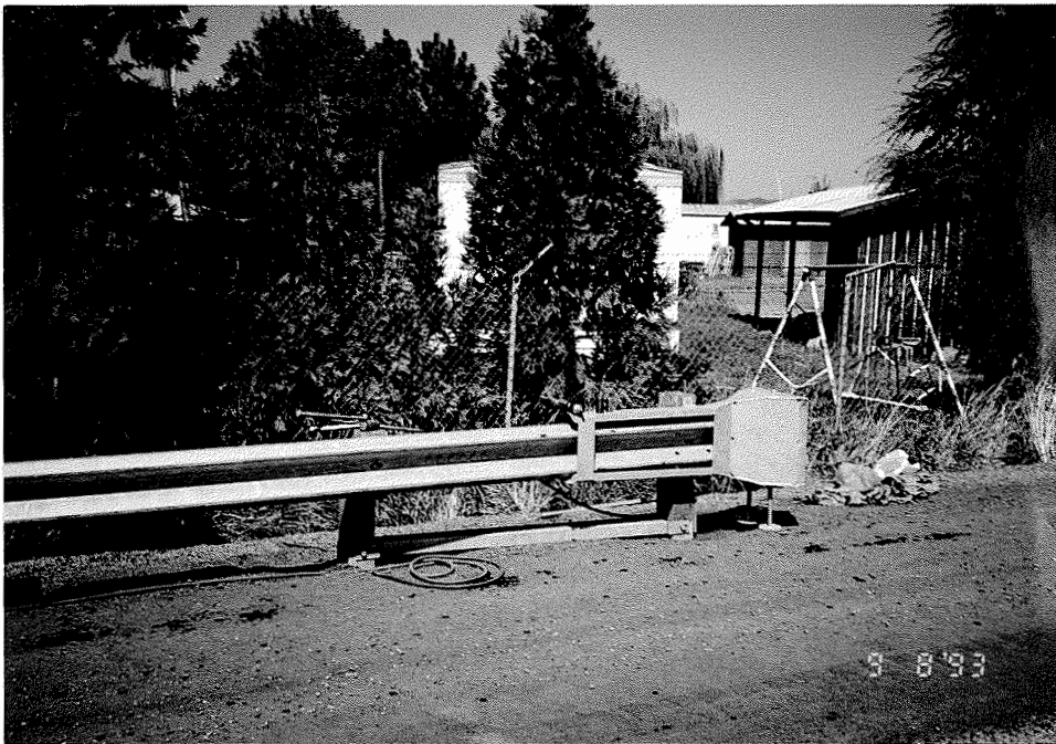
Figure 2.4: Note how close the GET is to the house in the background.
