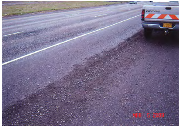
Figure 3.2: Raveling on I-205.
