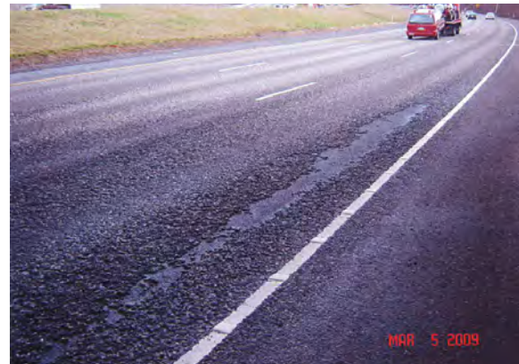
Figure 3.3: Pronounced raveling on I-205.
