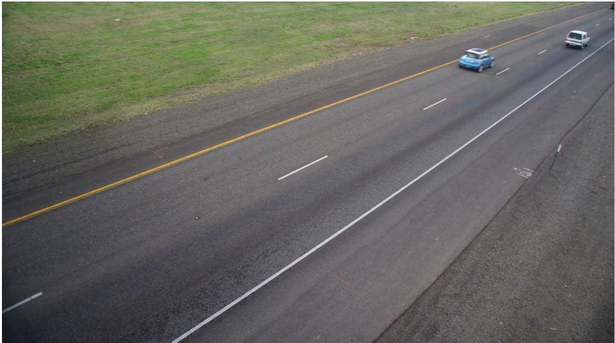
Surface was paved in 2007, picture taken in 2010. Note wear in the wheelpaths of outside lane.
