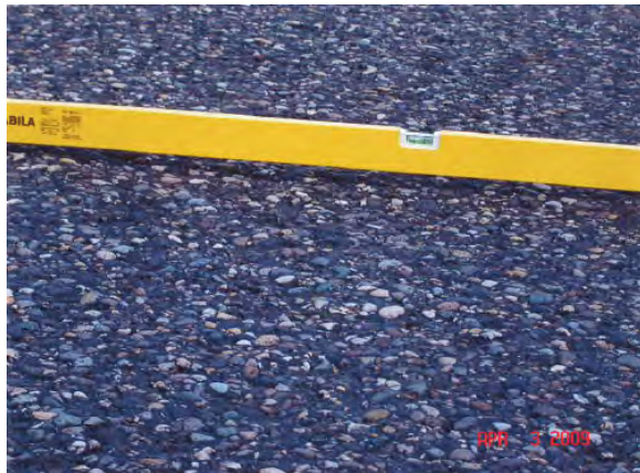
Figure 3.4: 1 ¼-inch studded tire wear on I-5 MP 304.33 NB “B” lane.
