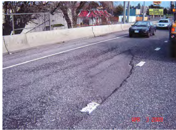
Figure 3.5: Delamination on I-5 MP 307.00.
