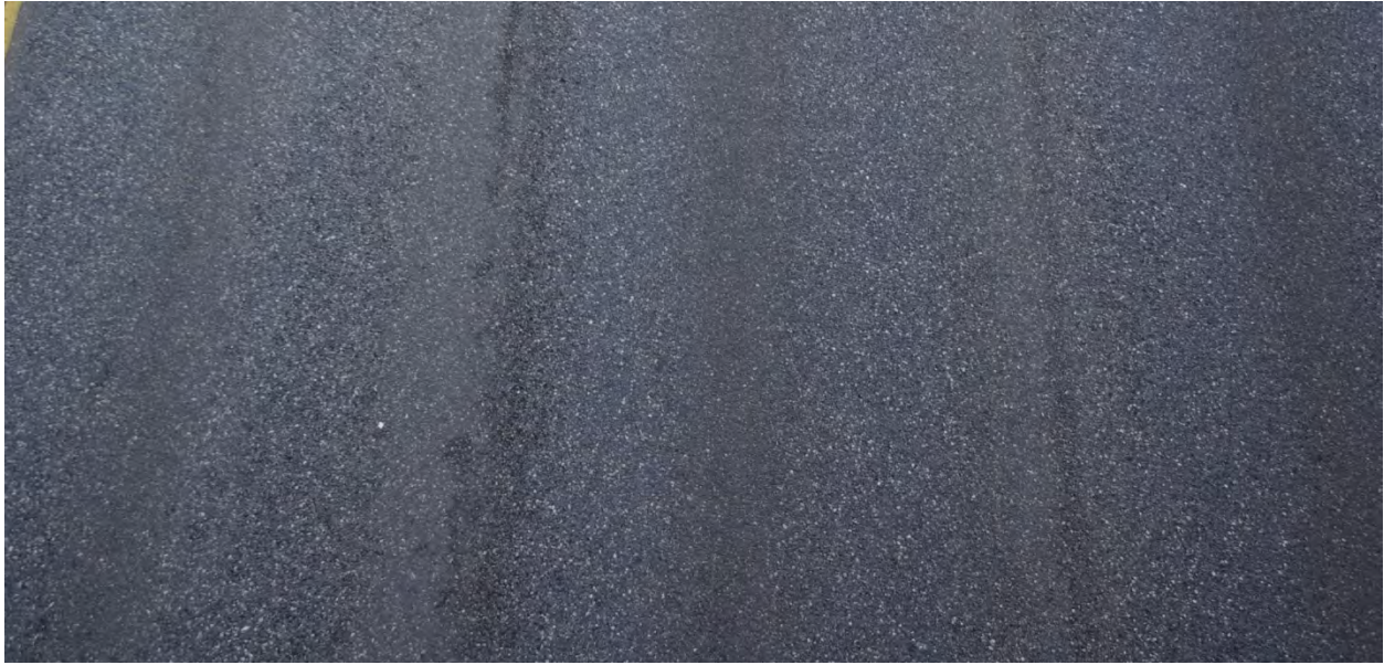
Figure 3.7 Close-up of \frac{3}{4} -inch HMA surface in Figure 2.53.
