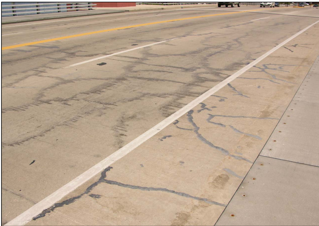
Figure 6. Cracking of exodermic bridge deck, east leaf (June 2010).
