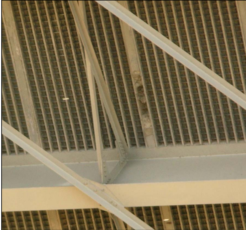
Figure 7. Void in concrete on underside of west leaf exodermic bridge deck (June 2010).
