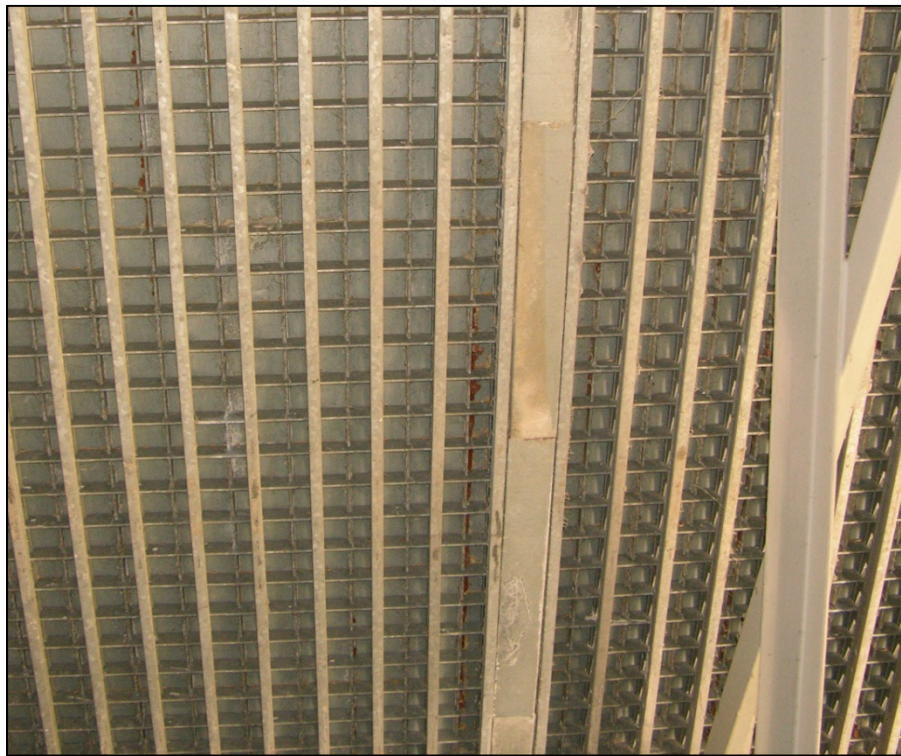
Figure 8. Corrosion and leached material on underside of west leaf exodermic bridge deck (June 2010).
