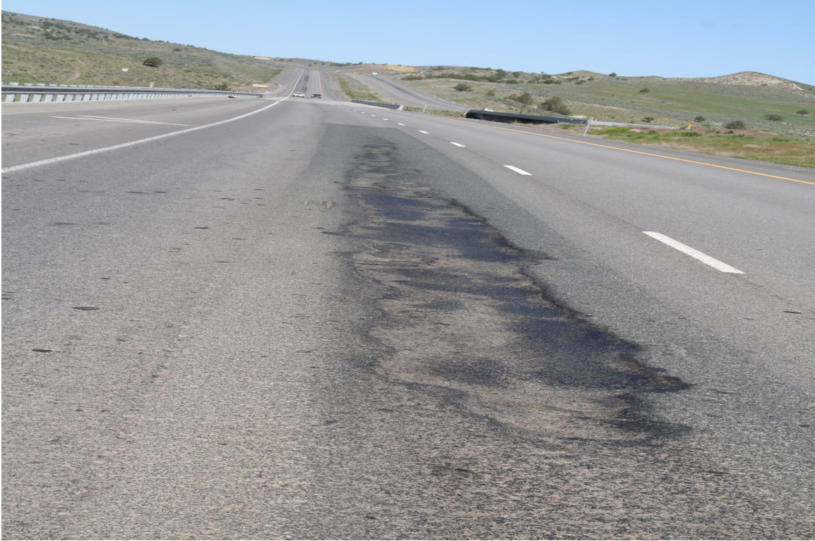
Figure D-1.4: Patch with Severe Distress Visible On the Outside Lane of the Project
