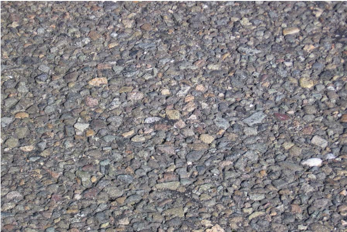
Figure D-1.26: Closer Look at the Pavement Section at MP 111
