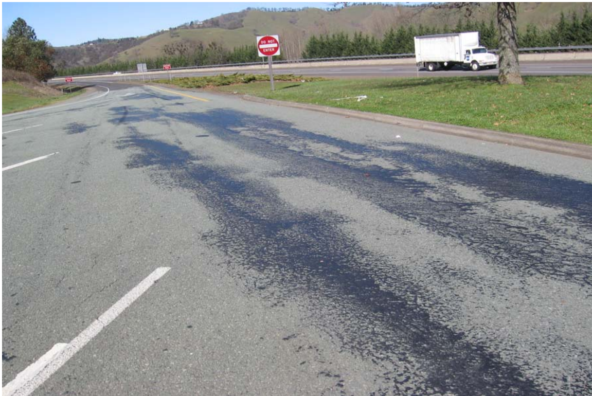
Figure D-1.22: Bleeding Observed on the Pavements near Rest Area at MP 111
