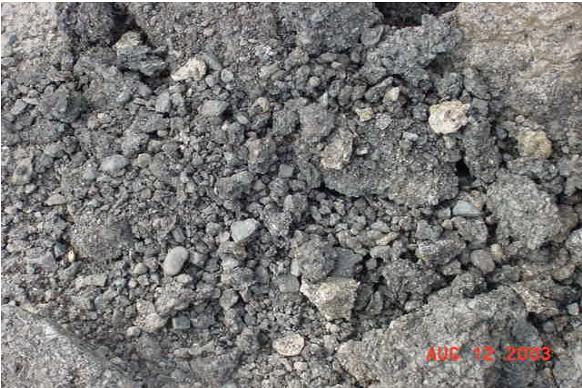
Figure C-1.3: Aggregates Removed From the Trench Showed Signs of Stripping
