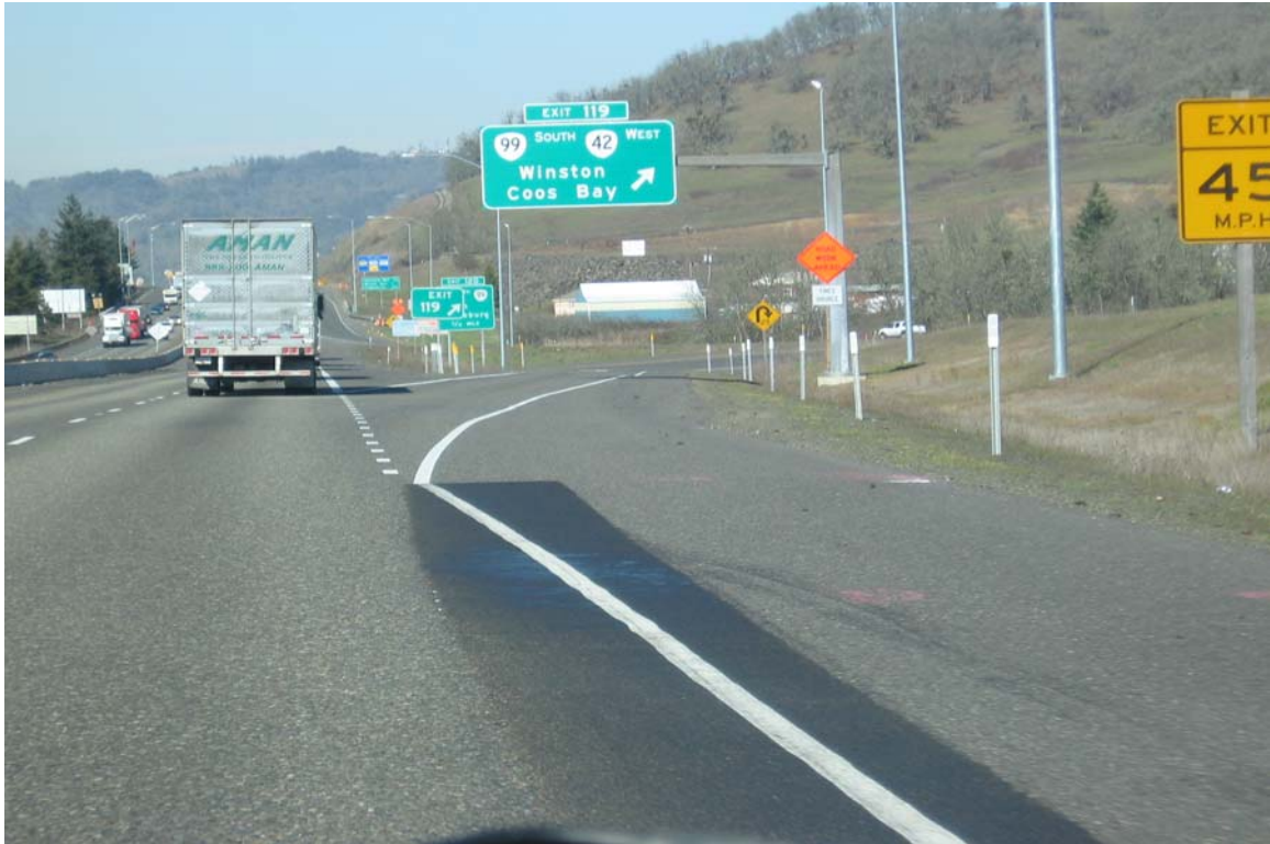
Figure D-1.14: Patch on the Outside Lane
