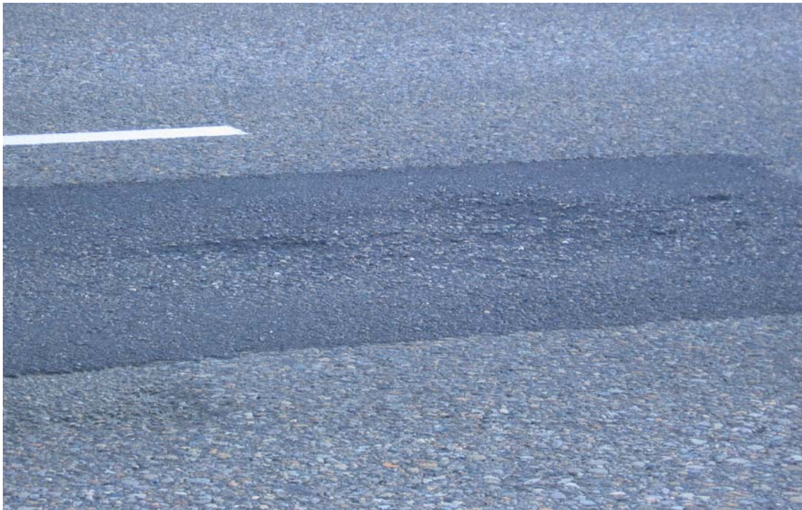
Figure D-1.12: Typical Patch Found Along This Project
