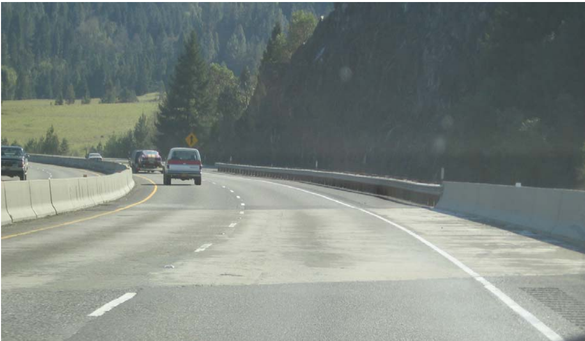
Figure D-1.21: Rock Cut Was Observed On Certain Locations of the Section
