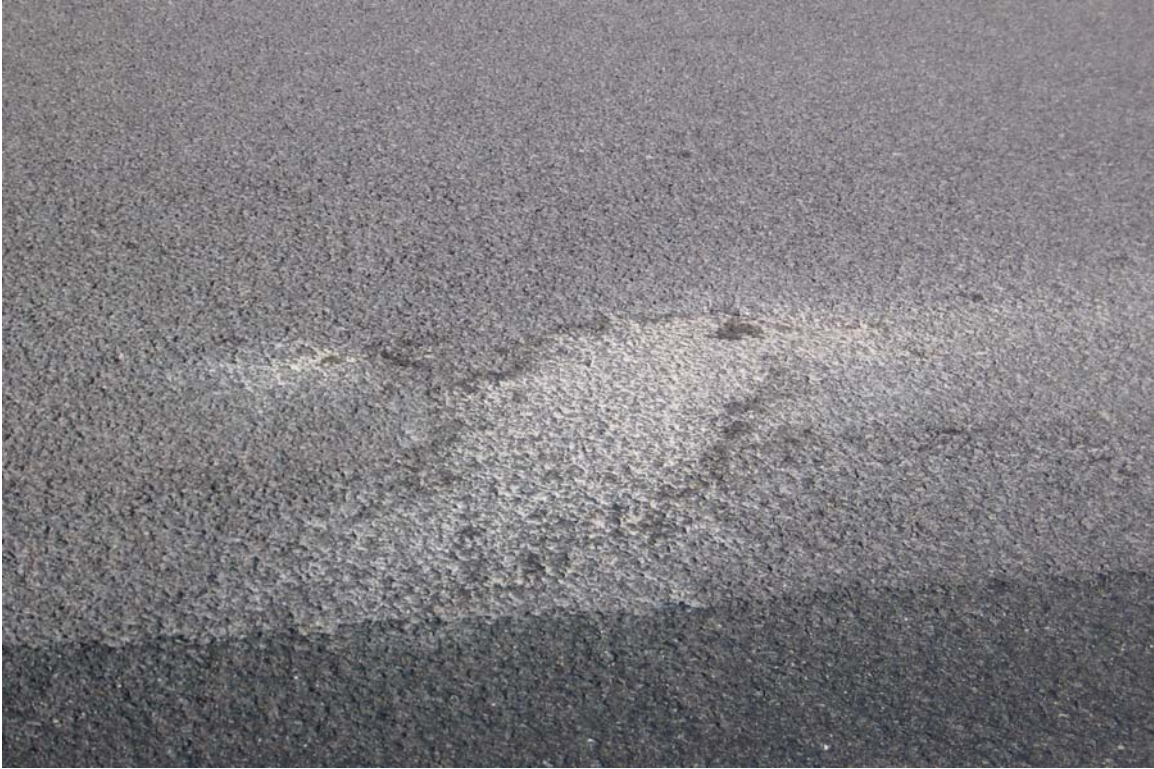
Figure D-1.5: Silt Deposits on the Pavement Surface Close To a Patch
