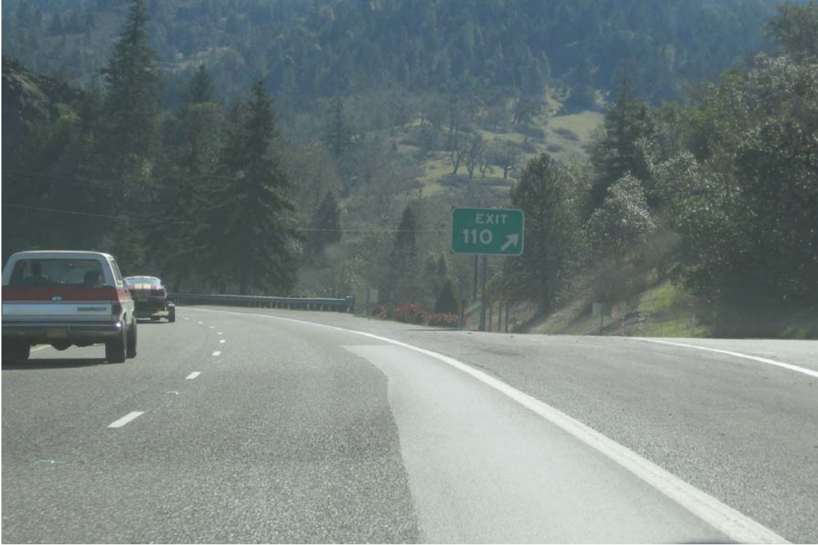
Figure D-1.20: Patch along the Outside Lane Wheel Path at MP 110
