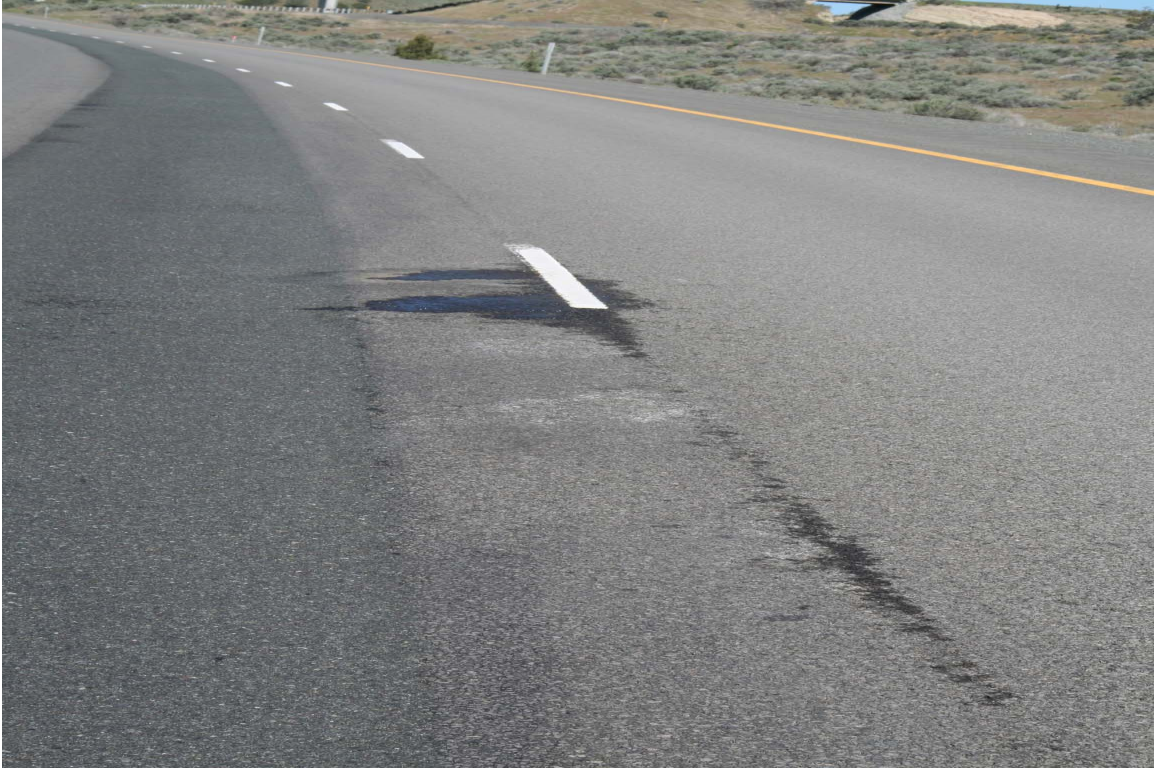
Figure D-1.2: Example of Water along the Construction Joints Close To a Long Patch
