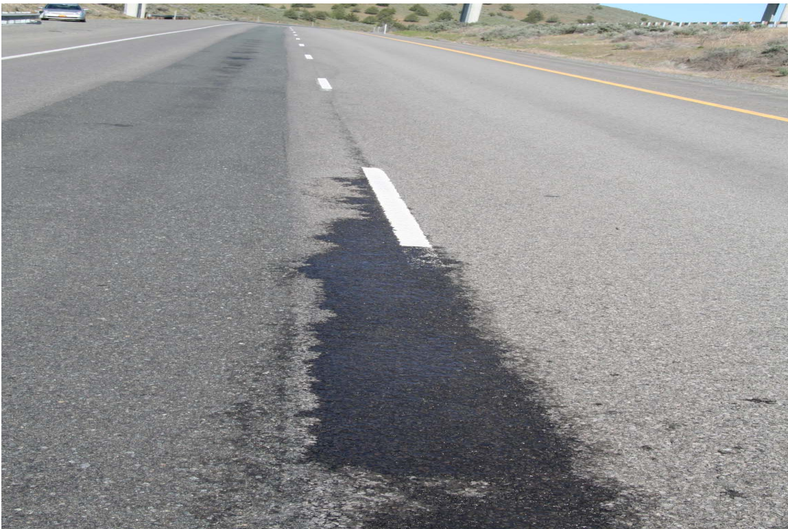
Figure D-1.1: Water Coming Out Of the Construction Joints
