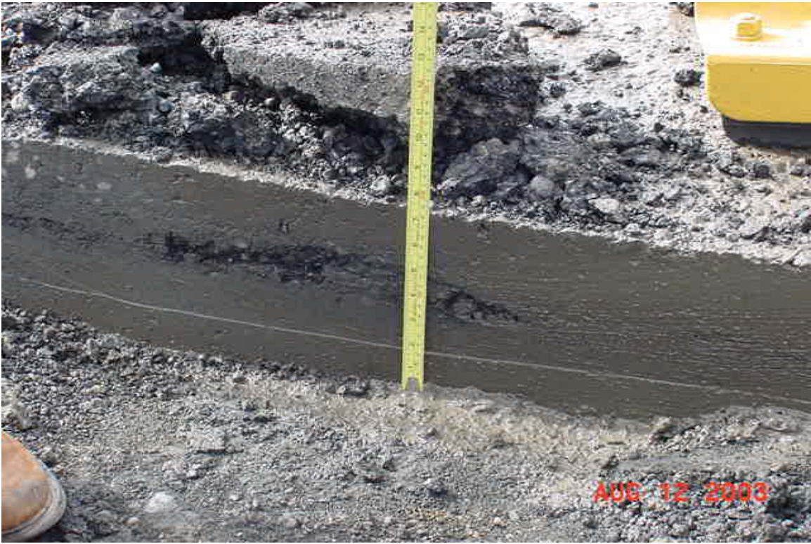
Figure C-1.4: Sides of Trench Showing Evidence of Stripping
