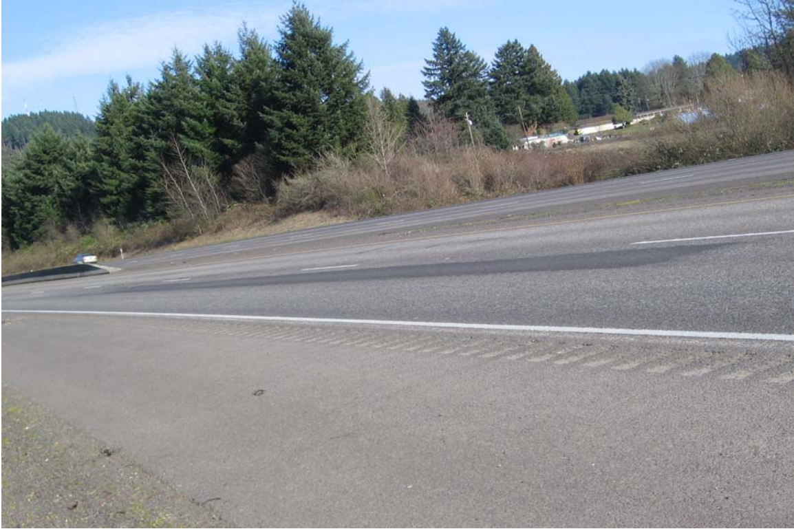
Figure D-1.6: Patch Visible On the Outside Lane inside Wheel Path
