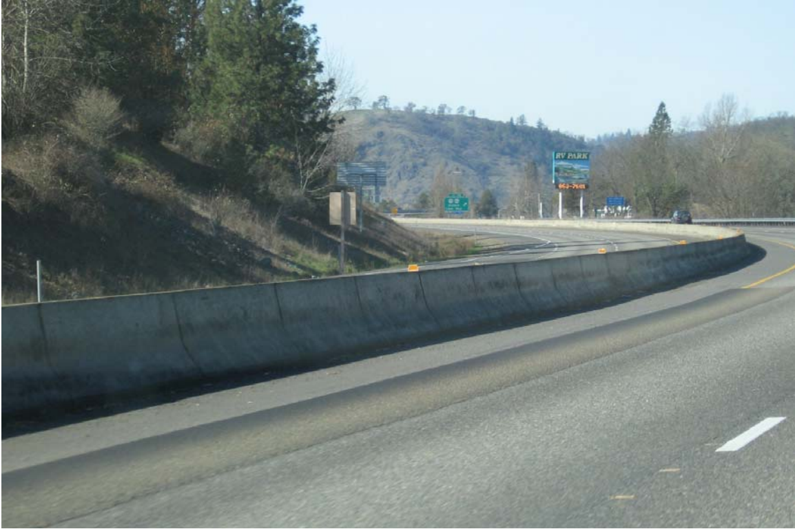
Figure D-1.28: Another Example of a Patch Found On the Inside Lane
