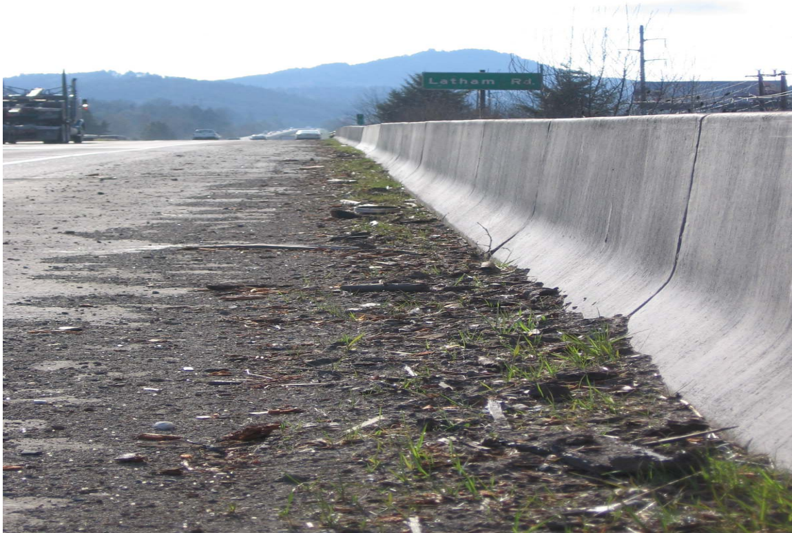
Figure D-1.9: Condition on the Sides of a Bridge Where Vegetation Has Grown
