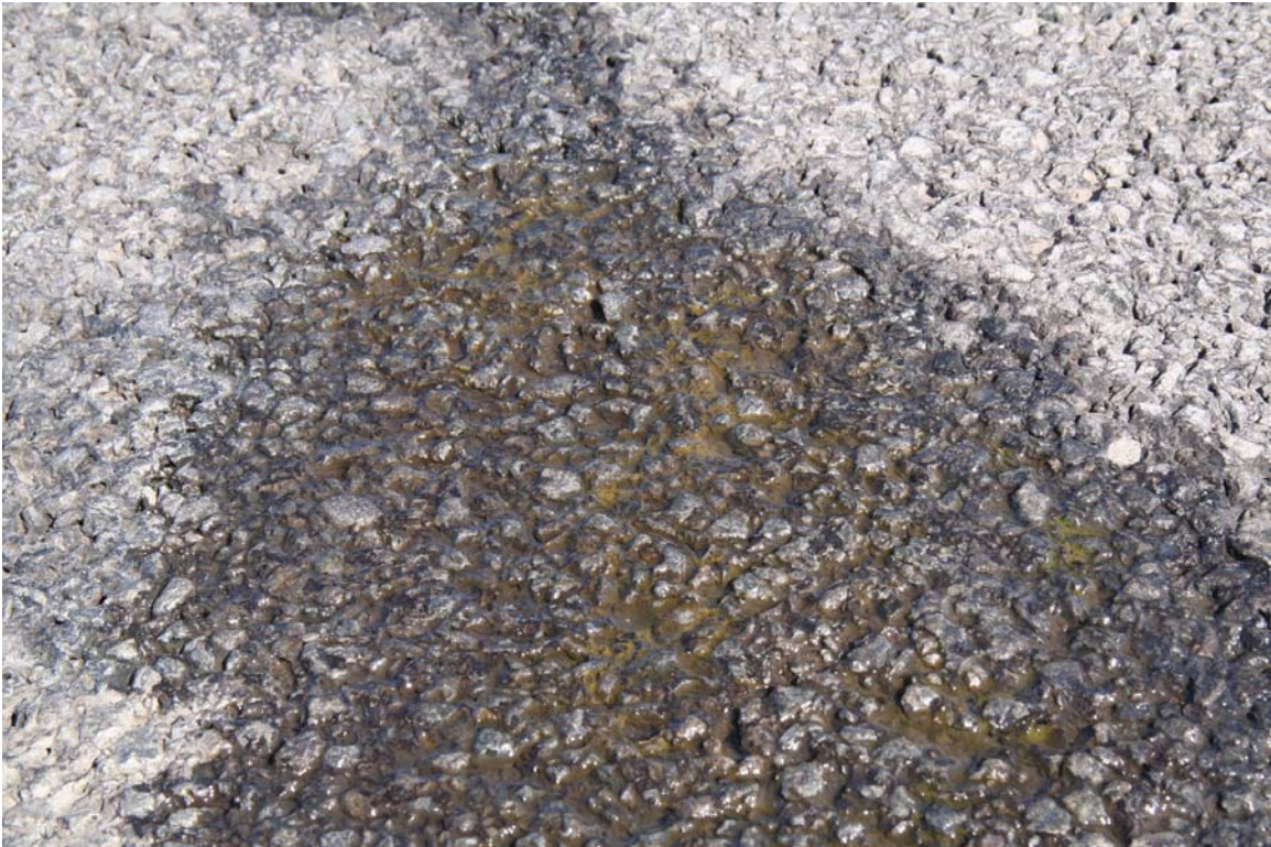
Figure D-1.3: Colored Water Coming Out Of the Pavement Joints
