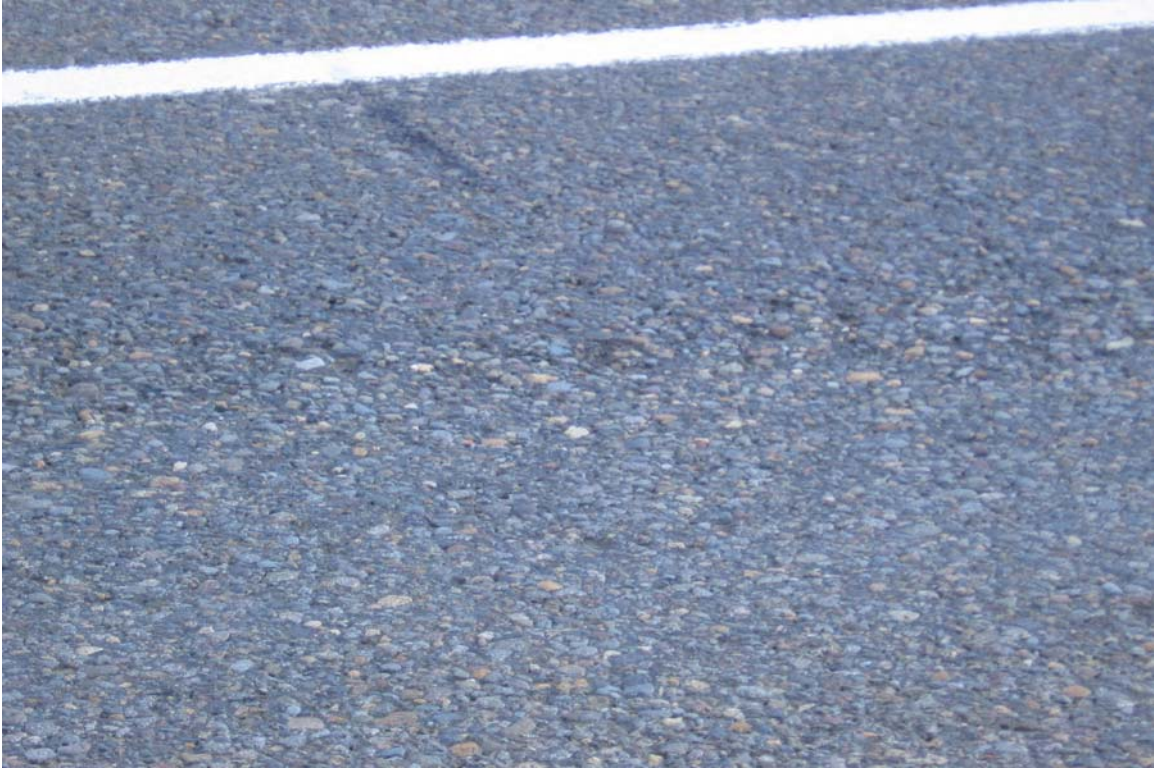
Figure D-1.13: Part of the Pitted and Raveled Pavement Section
