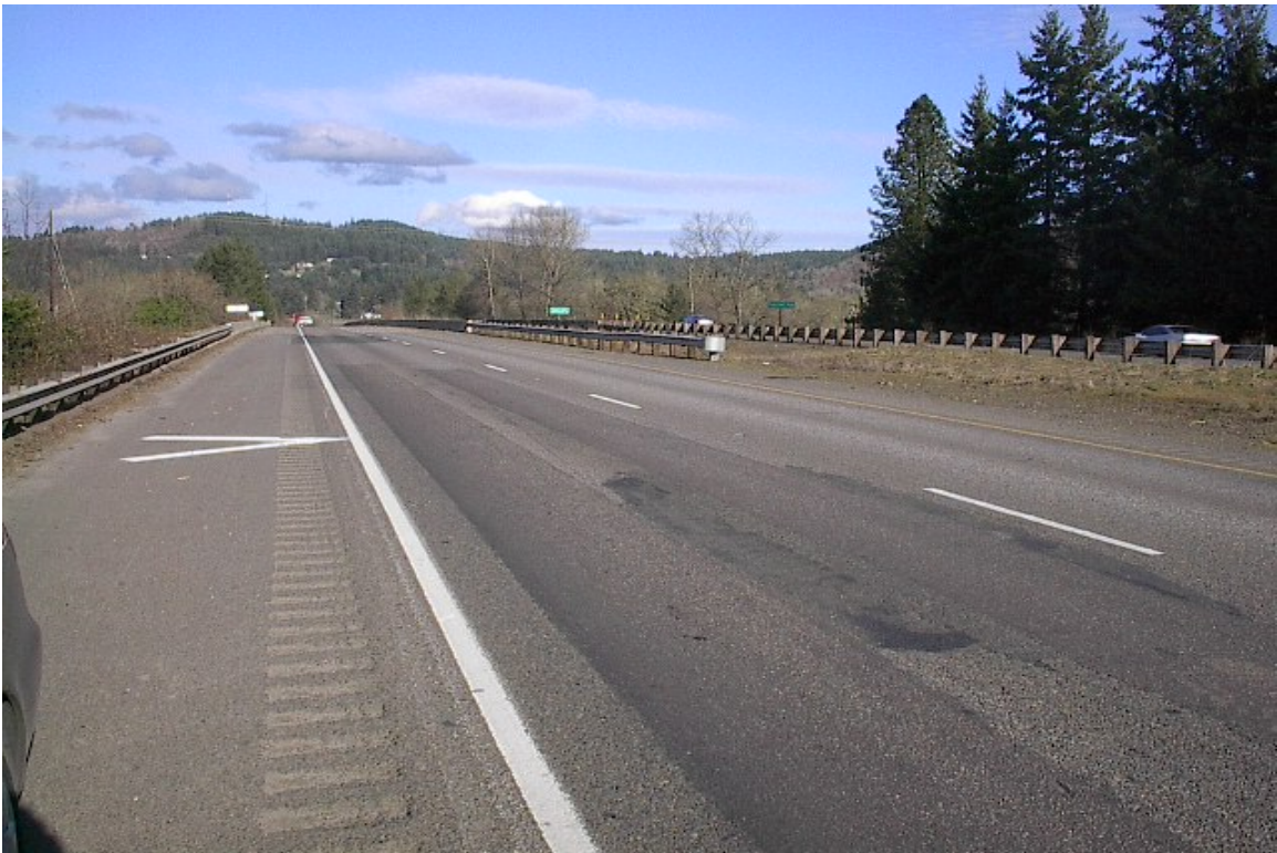
Figure D-1.7: Example of Two Patches in the Wheel Paths of the Outside Lane
