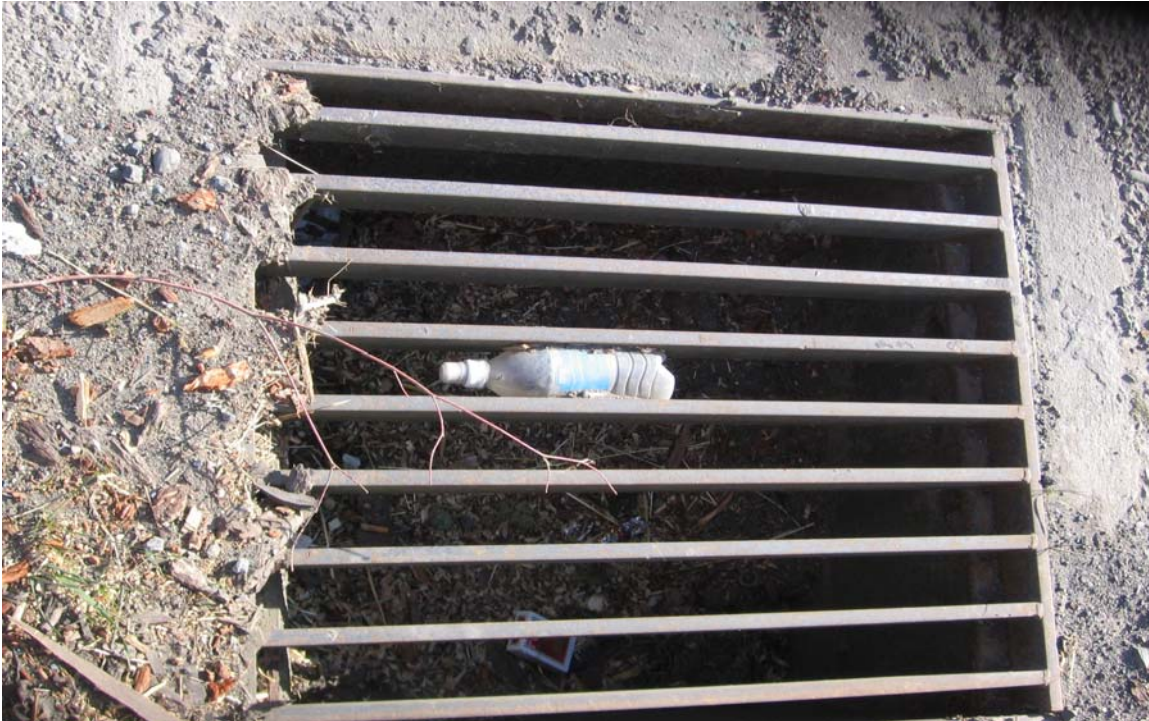
Figure D-1.8: A Partially Clogged Drain That Was Found Close To the Patches in the Previous Pictures (Figures D-1.6 and D-1.7)
