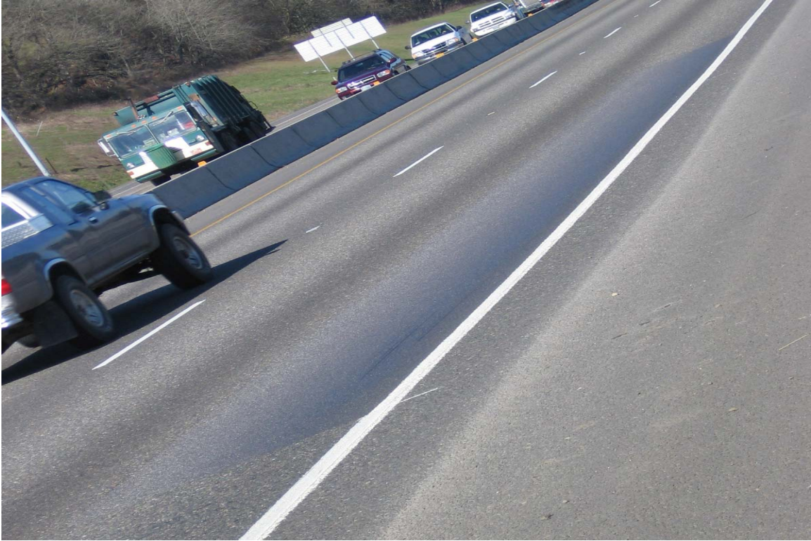
Figure D-1.16: Close-up of the patch on the outside lane wheel path
