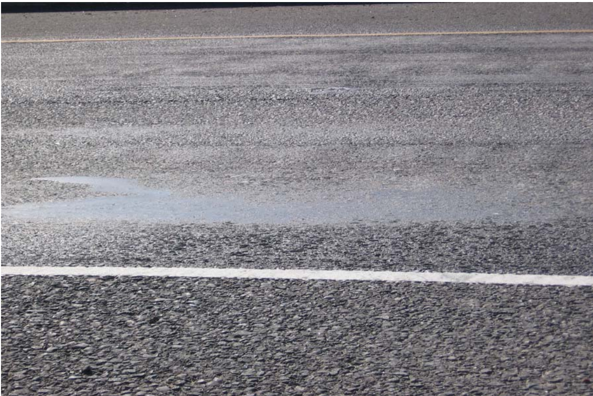
Figure D-1.29: Combinations of Rutting, Patches, and Bleeding
