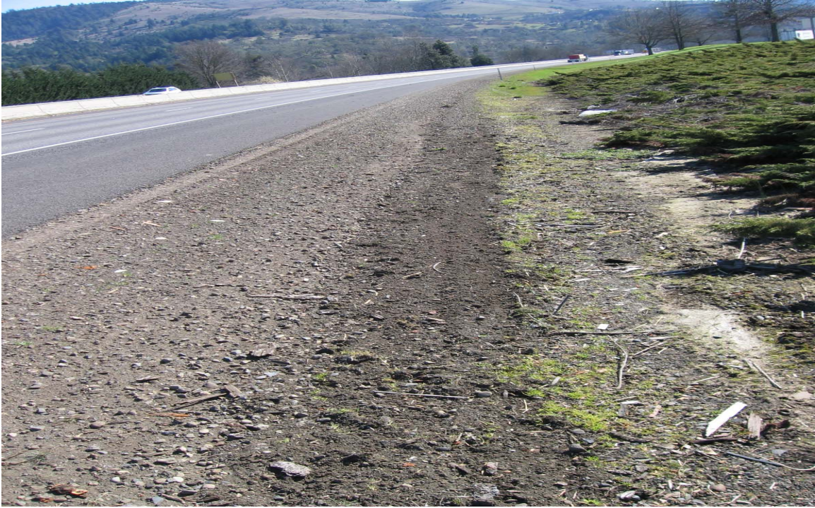
Figure D-1.25: Vegetation Scraped Along the Pavement Section (Scraped Once A Year)
