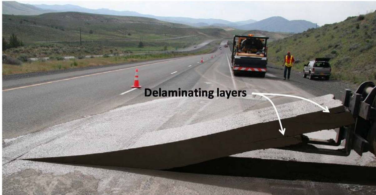
Figure 3.11: Pavement Layers Delaminating During Removal.
