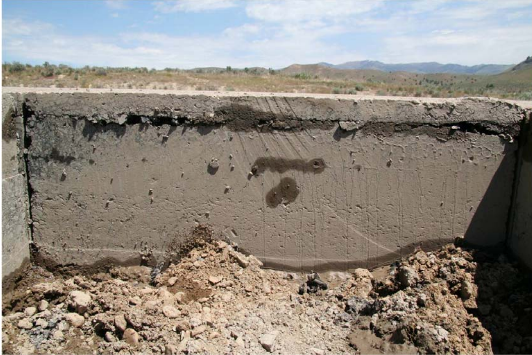
Figure 3.13: Wearing Course Delaminated from the HMA Course at the End of the Slab.
