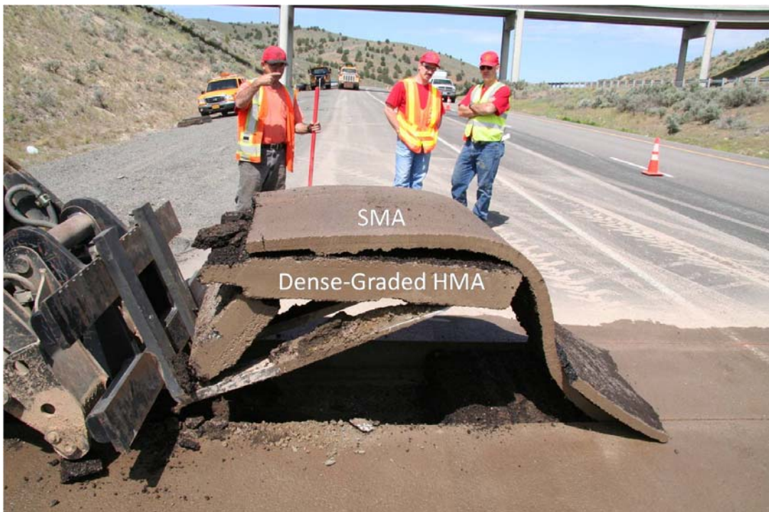
Figure 3.4: SMA Wearing Course Delaminating from Underlying HMA Course.
