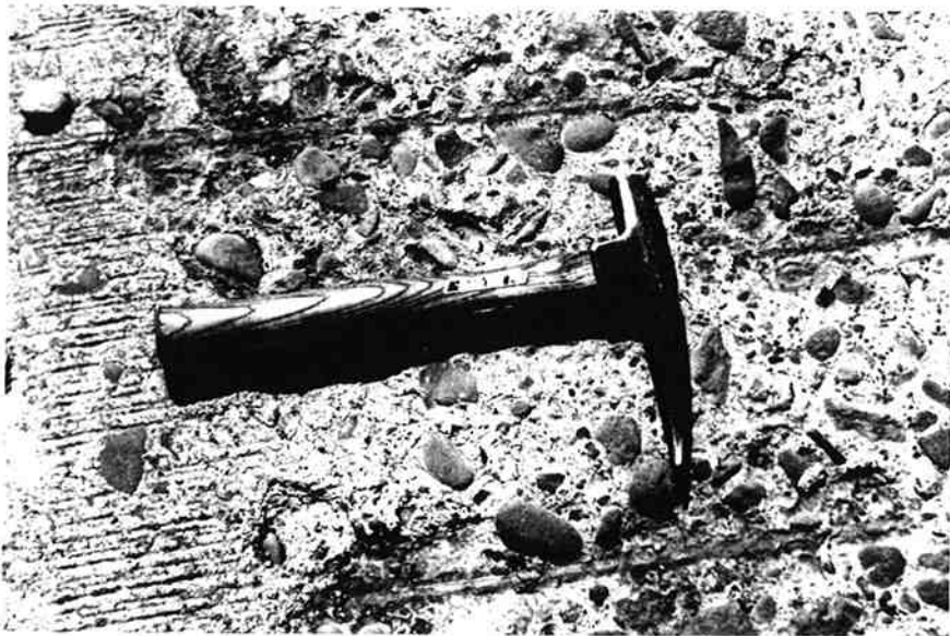
Figure 2. Typical bridge deck spalling.
