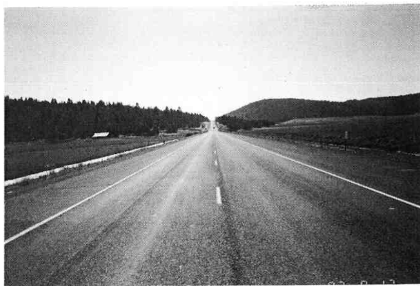
Figure B.4 - Typical pavement surface condition of the Lakeshore Dr. - Greensprings Jct, (Lake of the Woods) project. Photo was taken at MP 63.36 looking ahead on line on September 17, 1987. Surface is chip sealed.
