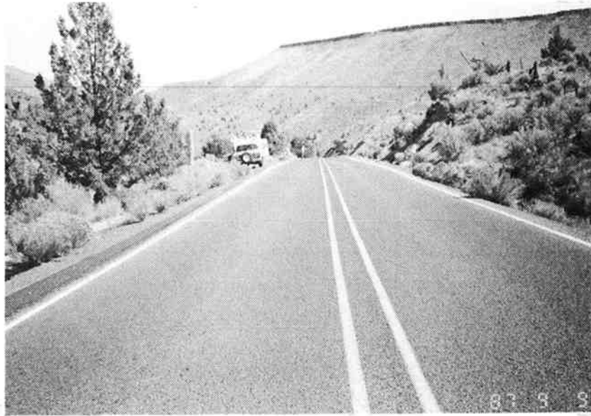
Figure B.3 - Typical pavement surface condition of the MP 89.6 - Jct. OR 19 (Ochoco Hwy) project. Photo was taken at MP 96.4 looking ahead on line on September 9, 1987. Surface is chip sealed.
