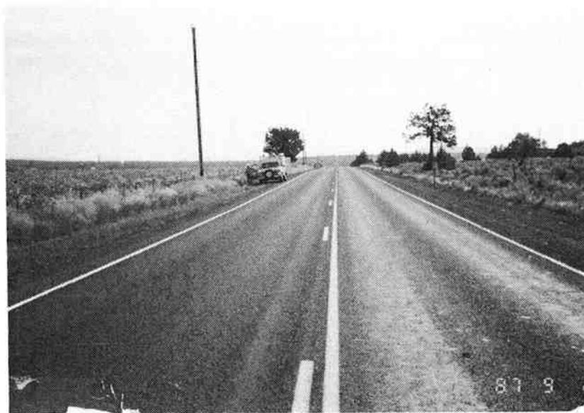
Figure B.2 - Typical pavement surface condition of the Powell Butte - Prineville (Ochoco Hwy.) project. Photo was taken at MP 11.0 looking ahead on line on September 2, 1987. Surface is chip sealed.
