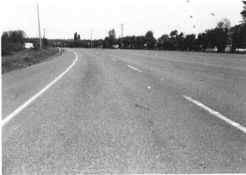
Fig. B.4. Good--pavement structure is stable. May have minor surface erosion or cracking.
