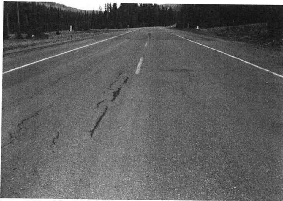
Fig. B.3. Fair--generally stable structure with minor areas of structural distress evident.
