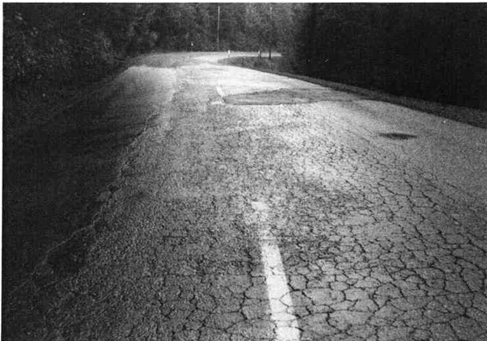
Fig. B.1. Very Poor--Extensive pavement distress and possible base failure
