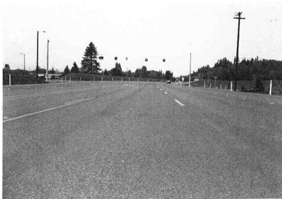
Fig. B.5. Very good--pavement structure is stable with no cracking, patching, or deformation.
