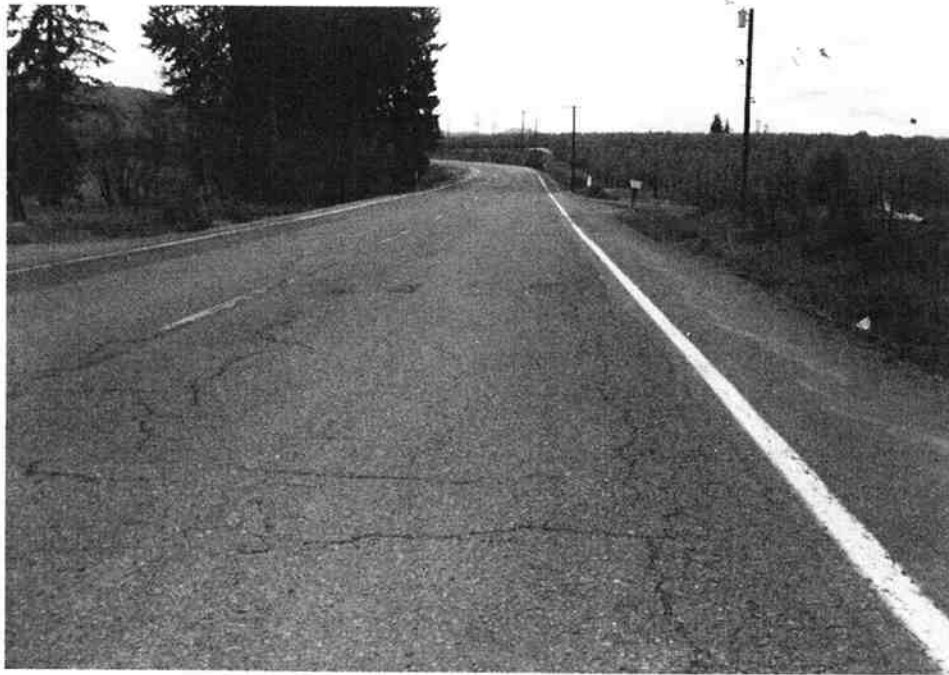
Fig. B.2. Poor--marked evidence of structural deficiencies.
