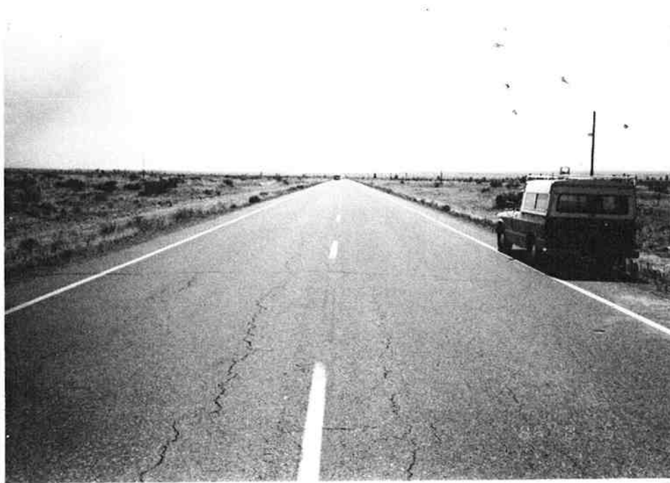
a) Warm Springs Highway, Unit A (Rated "Poor")
