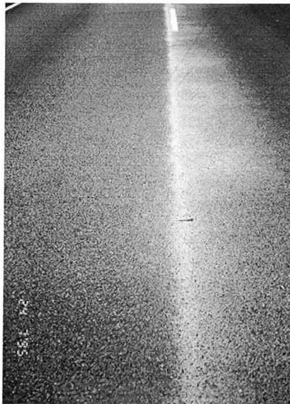
b) Staining at Joint, MP 134.5
