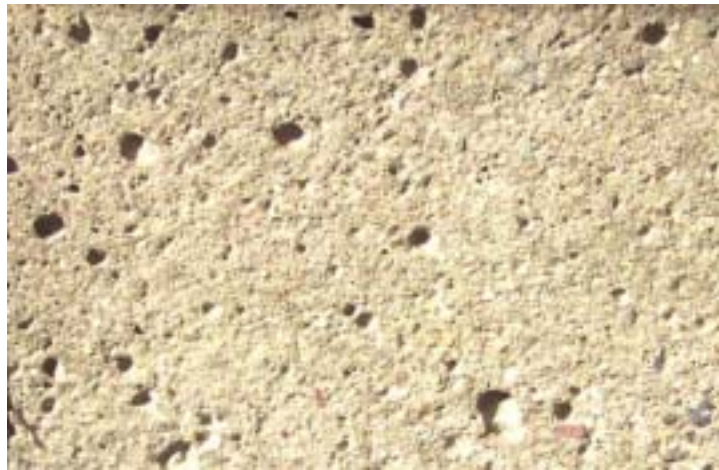
Figure 3-13: Concrete Surface Irregularities
