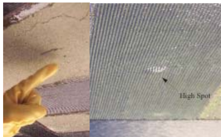
Figure 3-18: Air Entrapment over High Spots
