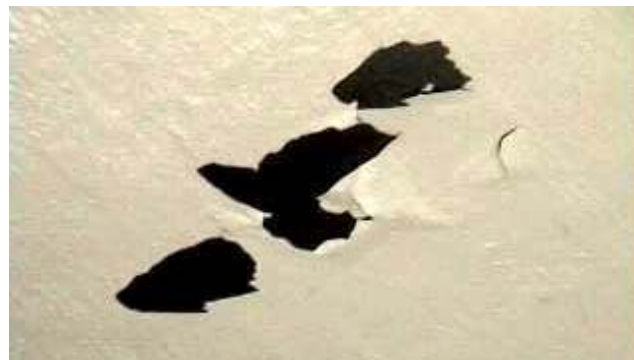
Figure 3-34: Damaged Surface Coating
