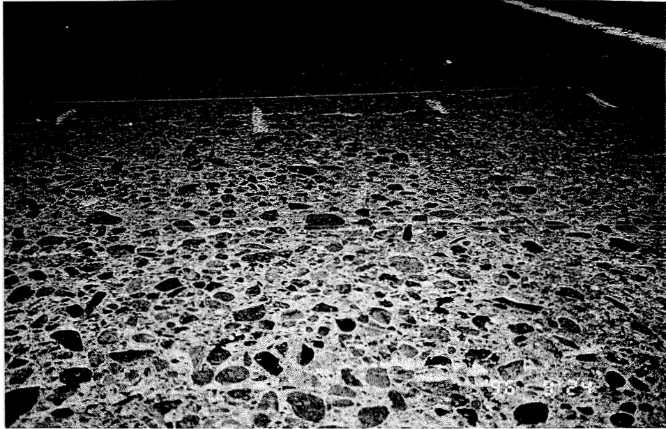
Figure 2.3 Rutting in CRC Pavement.
