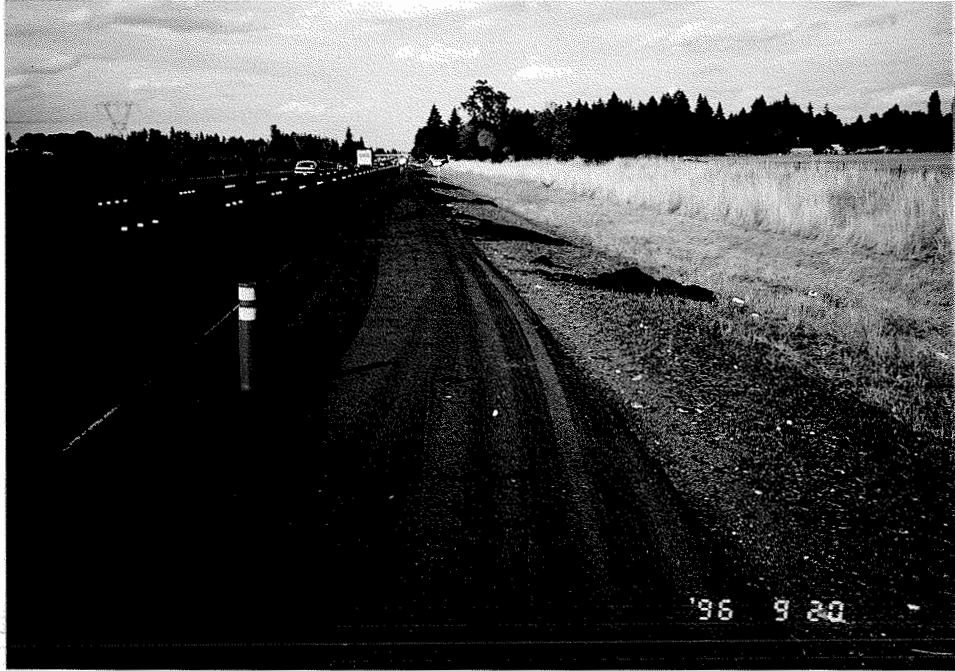
Figure 3.3 Lumpy asphalt mix was removed from the windrow and piled on shoulder.
