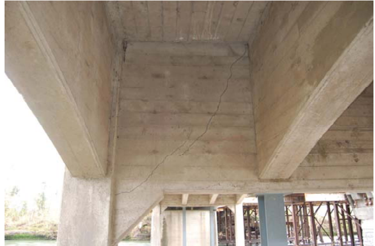
Bent cap with crack highlighted.
