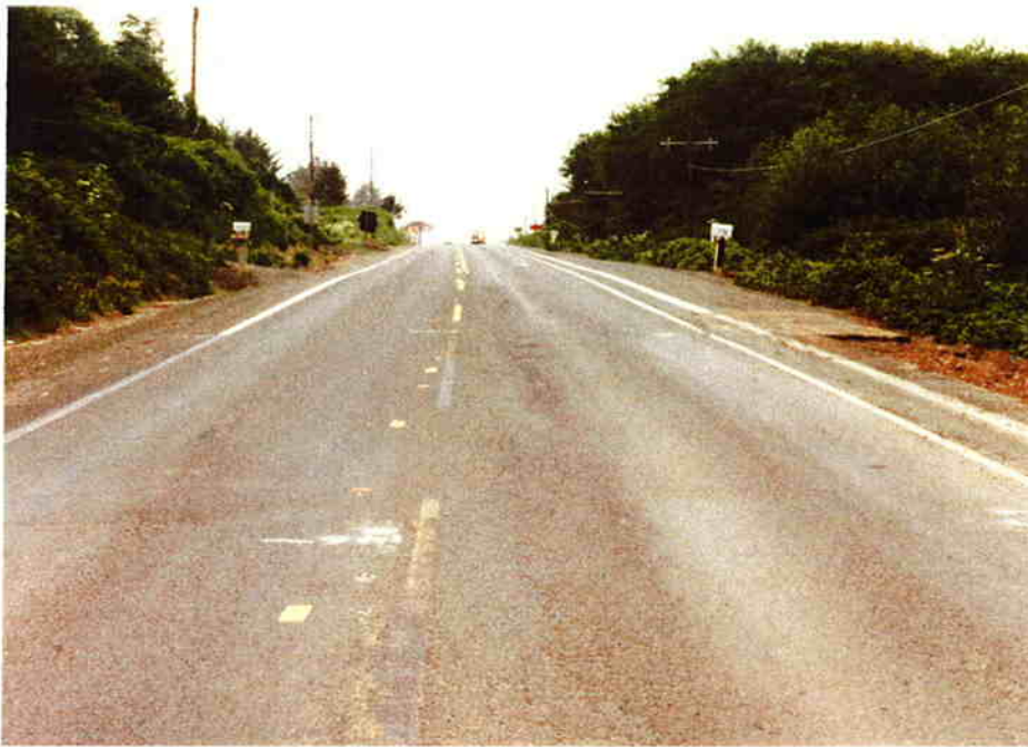
6/10/77 Southbound view from near sta. 146. Note use of reflective tape and faintness of the raised markers.
