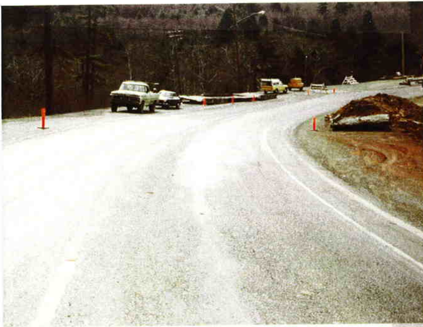
3/22/77 Looking south from sta 1869 at reflectorized buttons (overcast day). Buttons barely visible.
