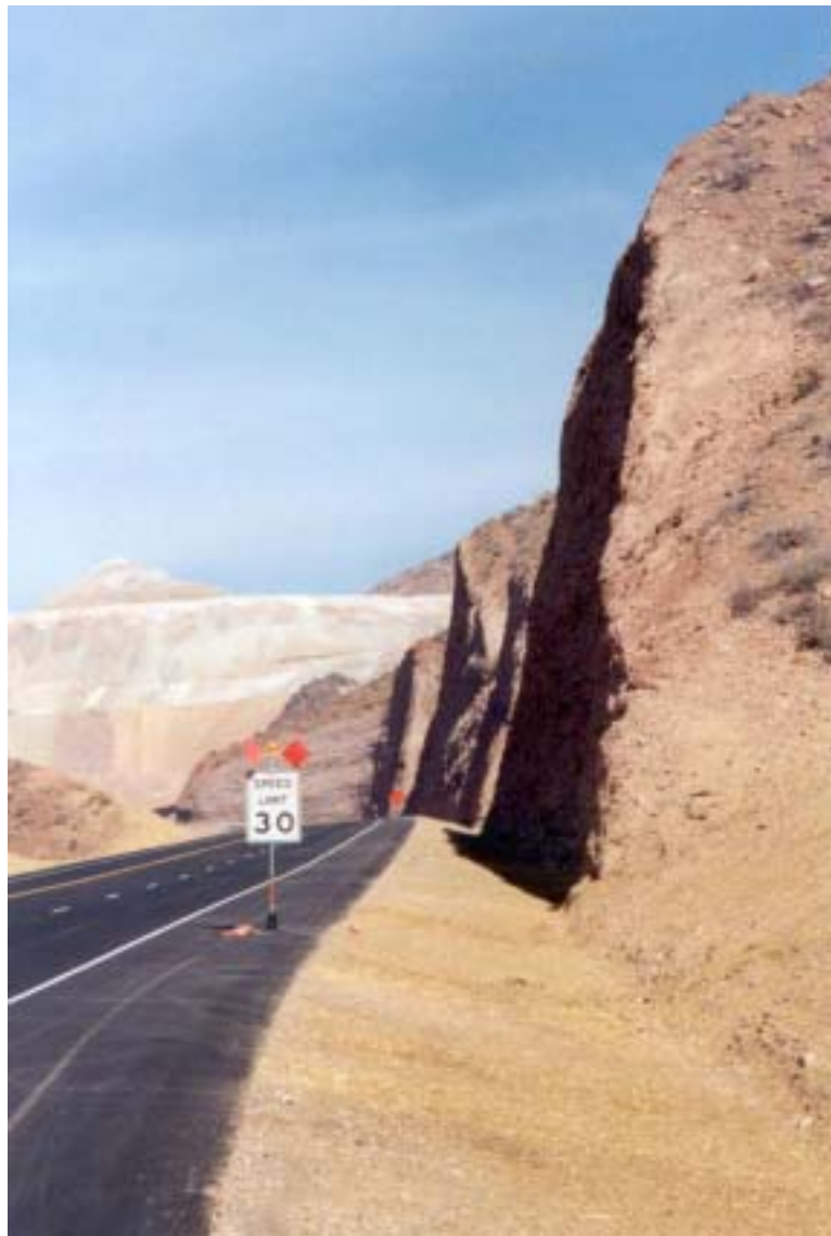
Photo 3: Arizona US 191 project. Shows the completed cut slopes and rockfall catchment ditches just prior to opening for traffic. Draped mesh not yet installed. View is Northbound.
