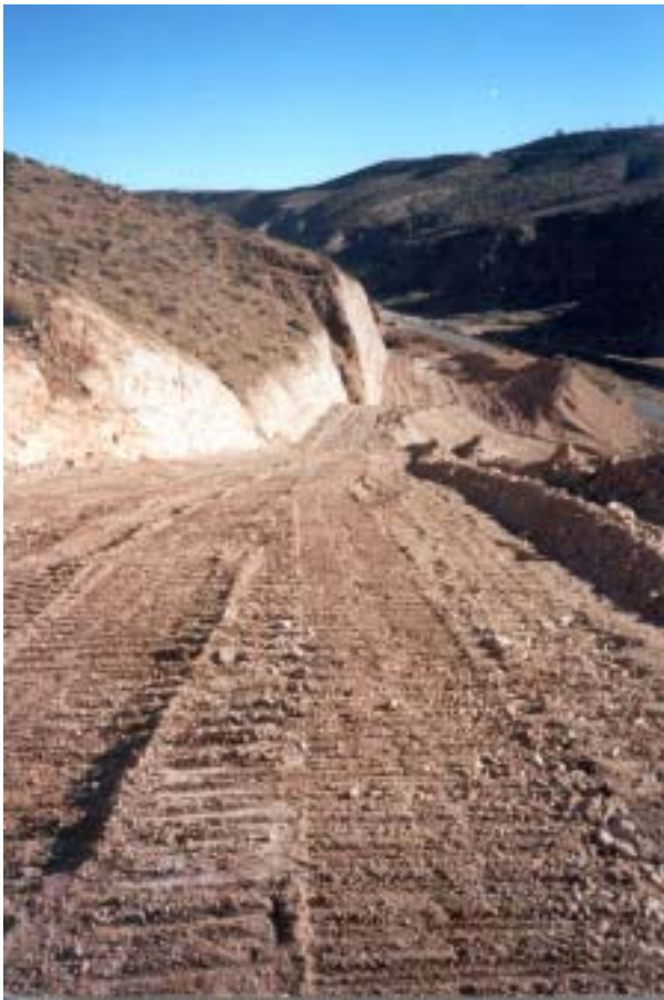
Photo 1: Arizona US 191 project. This shows the cut that the rocks were rolled from. Construction is in progress. View is Southbound.
