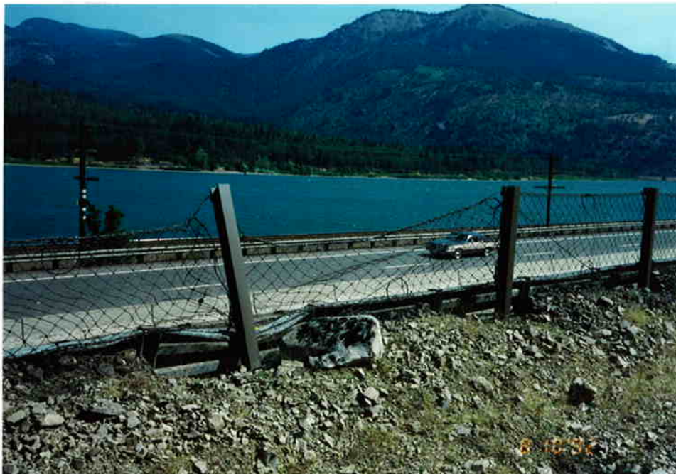
Figure 1: Brugg Cable Mesh Rockfall Fence after August 8, 1992 rockfall.
