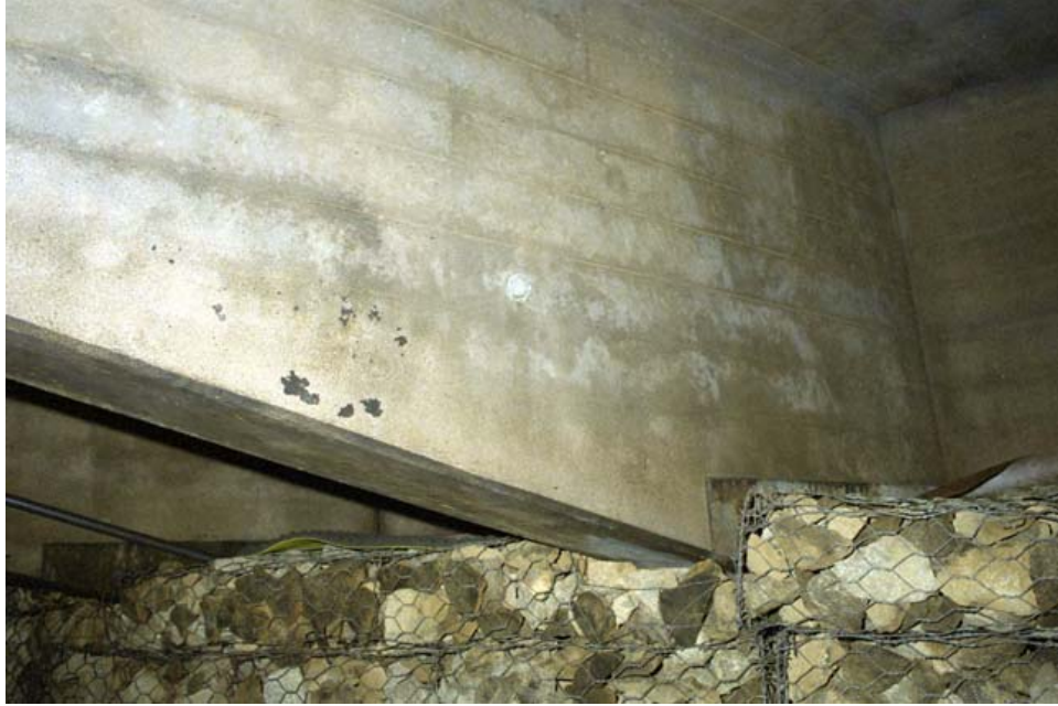
Figure 3.4: The catalyzed titanium anode CP zone 14 on the Depoe Bay Bridge. Small visible spalls on the anode occurred during thermal spraying the anode. There has been no recurrence of spalling since 1995 when the anode was applied to the bridge.
