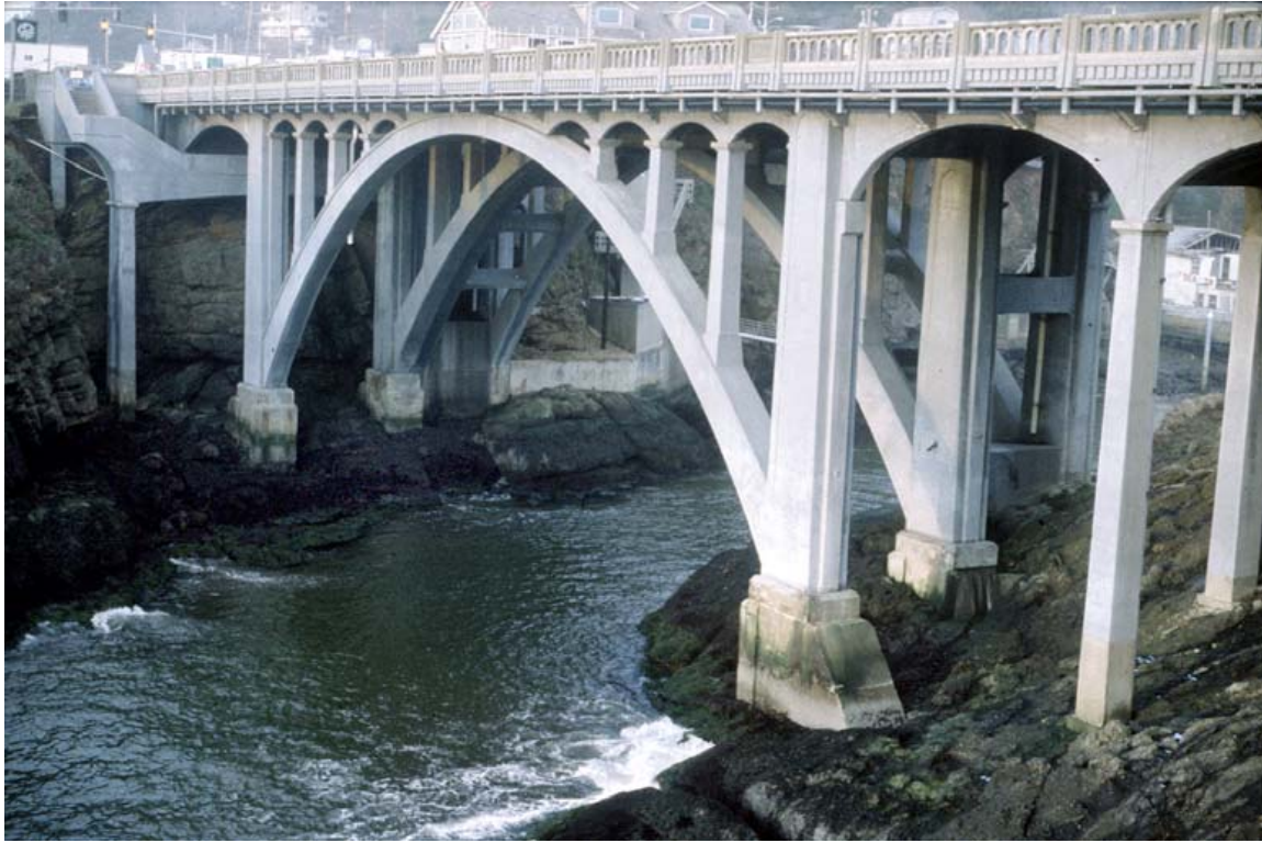
Figure 1.2: Depoe Bay Bridge with TS zinc anode ICCP zones in 1995. Approximately 21 tons of zinc was sprayed onto the bridge substructure to form the anodes.
