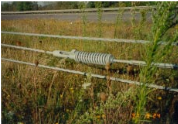
Three-cable median barrier system with spring turnbuckle
